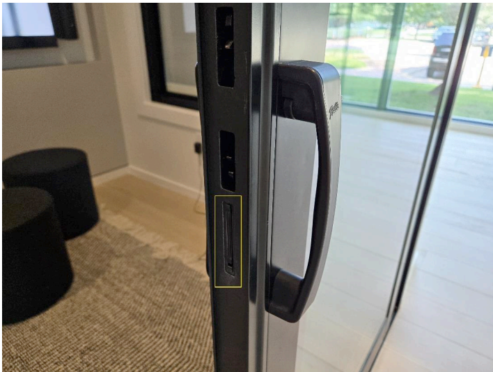
Doors' locking panel sensor location – Location of battery powered sensor
