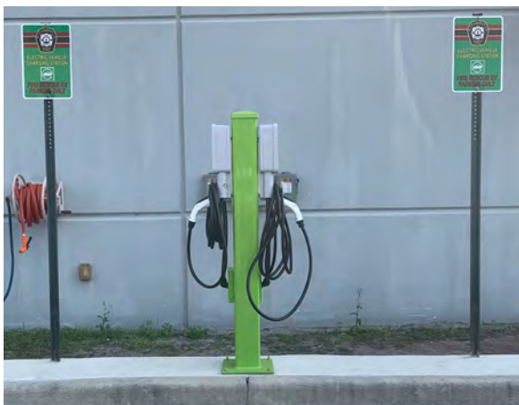
Fire Rescue provides EV charging stations.
