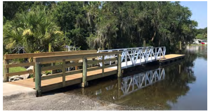
CELM department maintenance staff rebuilt the floating boat docks at the Riverview Civic Center Boat Ramp located on the Alafia River.
