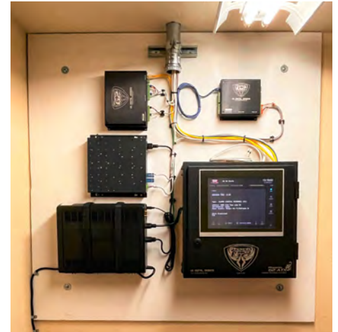
Information Technology assists Fire Rescue with the new enterprise Station Alerting infrastructure.
