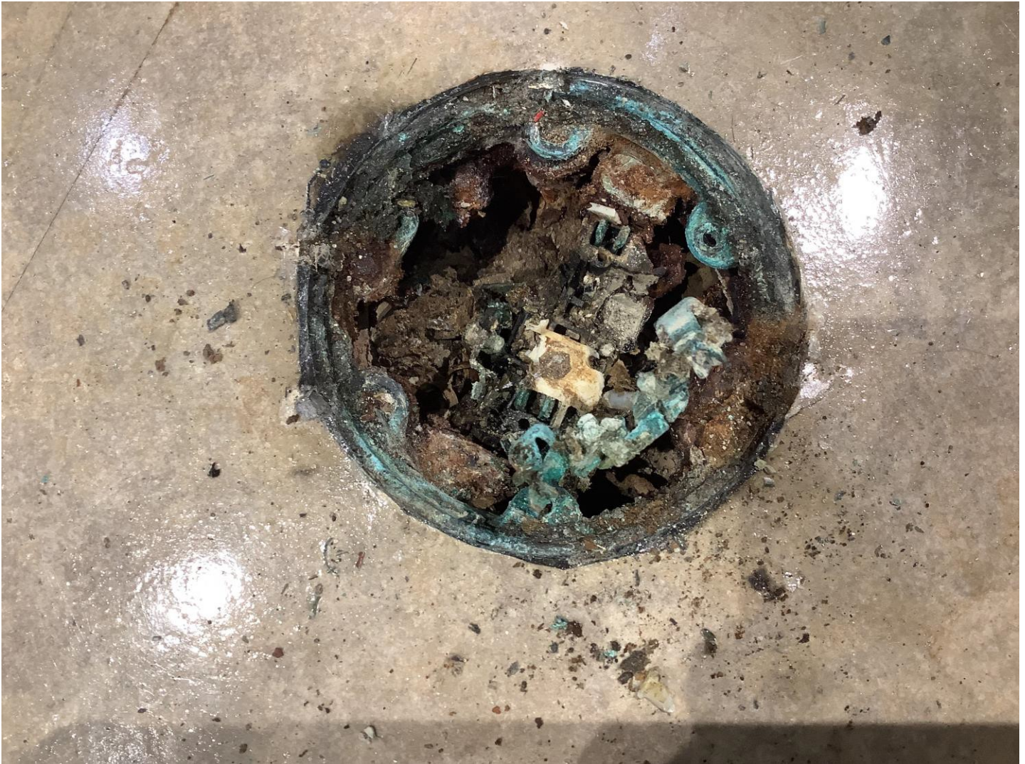
Image 4 – Removing the receptacle from the floor box, the corrosion was so severe the receptacle was fragmenting into pieces.
