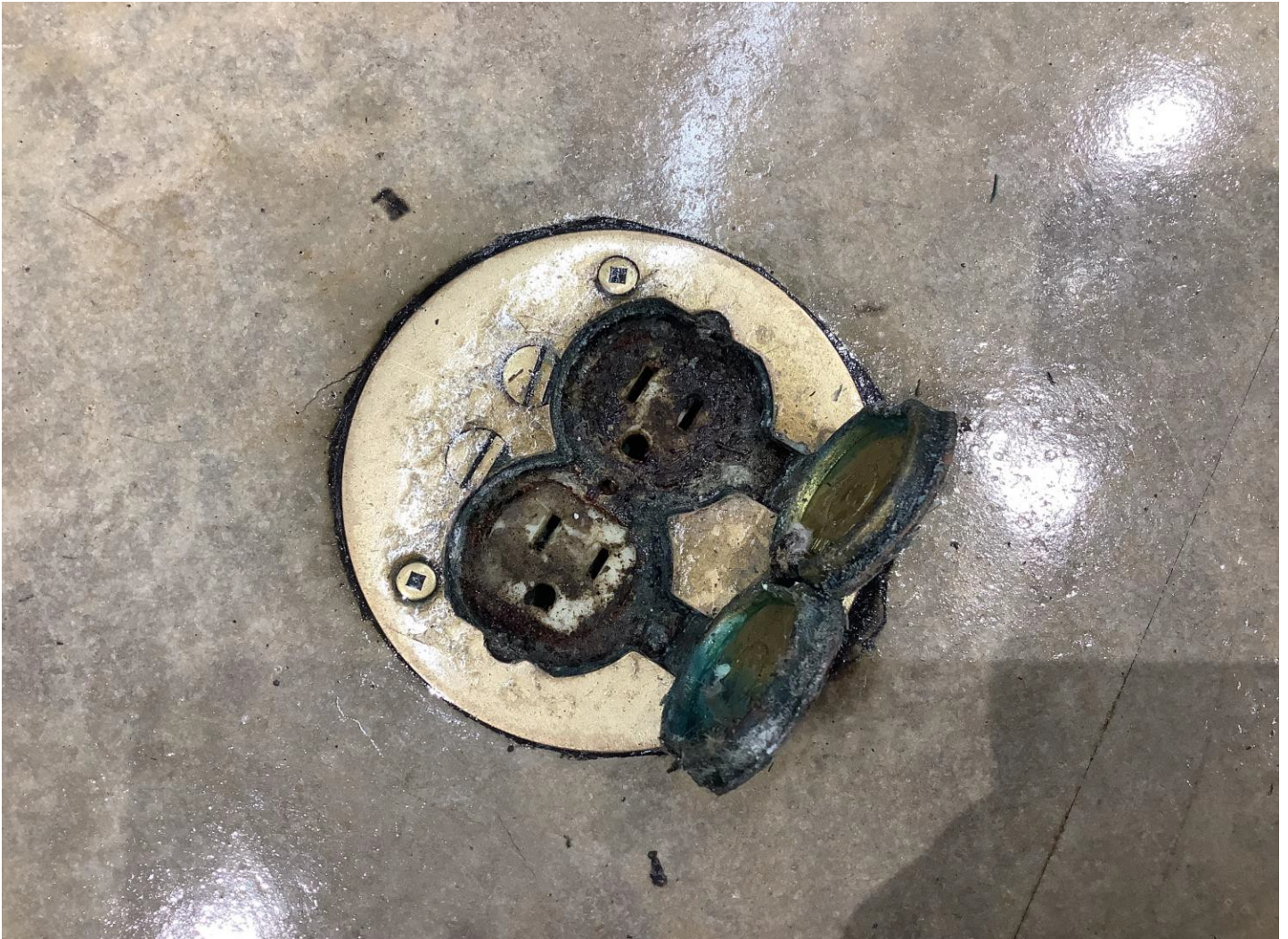
Image 2 – Images (2-5) are from a sampled floor receptacle located in the same building showing corrosion (not the one involved in the incident) sampled receptacle was energized before removal.
