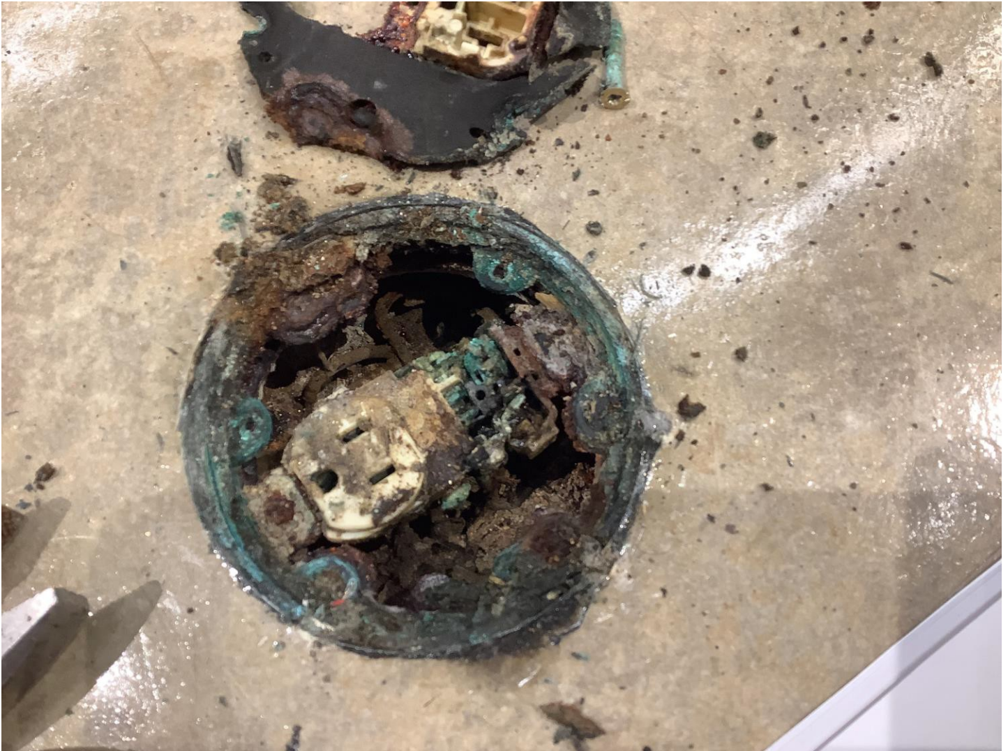
Image 3 – Floor receptacle with cover and gasket removed, when the cover was removed the receptacle corrosion was so severe the receptacle broke away exposing the corroded unprotected terminals.
