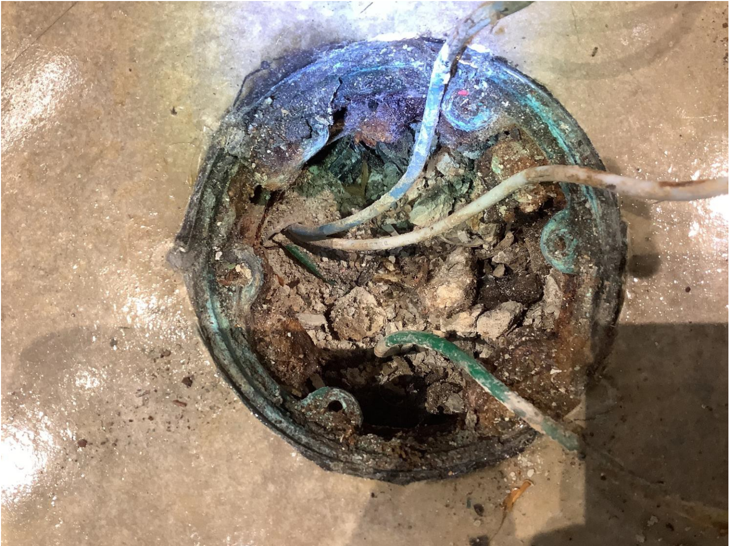
Image 5 – The amount of debris inside the floor box.
