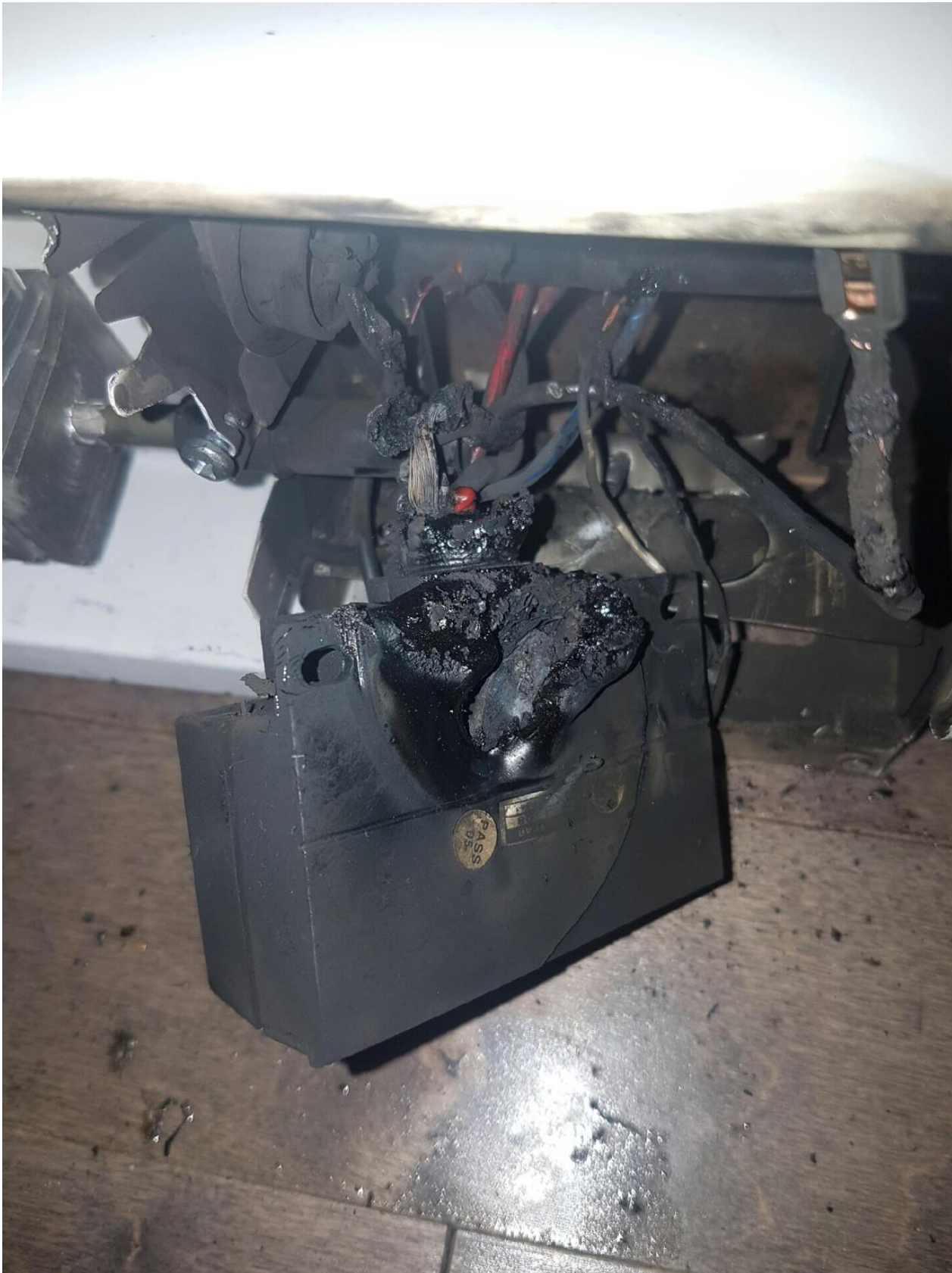
Figure #2 - Photo of relay with the side of the enclosure melted. Also showing the 240 volt and 24 volt wiring were not in separate compartments as per the manufacturer's instructions.
