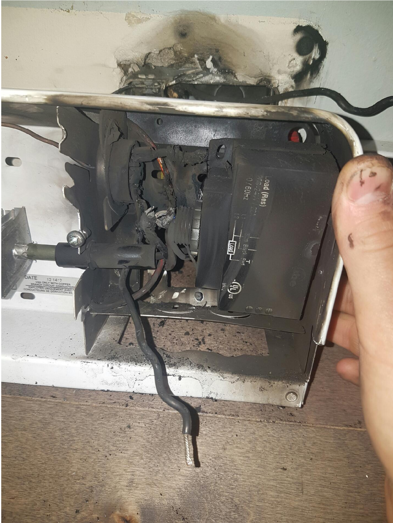
Figure #5 - Photo showing that the relay was not securely mounted as per the manufacturer's instructions.
