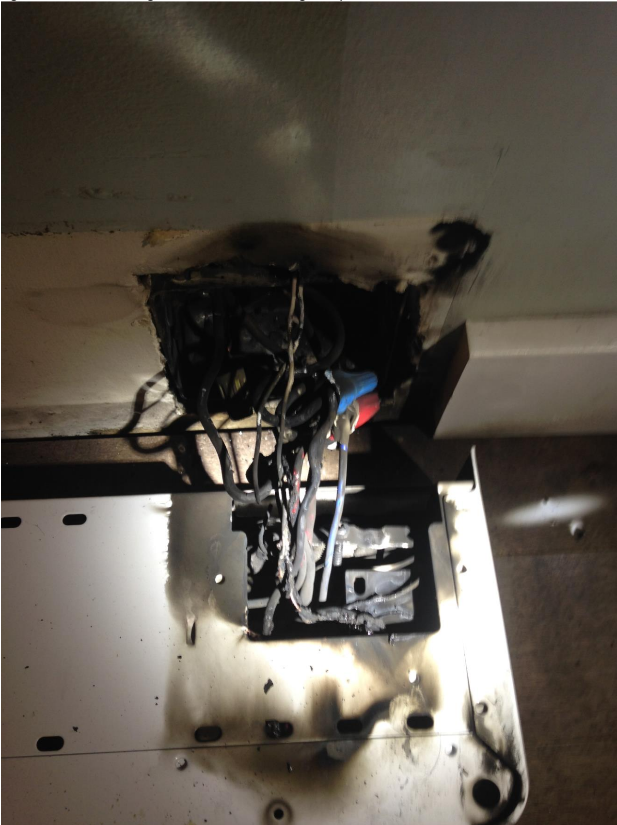
Figure #4 – Photo showing baseboard heater missing back plate.
