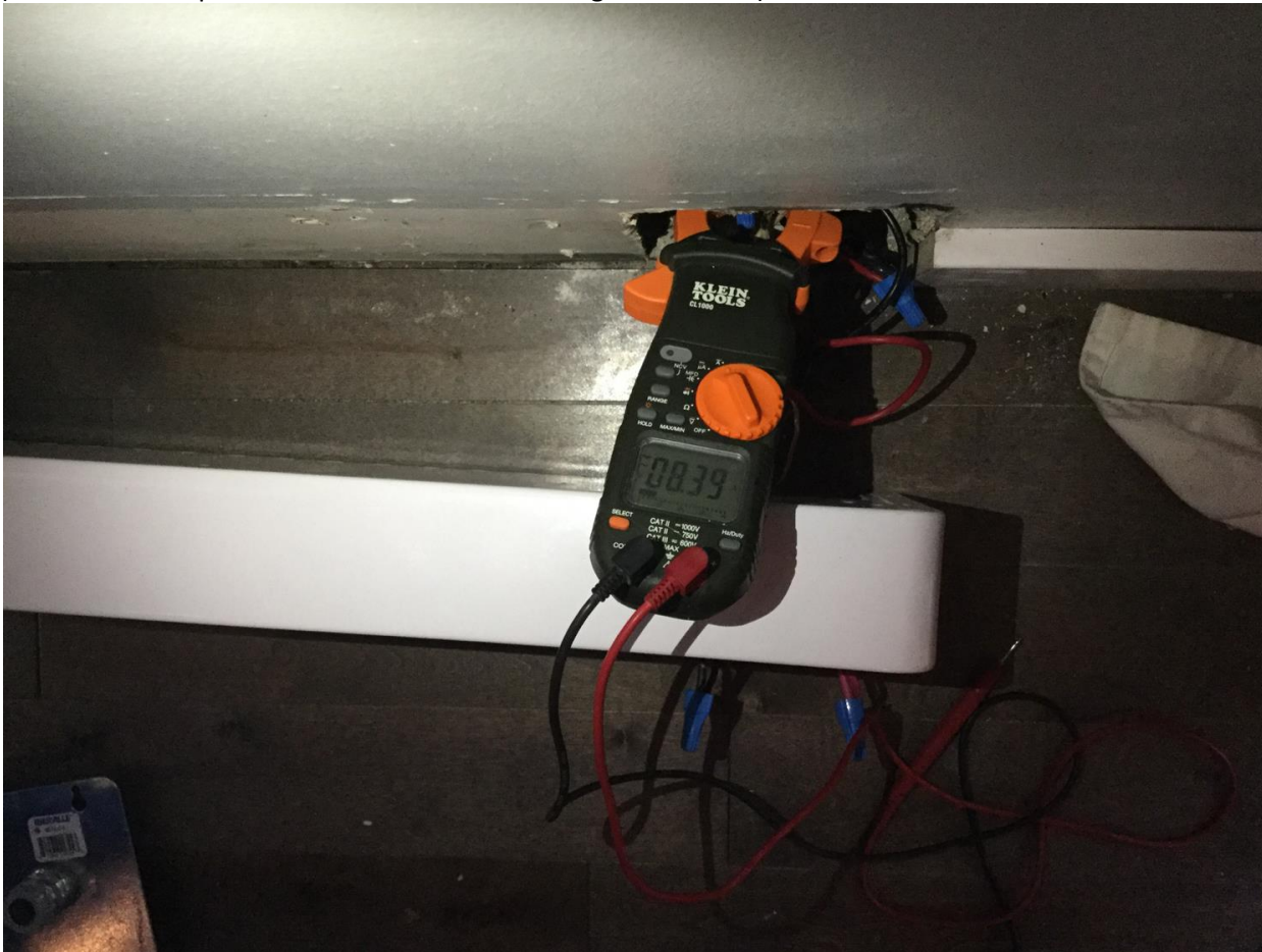
Figure #3 - Photo showing the circuit loaded at 8 amps on a 22 amp relay within tolerable levels. (Circuit and components rewired similar to during the incident)
