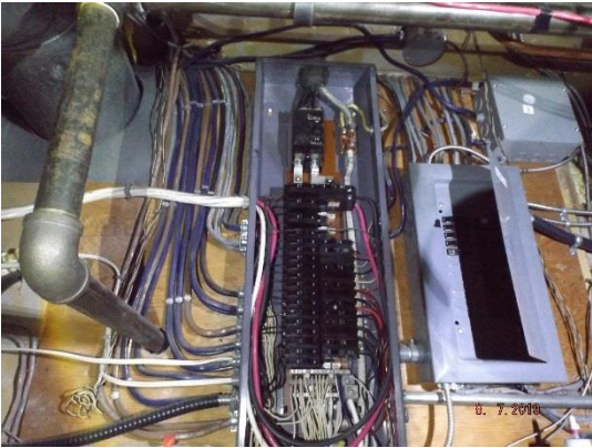
Photo 4: The main breaker did not trip during the fault. The location is difficult to work around.
