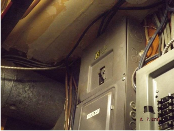
Photo 1: Panel location in basement. Utility room
