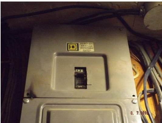
Photo 2: Panel mounted too high
