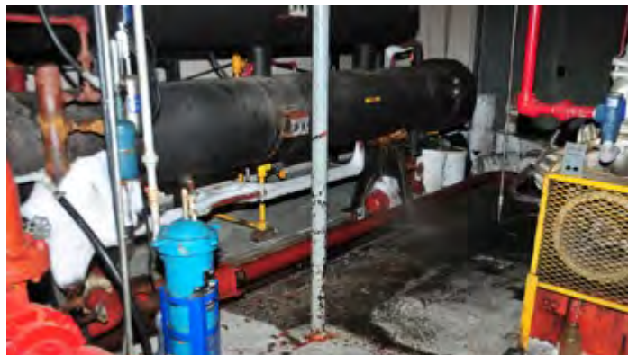
Photo 11: Projected contents of the brine piping from the separated coupling.
