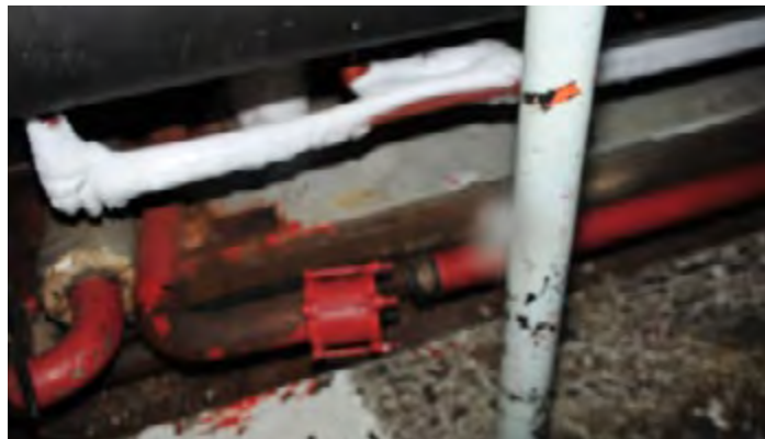
Photo 10: Separated coupling and projected brine system contents. Photo taken on October 18, 2017.
