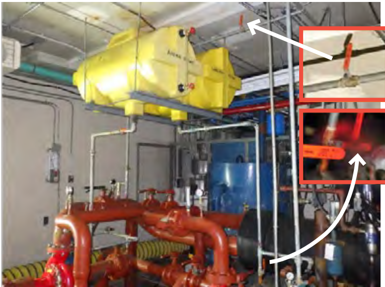
Photo 5: Brine expansion tanks – closed valve positions as found after incident shown in photo insets. Main photo taken after hazardous material removal.
