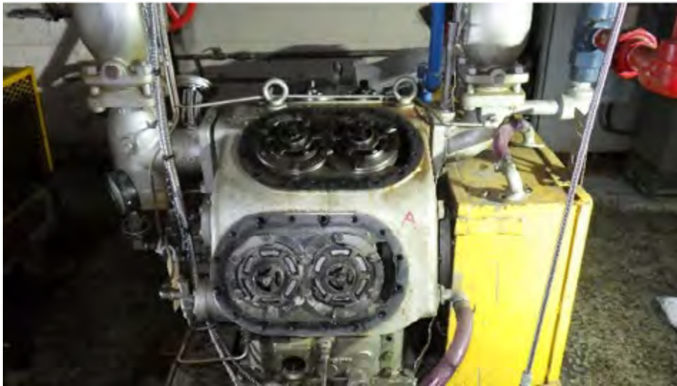
Photo 6: Compressor #2 (#1 similar) showing salt crystal build-up on lower compressor cylinder heads, upper heads were clean.
