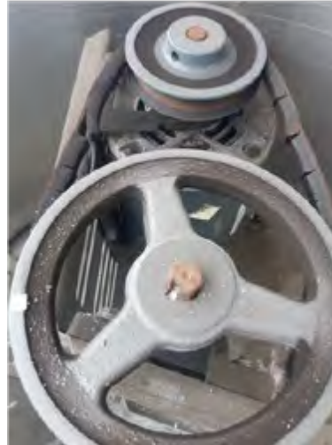
Photo 13 (above): Leak/Rupture Fan Motor, Pulley and Damaged Belt.
