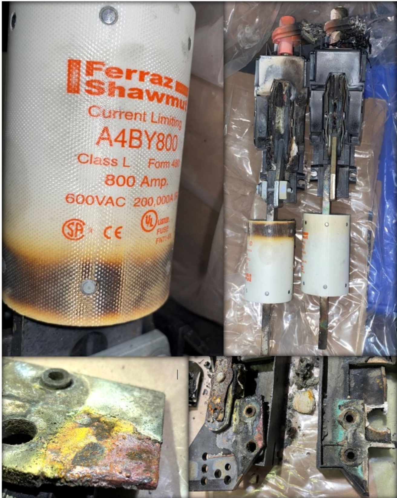
Image 3 - 800 Amp service switch fuses and mechanisms with heat/ melting damage
