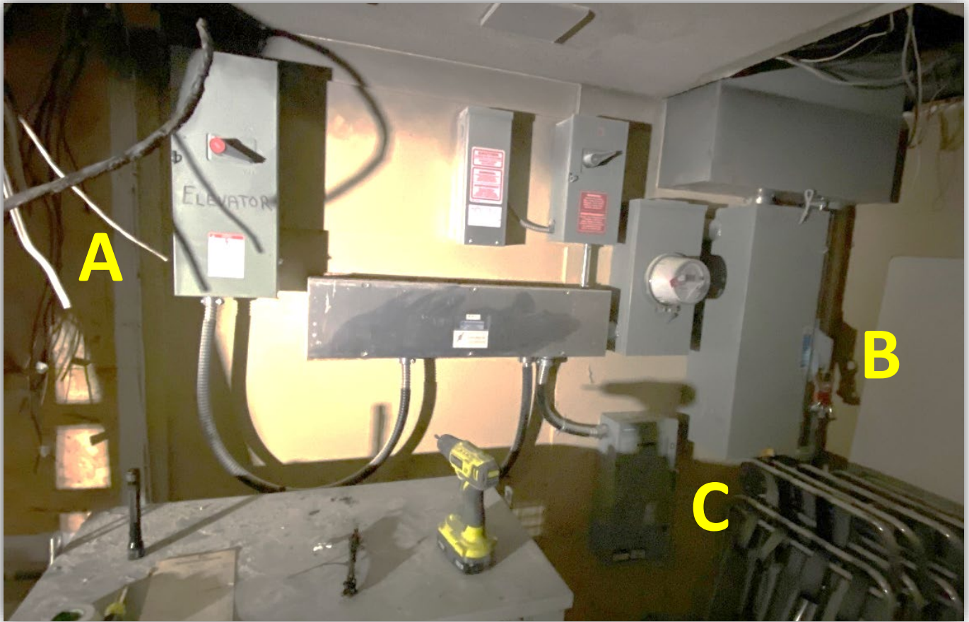
Image 6 – Service disconnect in relation to the damaged electrical panel. [A] Location of the damaged panelboard after being removed. [B] Main service disconnect. [C] Transformer / panelboard disconnect.
