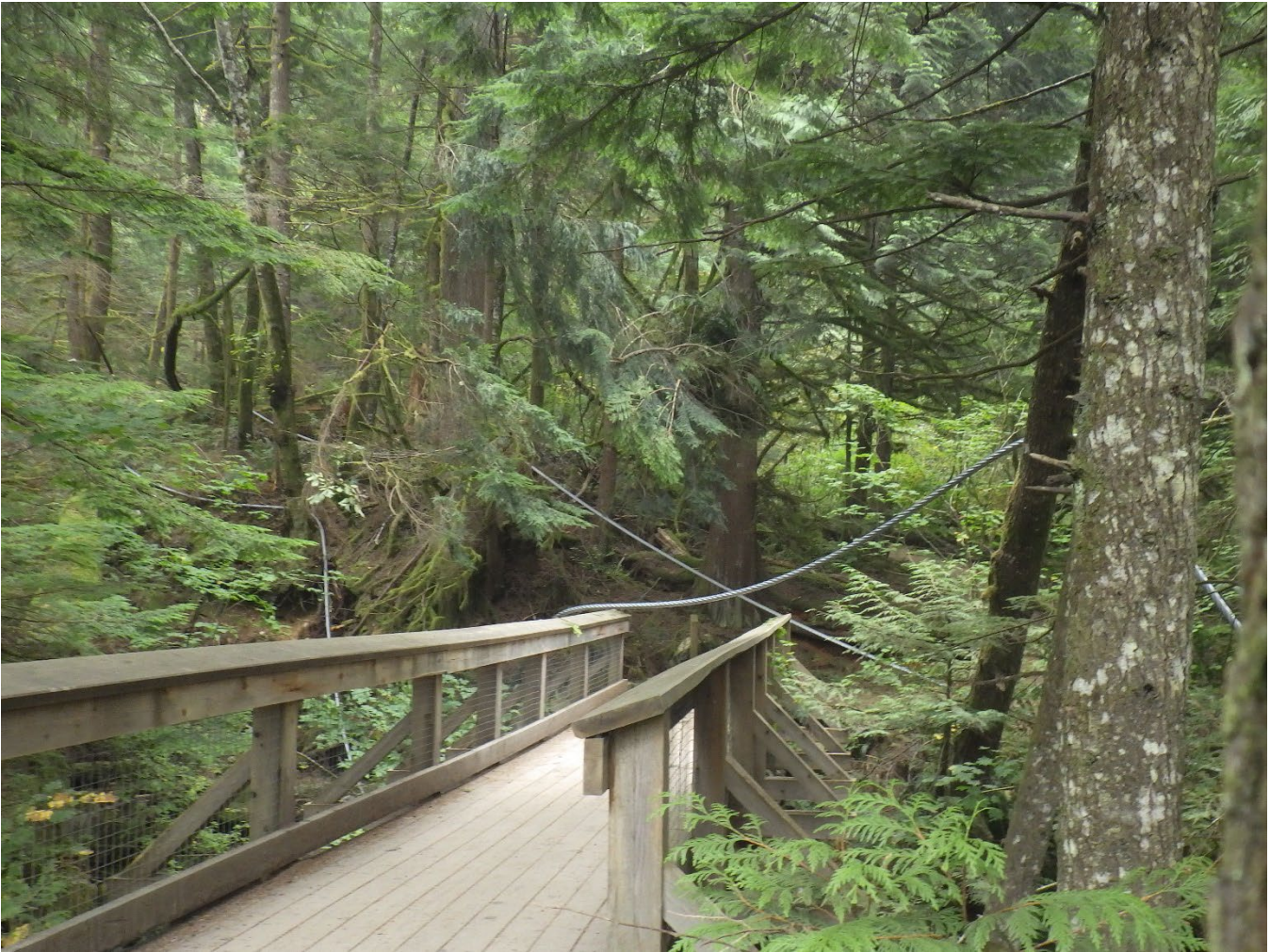
Image 5 – Fallen haul rope lying across public trail
