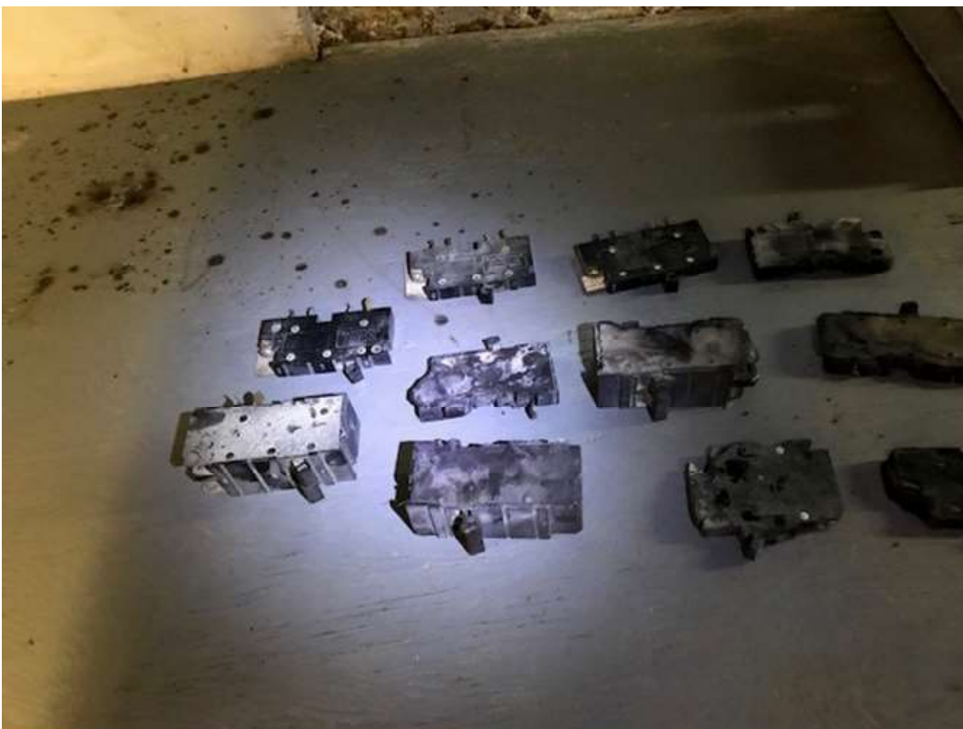
Photo of the damaged breakers that were installed within the load center
