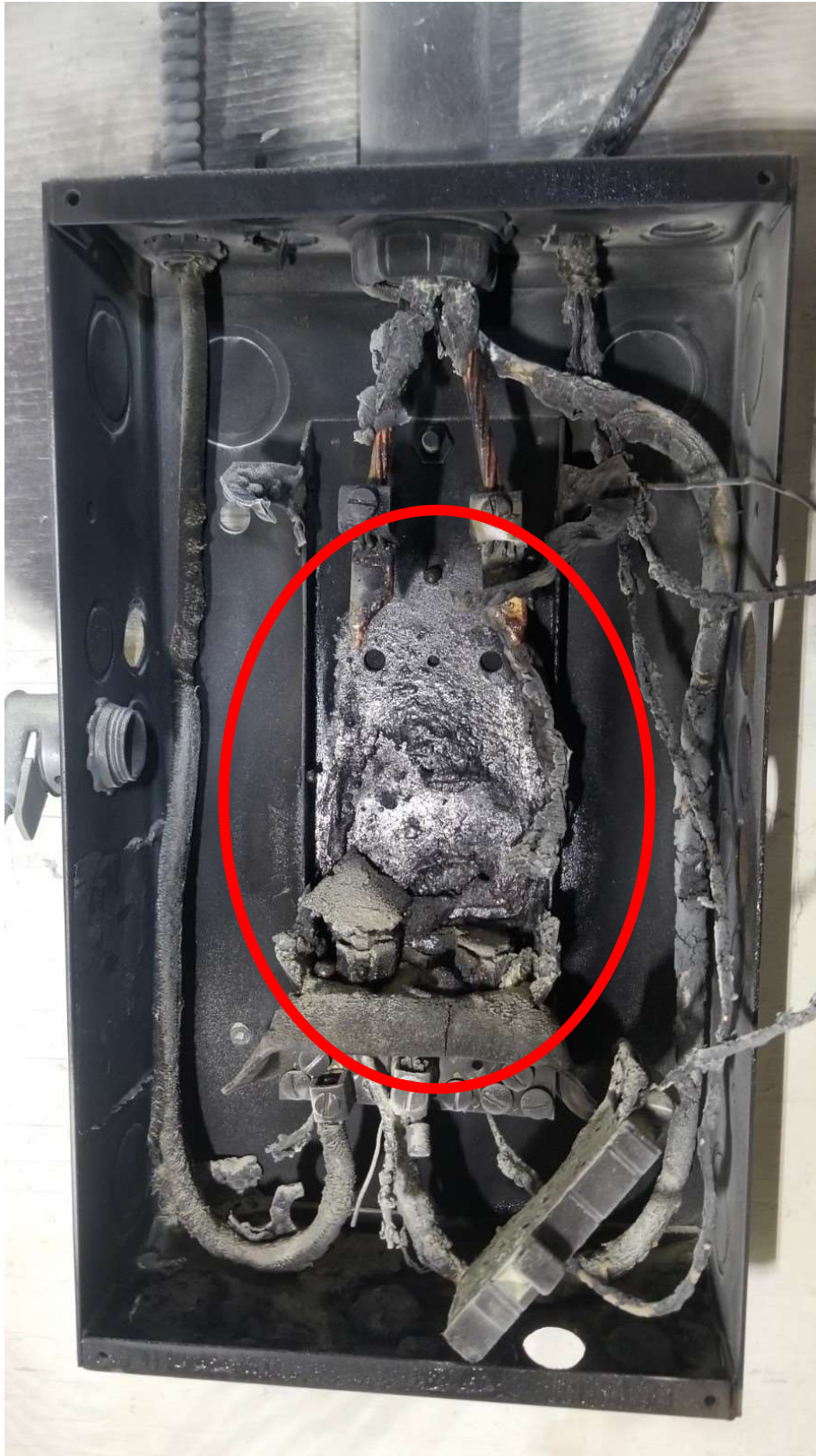
Photo taken of the inside of the panel after the incident. Observe within the red - the area of the large fault occurrence and rapid energy release.
