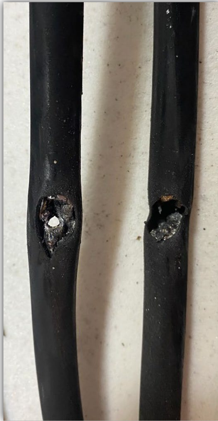
Image 4 - Close up of the ungrounded service conductor on the left showing where the wood screw penetrated through the internal aluminum conductors and the neutral conductor on the right which the tip of the wood screw penetrated and where most of the internal aluminum conductors melted due to the generated heat while not entirely severing the neutral conductor.
