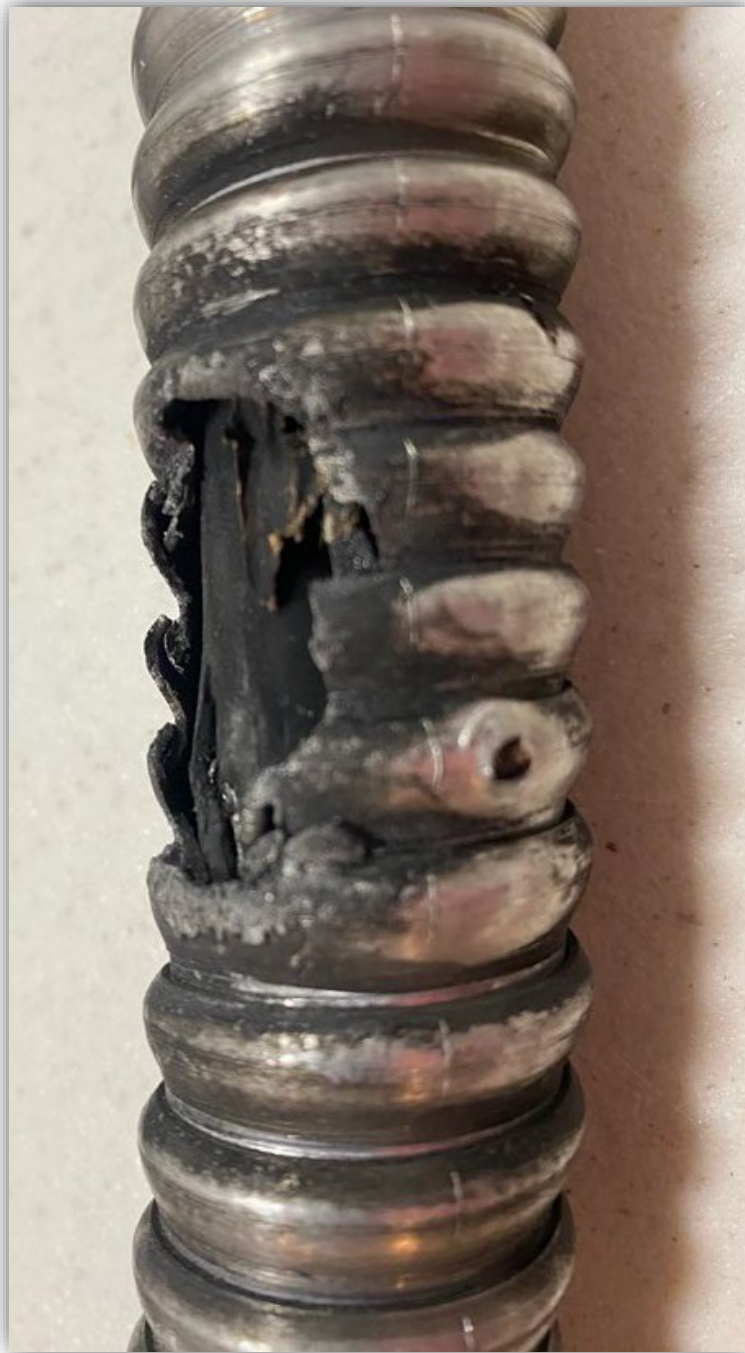
Image 2- Rubber outer jacket of cable removed showing entry point of wood screw and area where armoured jacket melted due to the generated heat from the short circuit.
