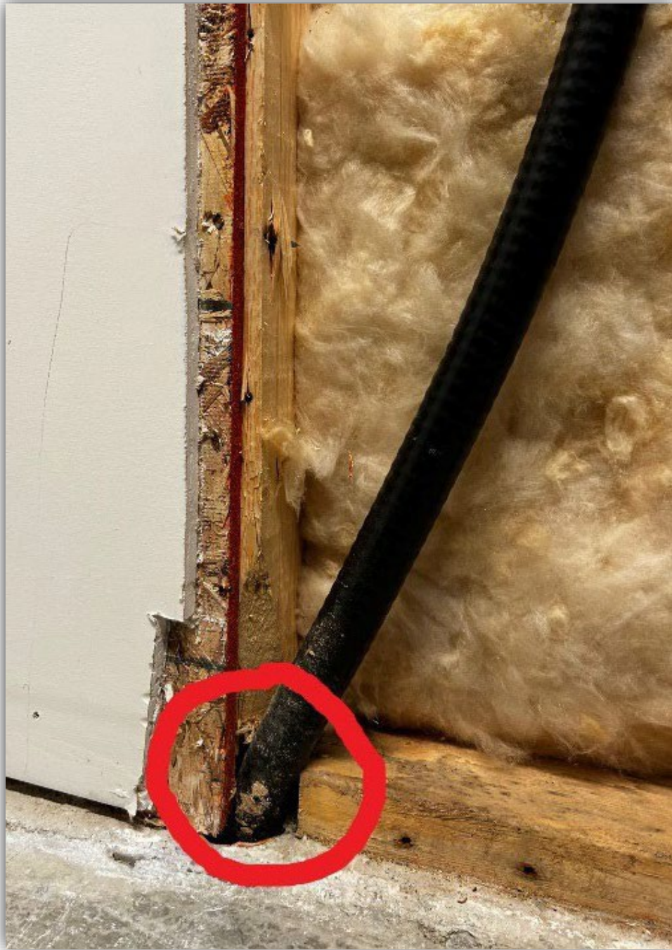
Image 1 - Location where wood screw penetrated the ACWU cable.
