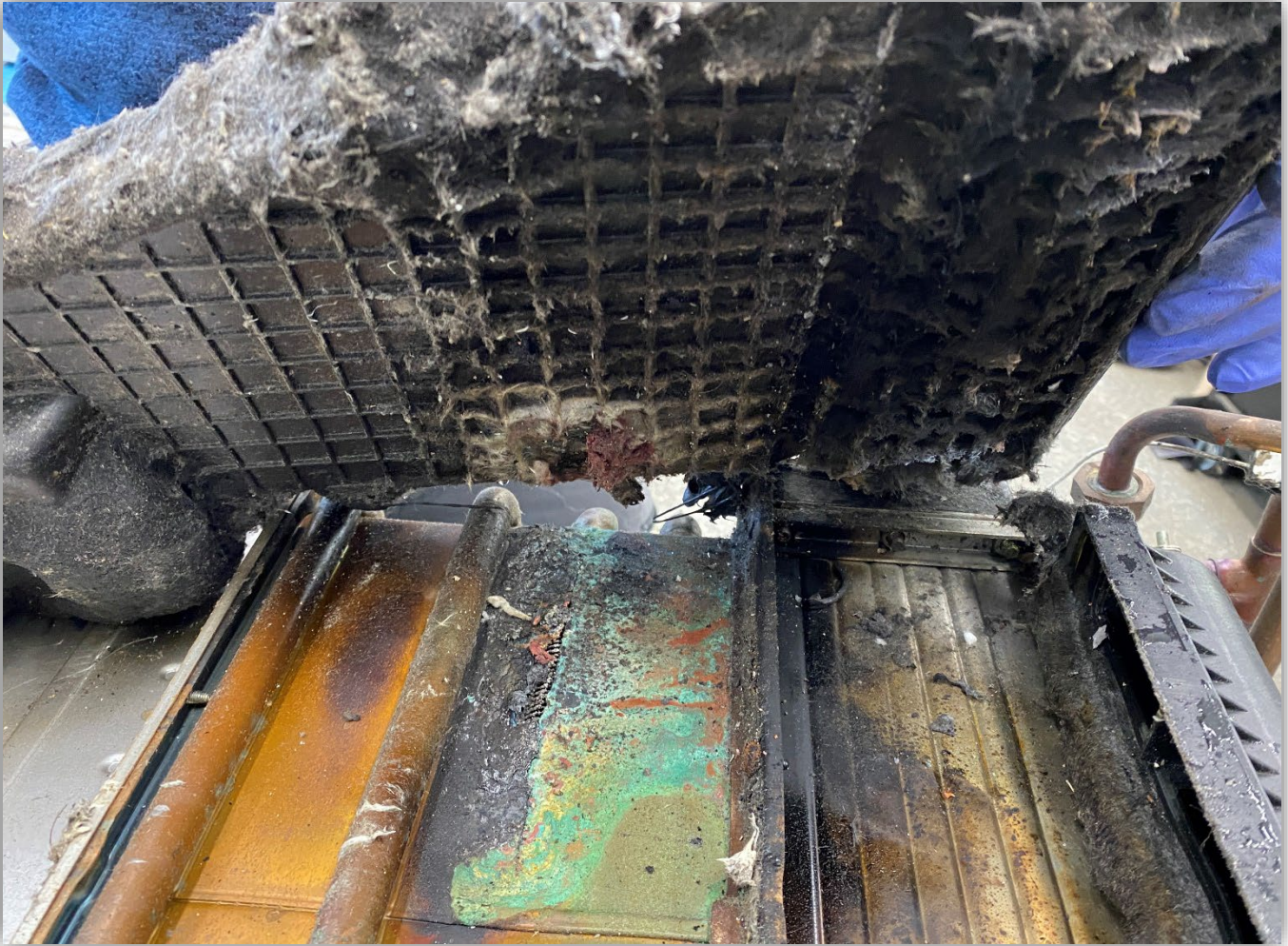
Image 5 – Damaged flue gas collector duct and rear of combustion chamber.
