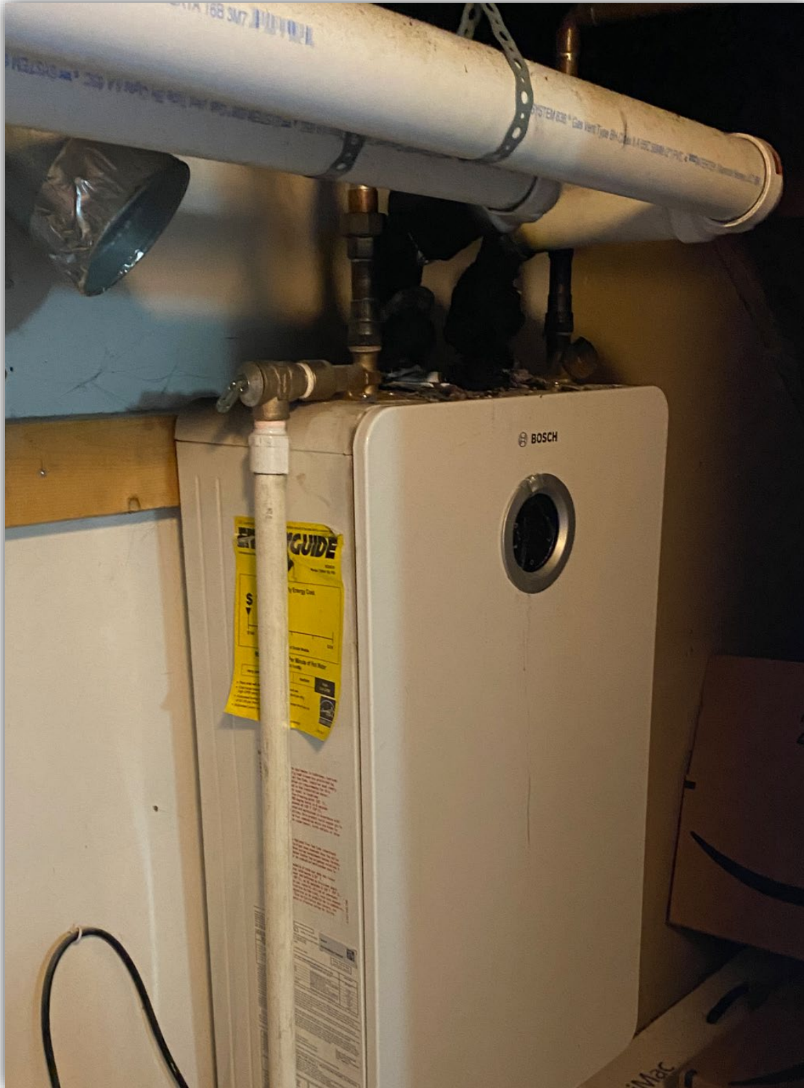
Image 1 – On-demand water heater installed in the mechanical room.
