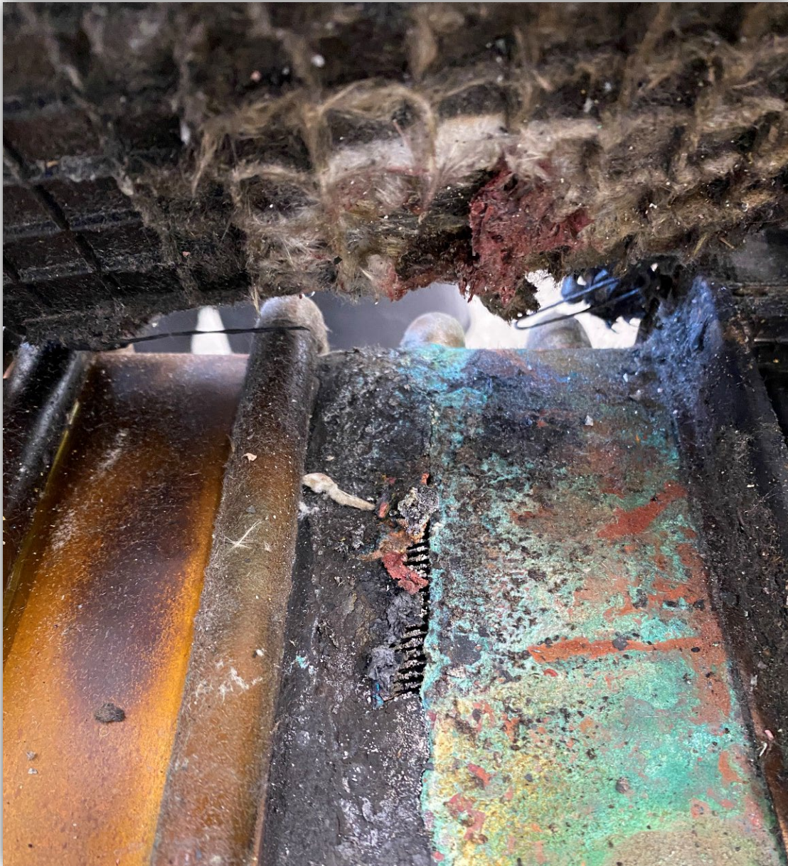
Image 6 – Closeup of damage and hole in the combustion chamber.
