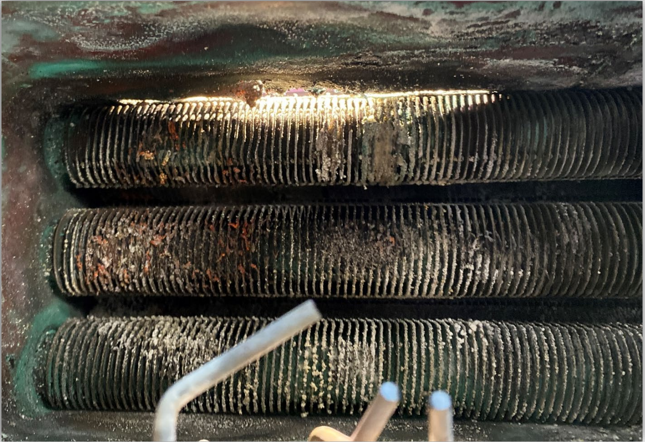
Image 10 – Primary heat exchange tubes with light shining through the hole in the combustion chamber.
