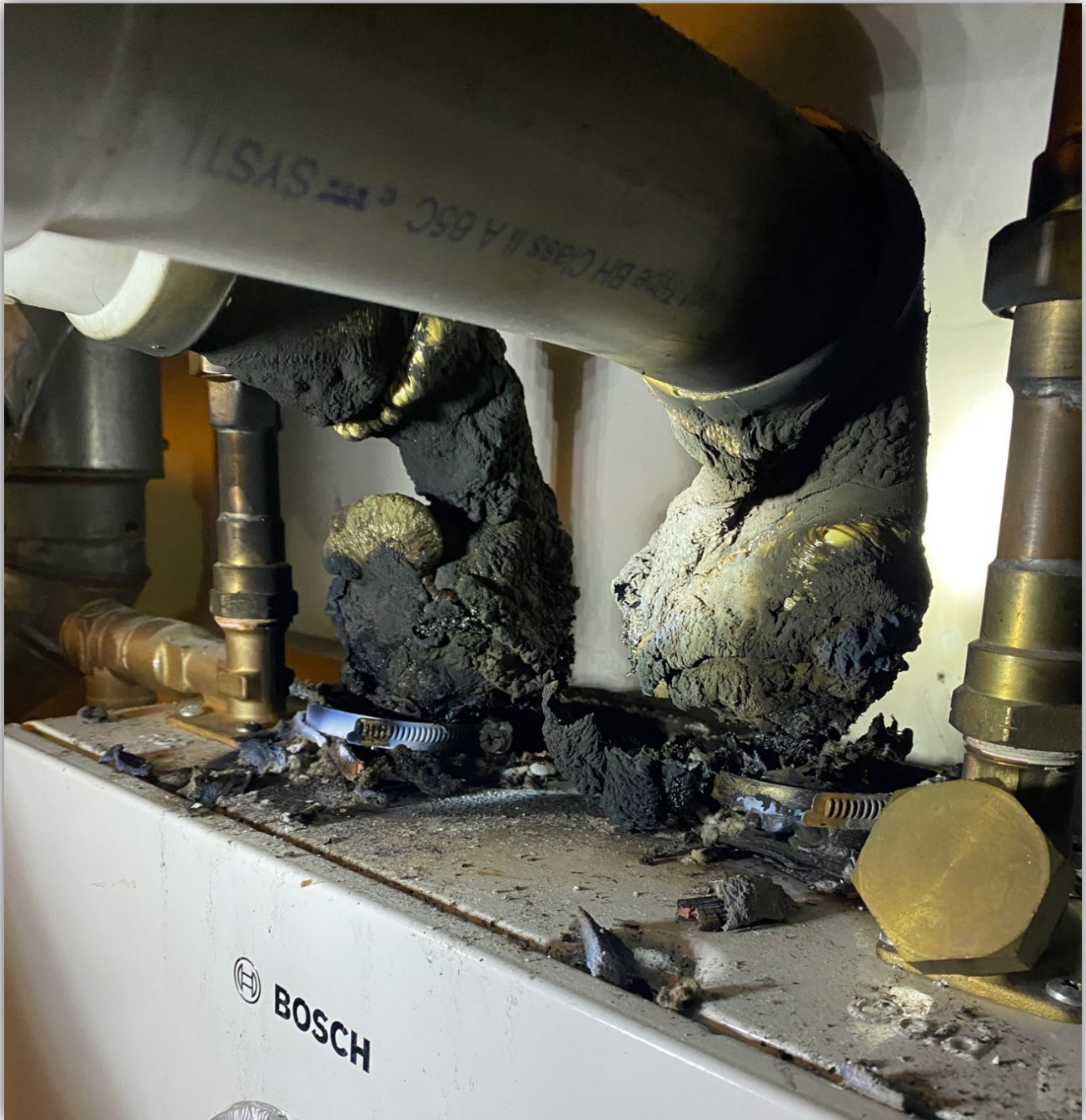
Image 2 – Fire damaged venting and combustion air PVC piping.
