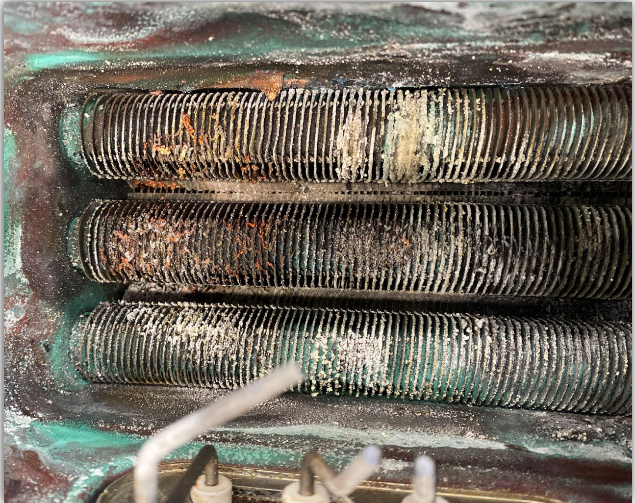
Image 9 – Corrosion and scale buildup on the internal primary heat exchanger tube fins restricting flue gas flow.
