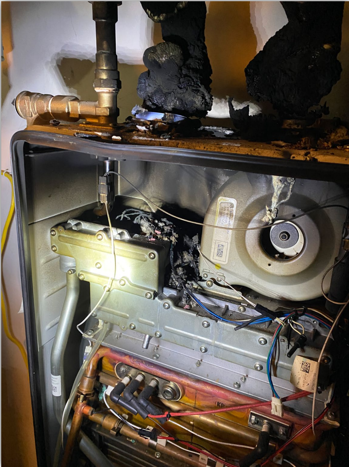
Image 3 – Heat and fire damaged internal components inside the water heater.
