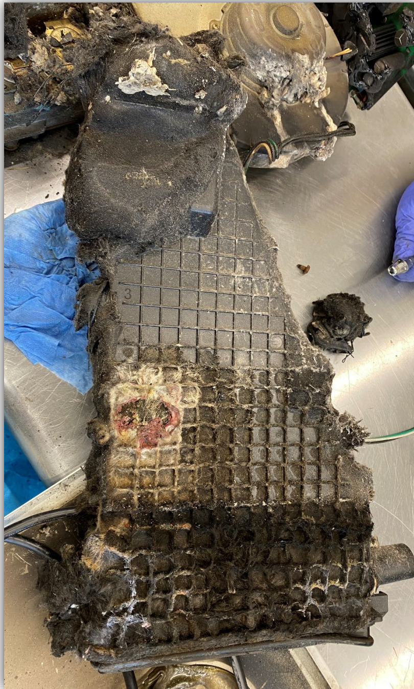
Image 7 – Damaged composite flue gas collector duct.
