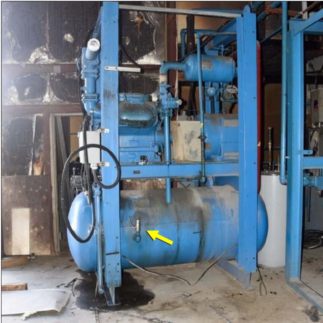
Figure 1 Overall view of subject valve installed vertically on ammonia tank (arrow). Lever is in "open" position with outlet side of valve in the upward position (site photo).
