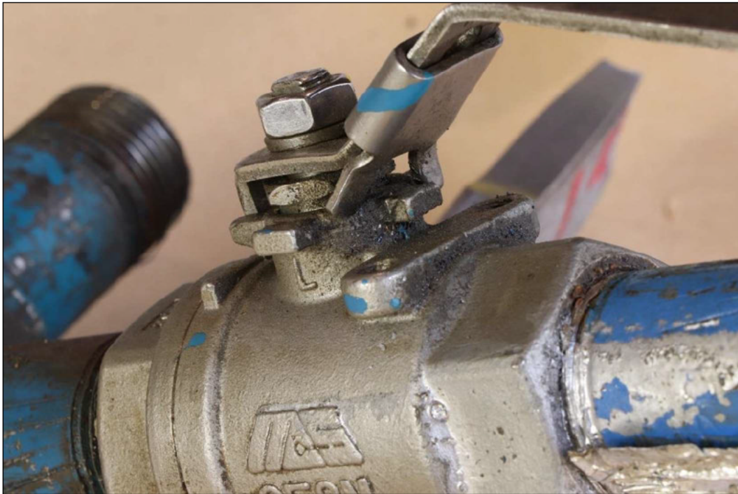
Figure 4 View of deformed locking tab showing deformation preventing proper sliding and positioning of the locking tabs; however, the valve can be opened and closed normally.
