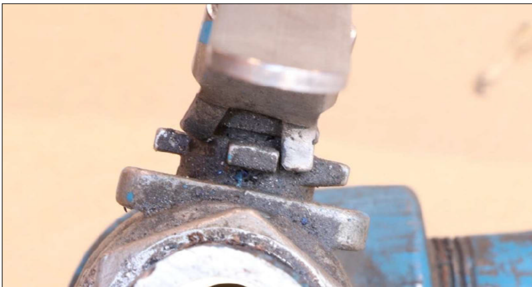
Figure 5 Close-up view of deformed locking tab. Tab can slip by cast-in stop.
