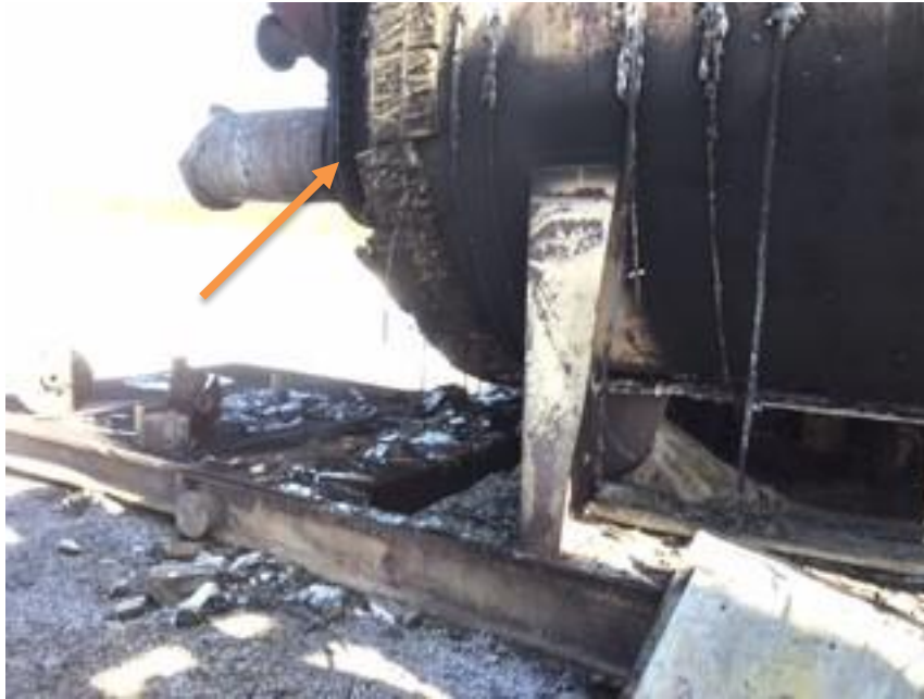
Treater Burner End skid and Support Brace
