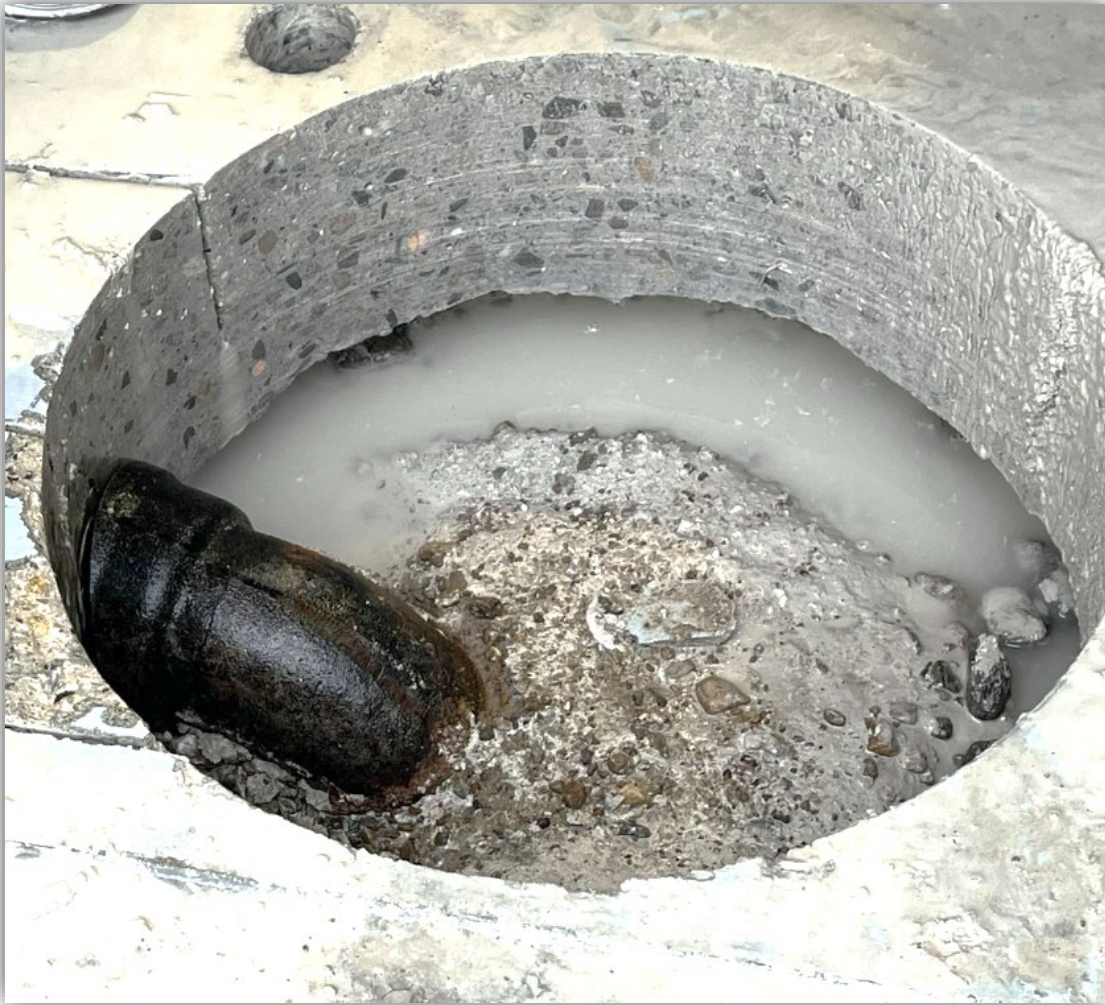
Image 2 - Original coring hole that hit watermain's cast iron pipe fitting that was encased in concrete.
