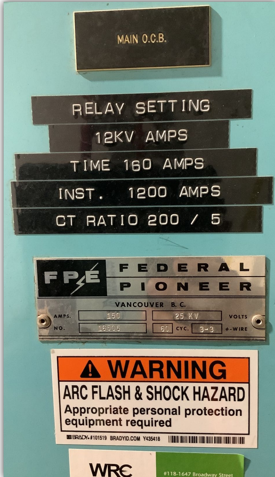
Image 5 - High Voltage Unit Sub-station labelling.
