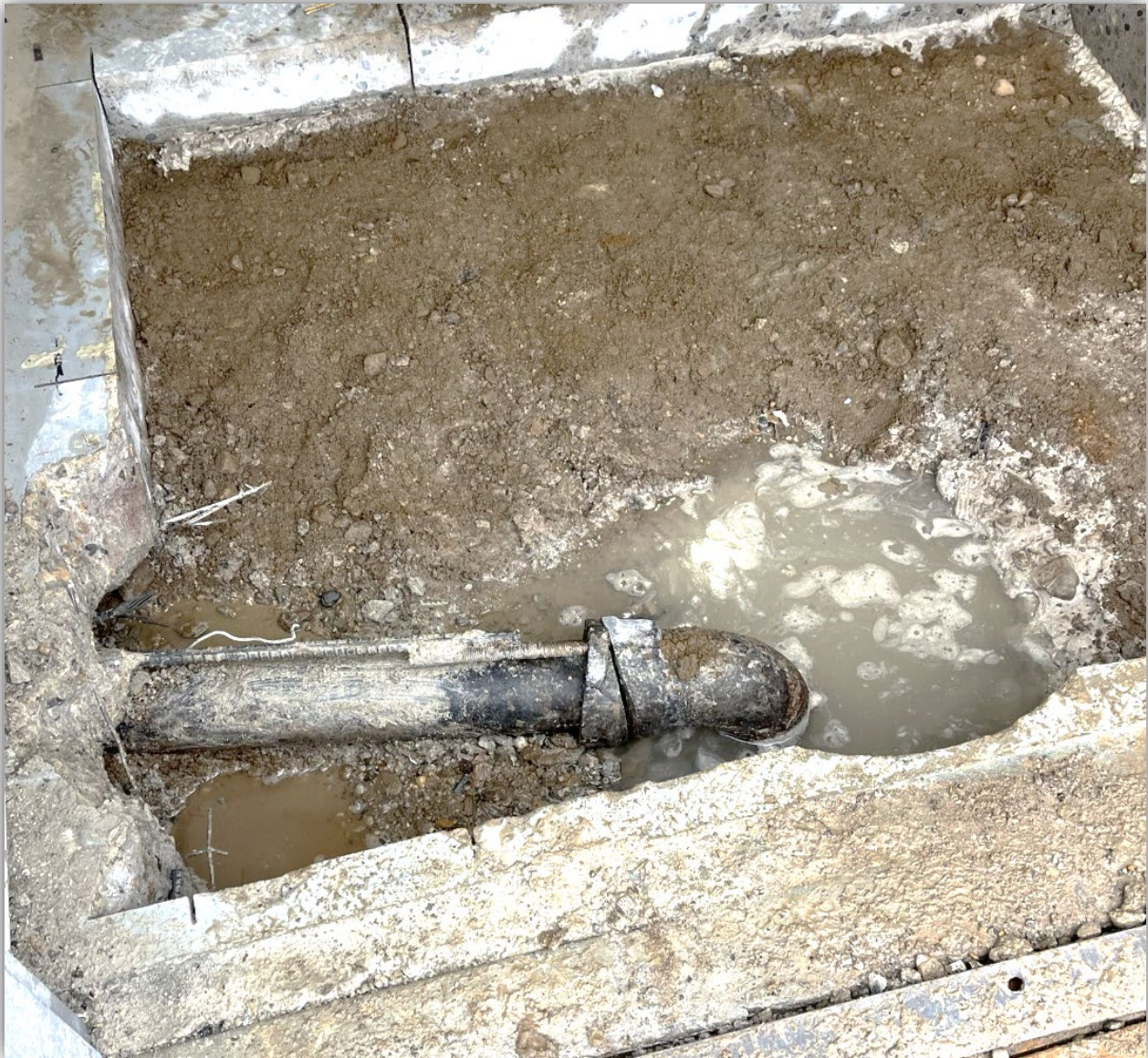
Image 3 - Remaining floor cut open, exposing damaged waterline. Saw cut can be seen to cast iron elbow on the top, where it runs horizontally.
