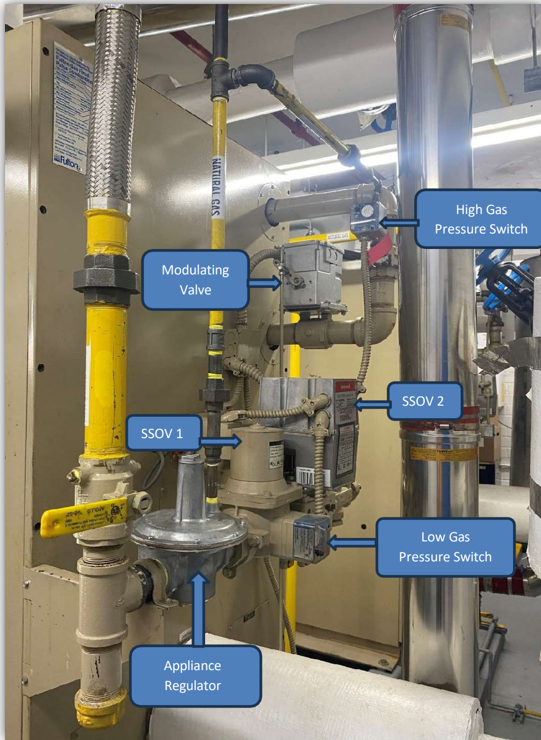
Image 3 - Boiler Valve Train Components.
