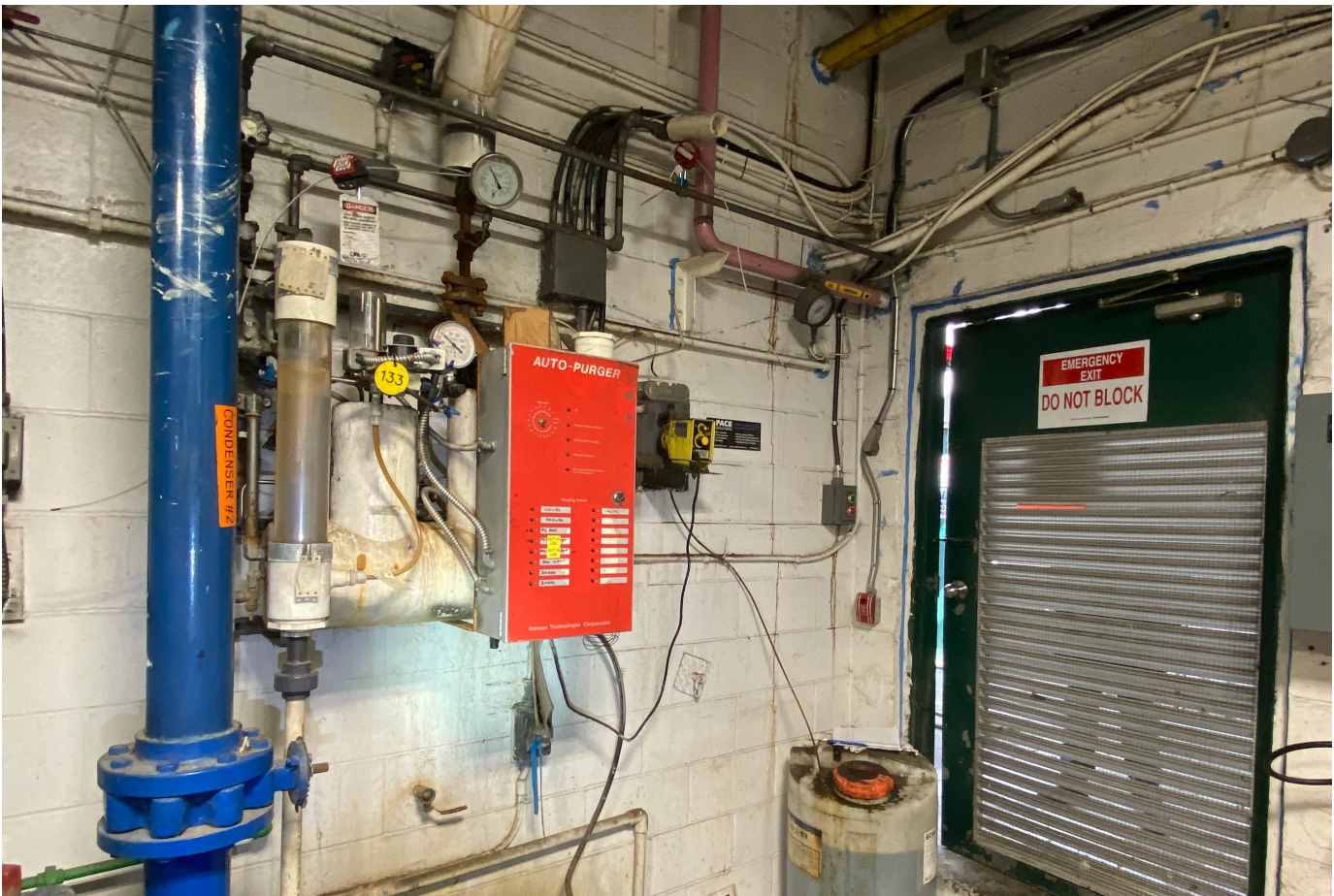
Image 2 – Auto purger installation in mechanical room.
