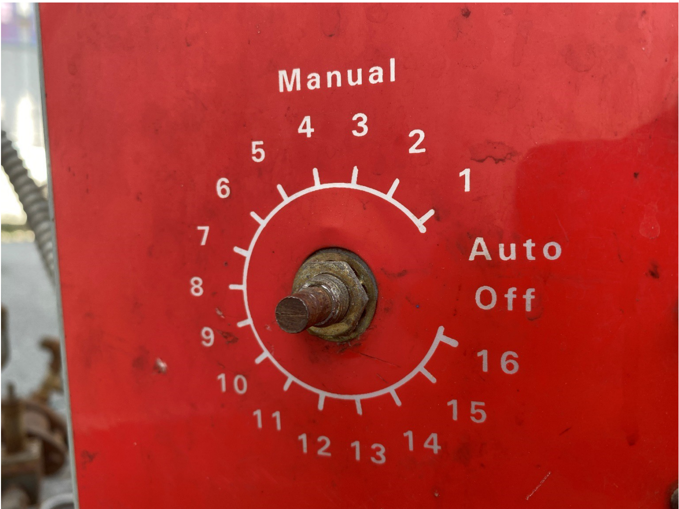
Image 5 – Auto-purger control switch with missing knob. The end of the switch shaft has a slight scribed line indicating the switches set location. It is horizontal indicating it is in the “Off” location. When tested the shaft could not be turned by hand and required tools to rotate.
