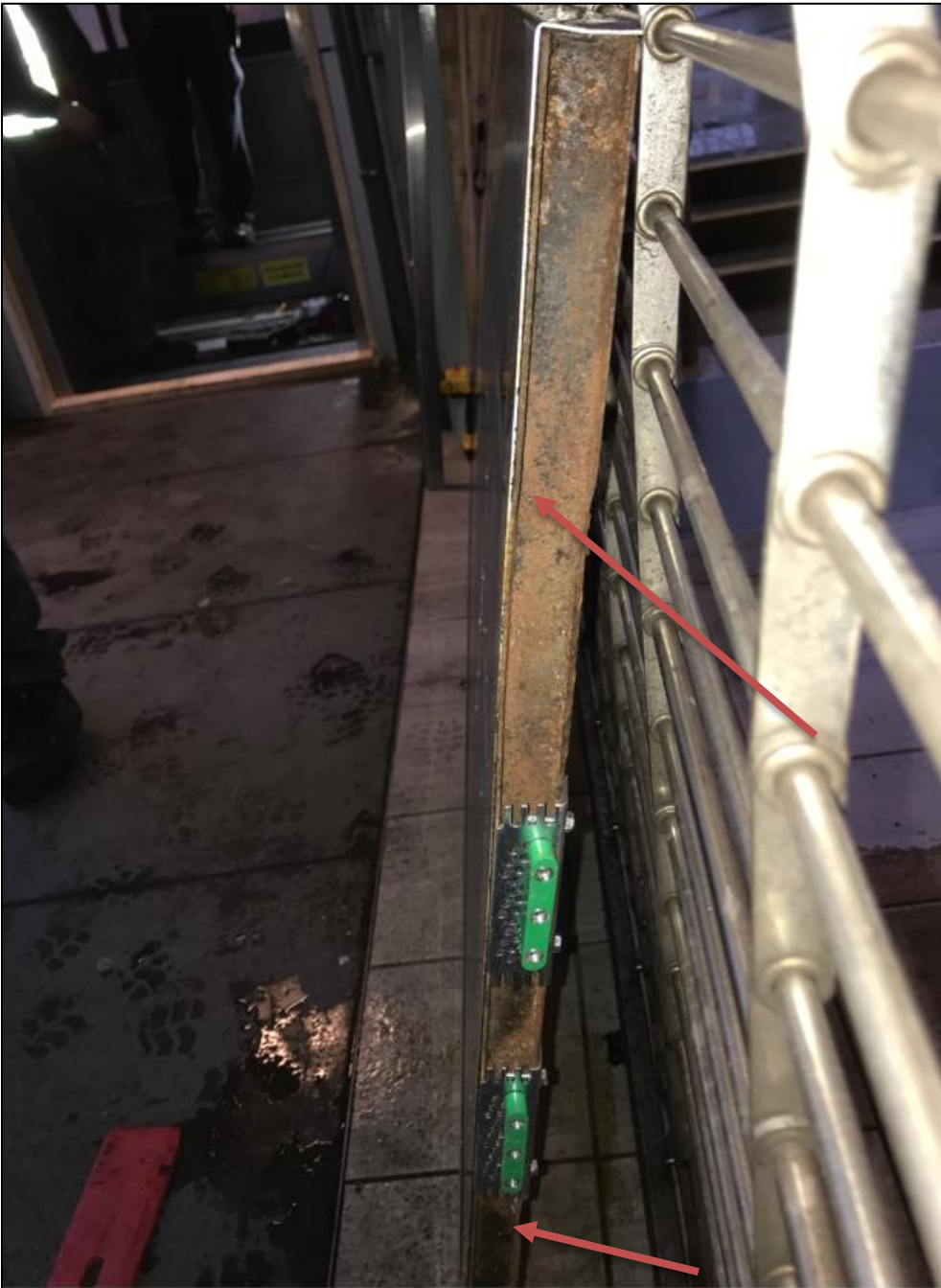
Photo 5: View of bottom of elevator door – corrosion present on bottom and some damage from impact
