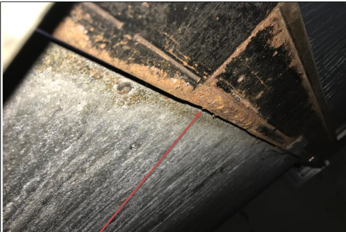
Photo 2: Corrosion of Lower Door Section
