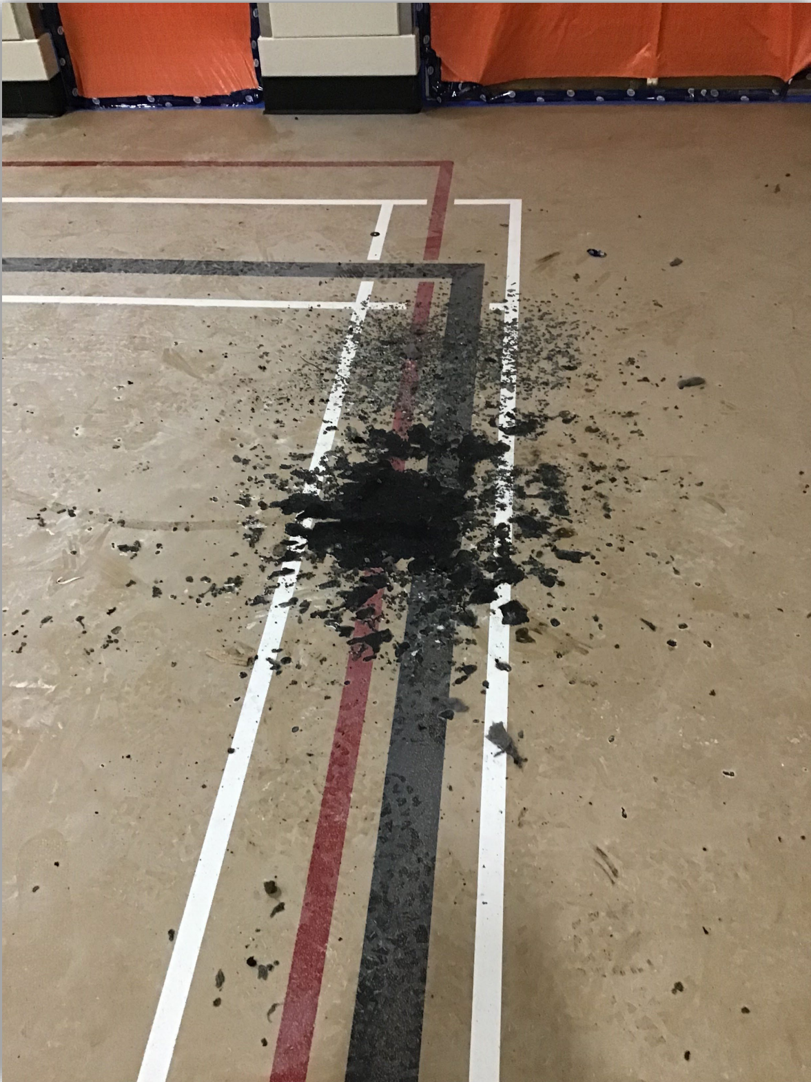
Image 2 - Floor damage directly below luminaire.
