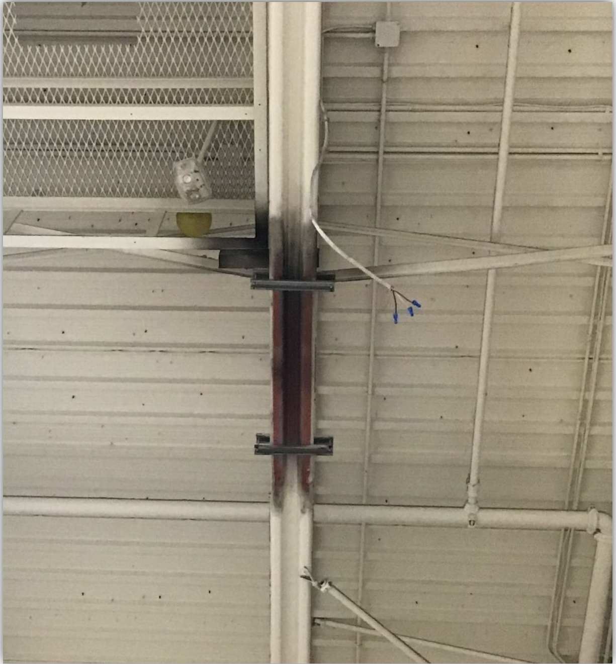
Image 1 - Heat and fire damage to area where luminaire was secured.
