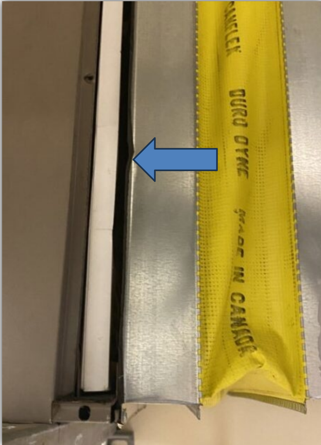
Image 6 – Unsealed AHU filter rack with arrow showing the gap that drew in the boiler exhaust.
