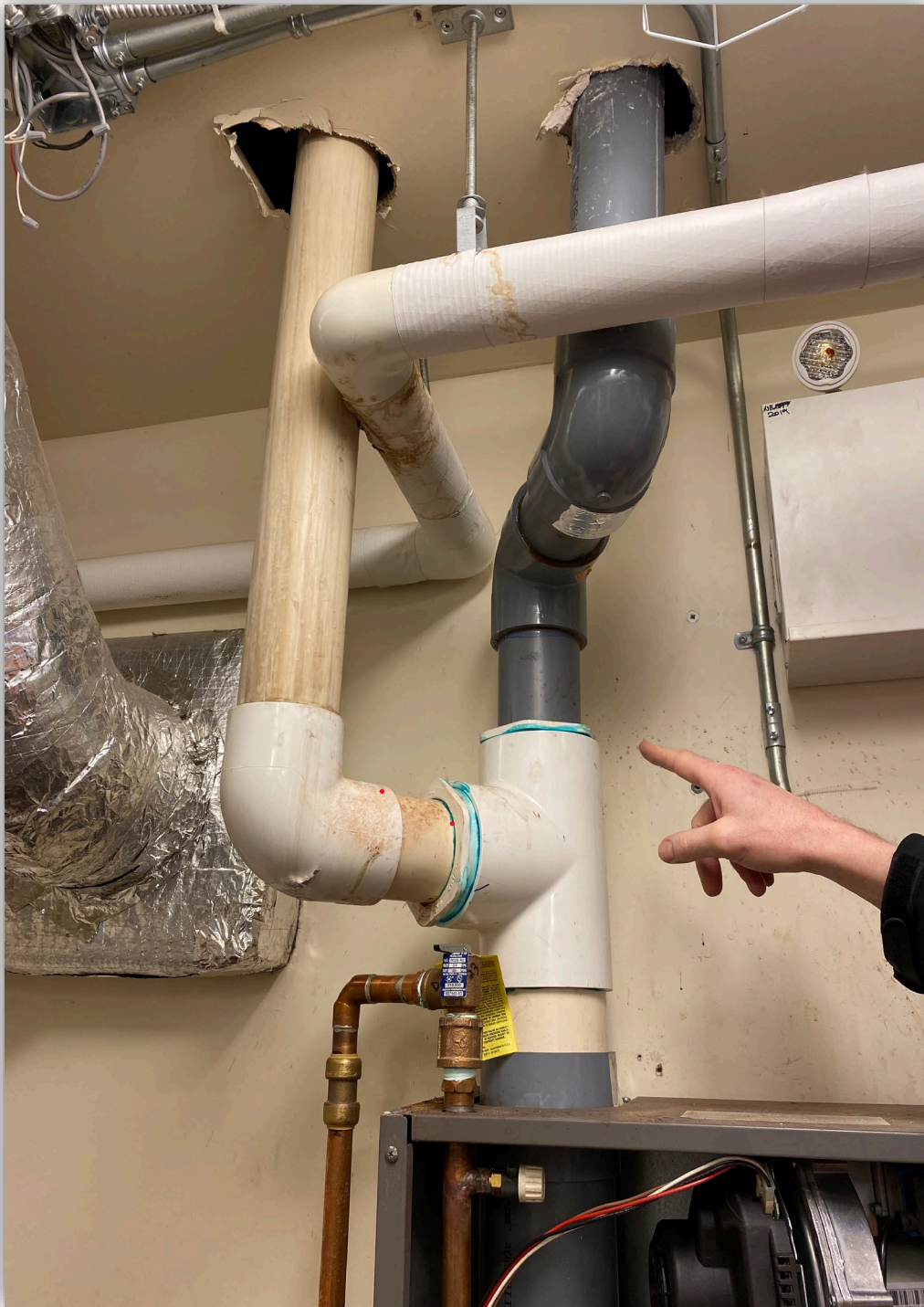
Image 3 - Exhaust piping modification that occurred sometime in the life of the appliance.
