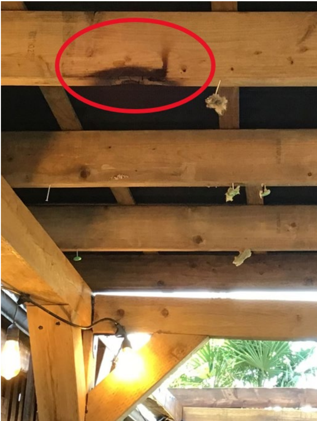
Photo 4: Charring above unit 2 when heater and metal sheeting removed.
