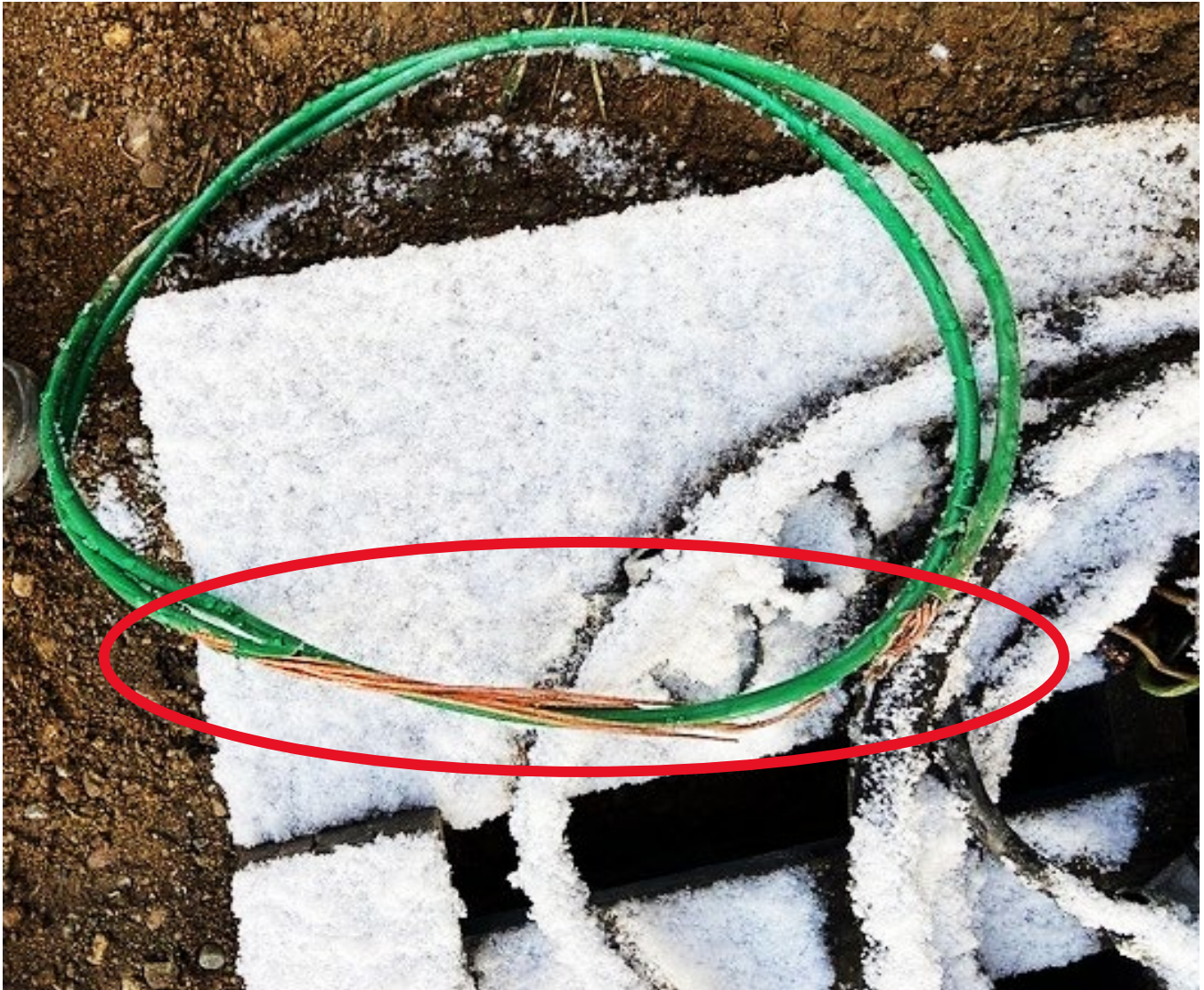
Photo 1 - Exposed copper is due to strain on conductor from excessive force from excavator.
