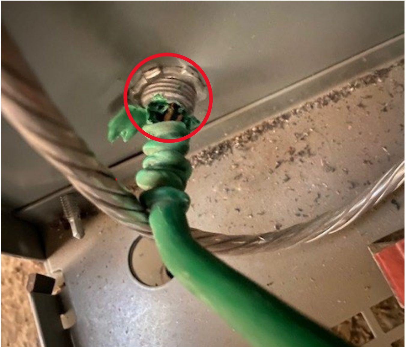
Photo 3 - Damage to grounding conductor insulation due to excess strain.
