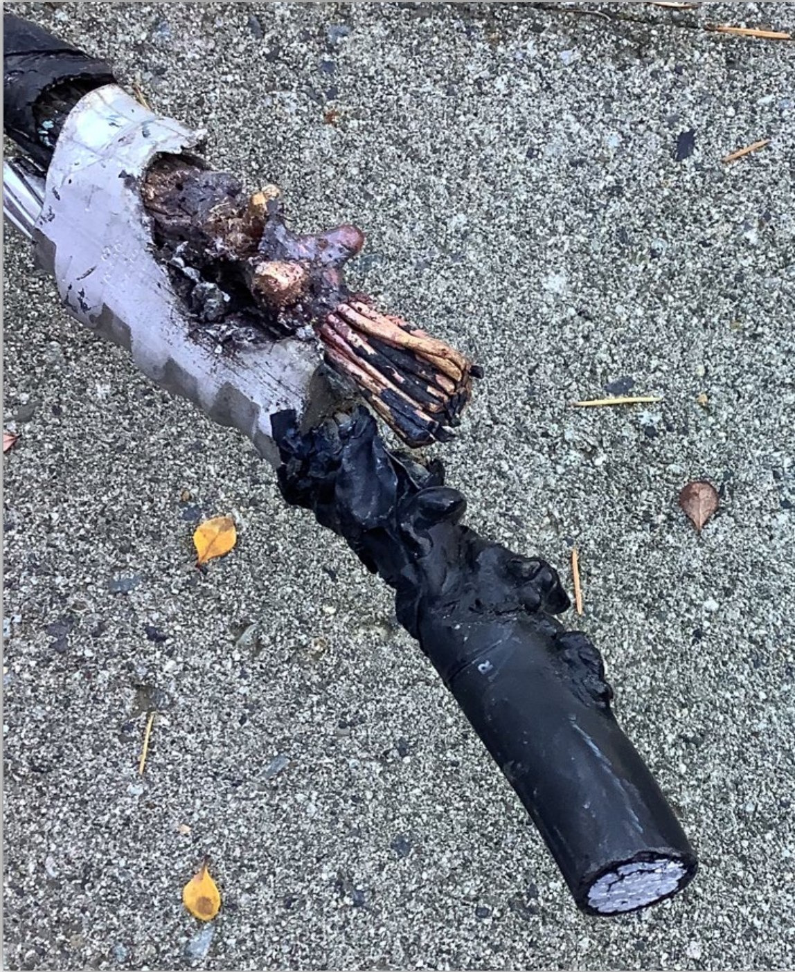
Image 6 – Molten drips and melted insulation.
