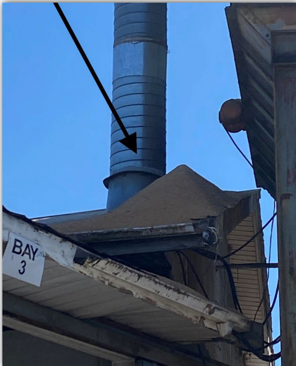
Image 5 – Dust accumulated on the roof.
