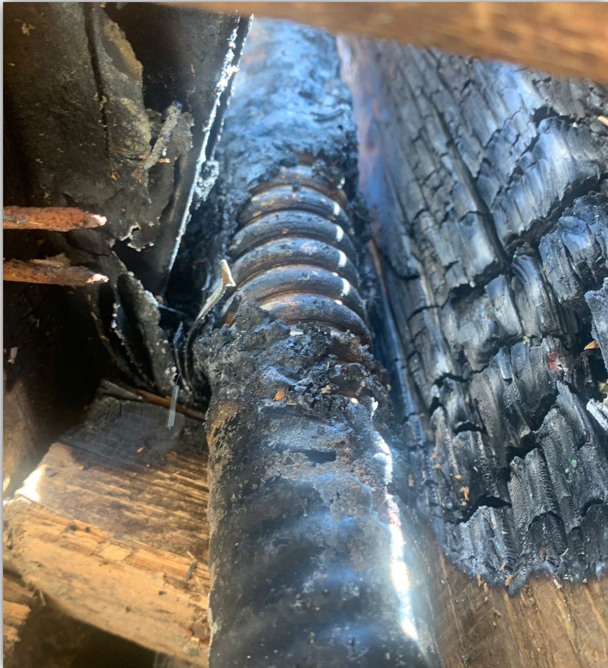
Image 4 – Soffit removed by the fire department.
