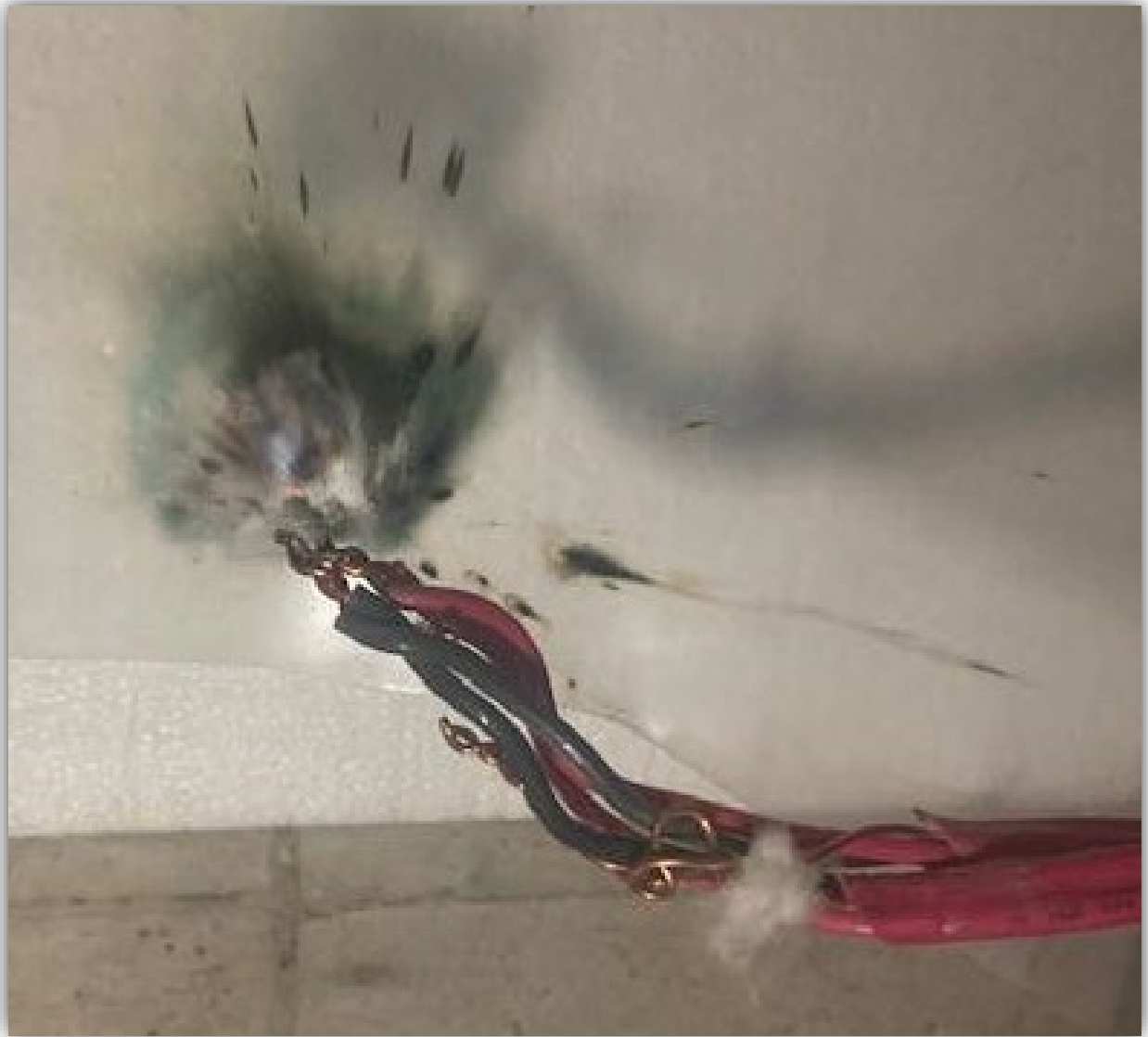
Image 5 - Live conductors that the owner contacted in the crawl space.
