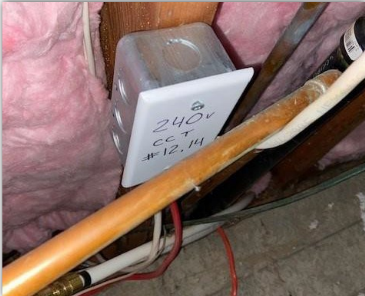
Image 3 - 2c #12 wire from panel to crawl that was feeding the exposed circuit.
