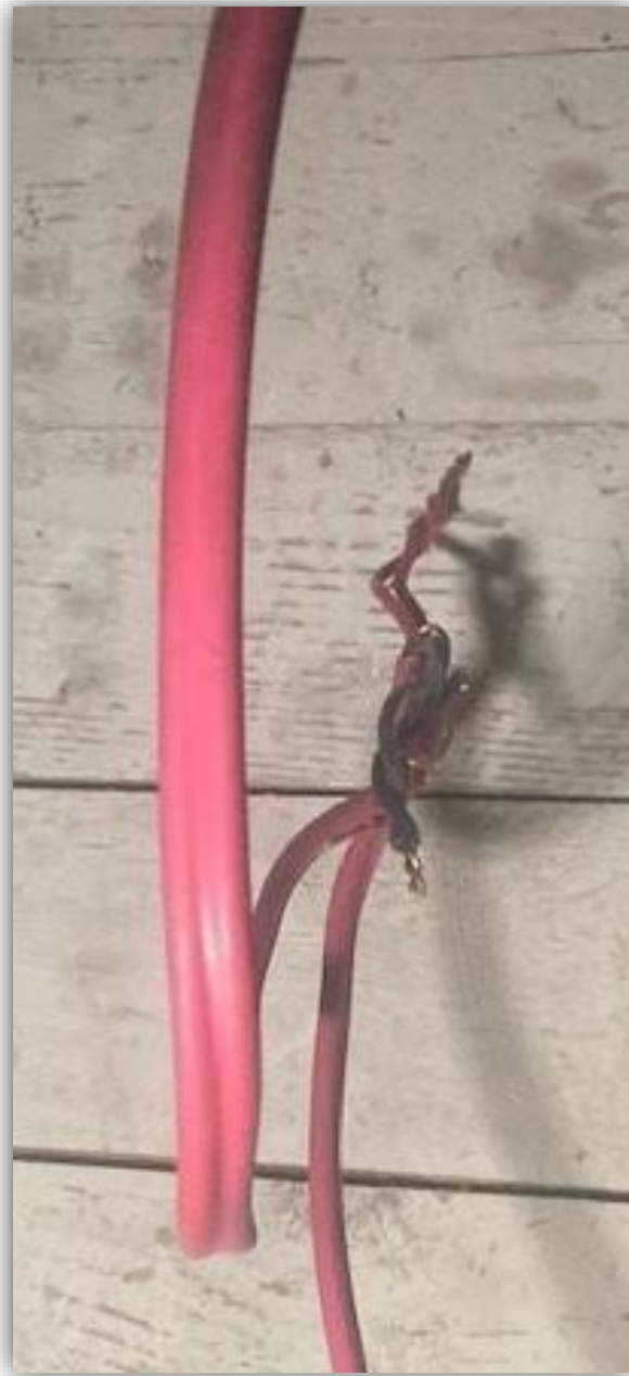
Image 4 - Bare conductors from decommissioned base board heating circuit.
