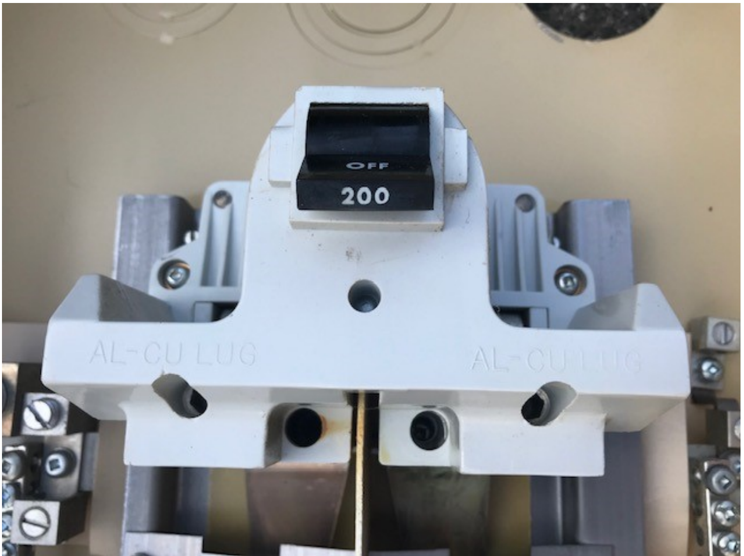
Photo 3: 200A breaker with slight discoloration on the left buss screw
