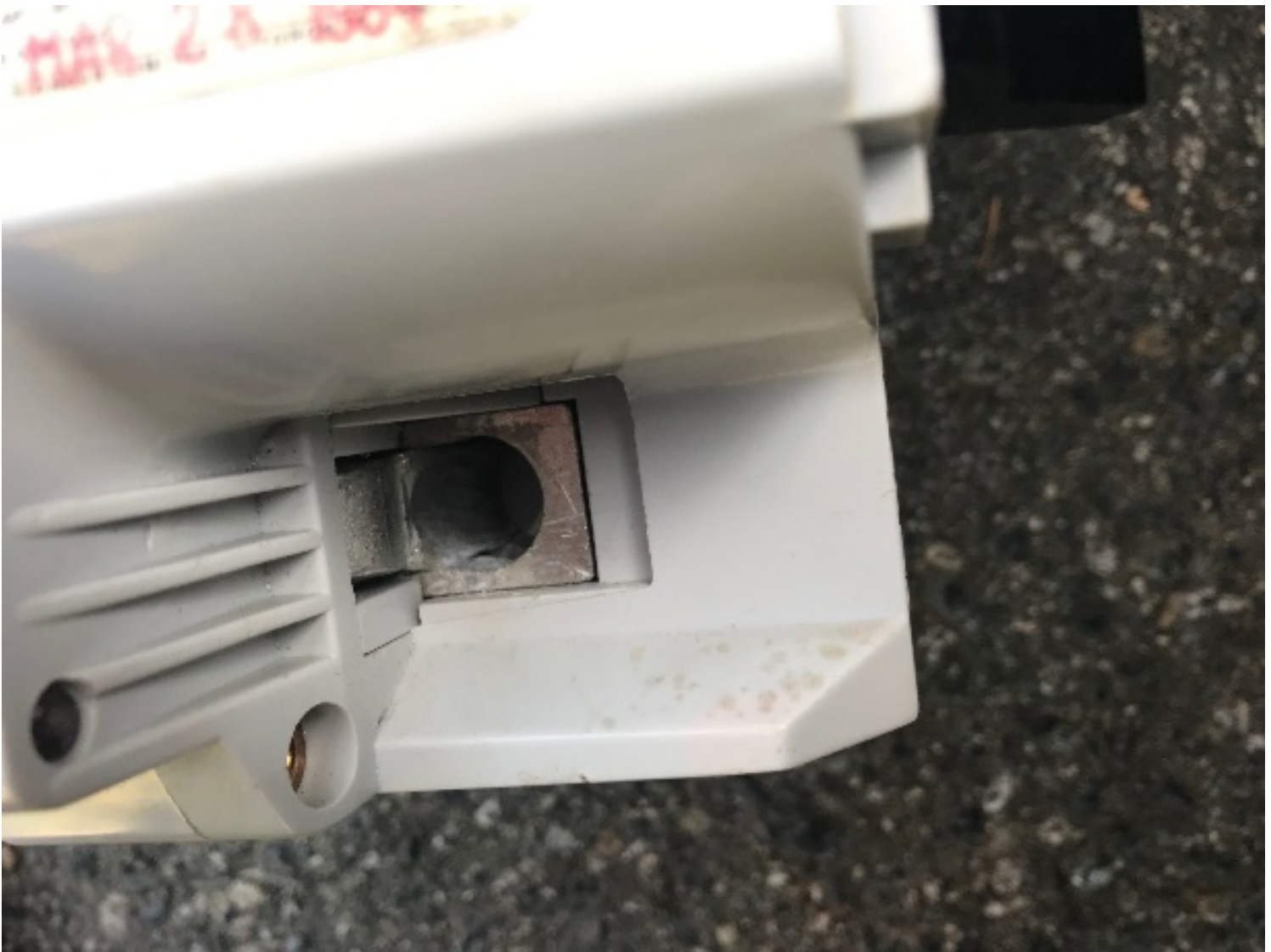
Photo 4: Breaker cable termination shows white powder
