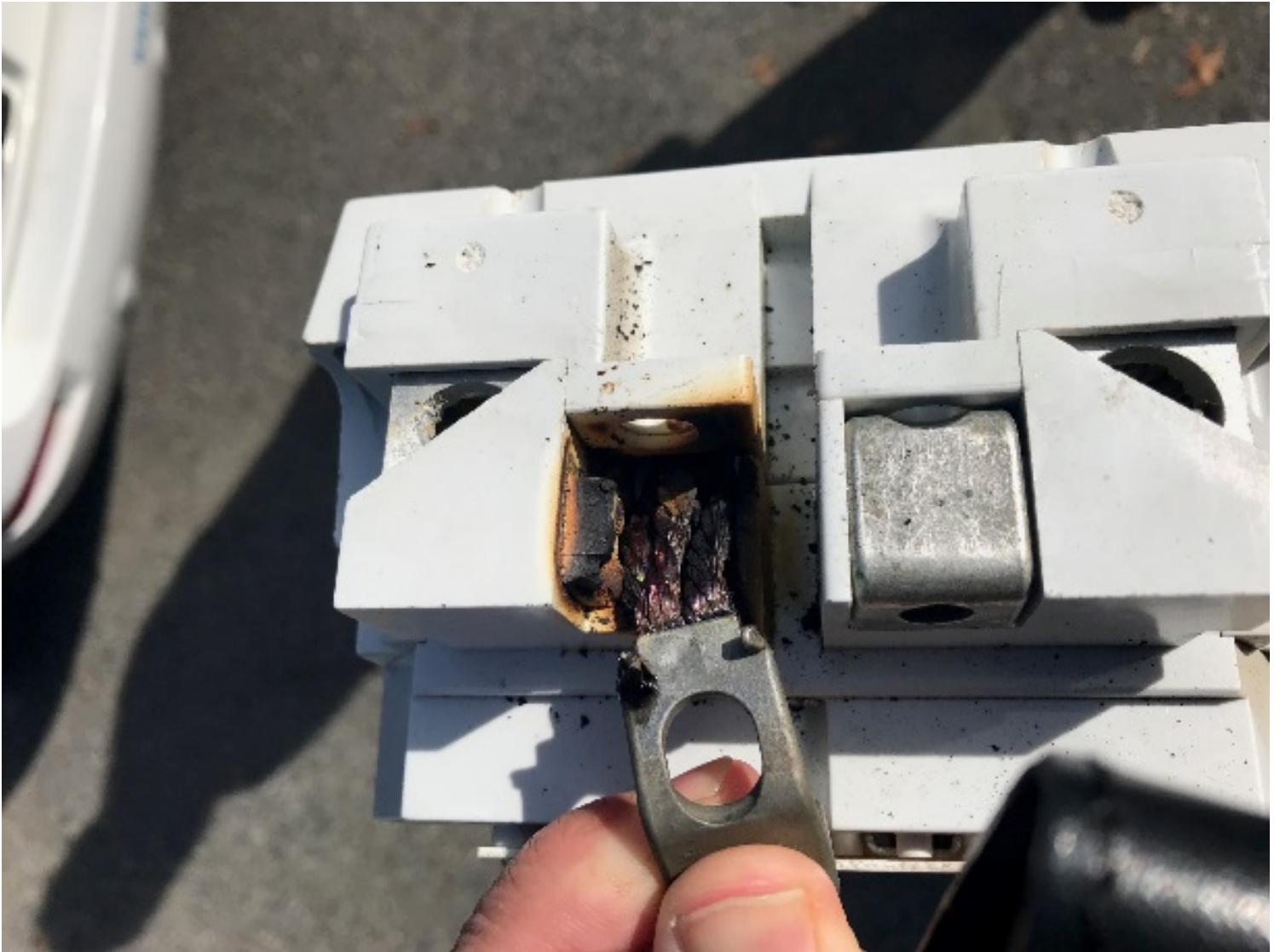
Photo 5: Breaker to buss contact melted apart
