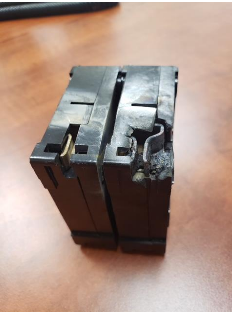
Photo 2: Burnt out breaker
