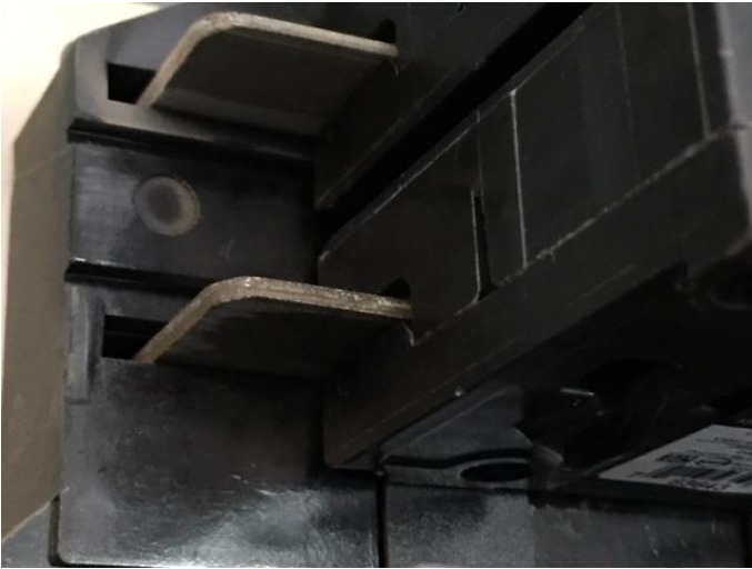
Photo 3: New breaker installed on refurbished buss work. Note slightly different colored buss material of lower component
