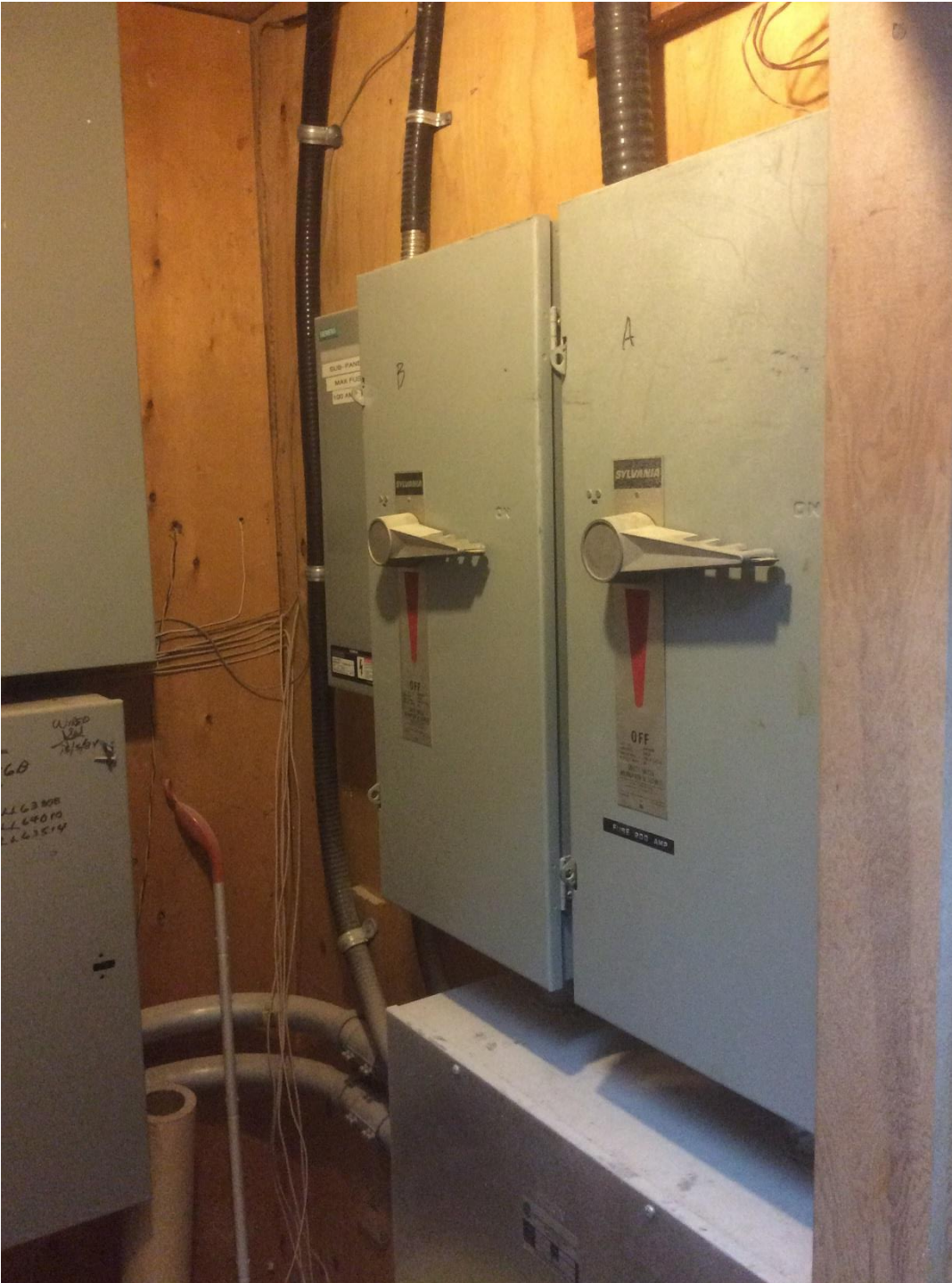
Photo #2 Main electrical room with sub-distribution feeder disconnects on right which feeds sub-panels on other side of this wall where electrical fire occurred.
