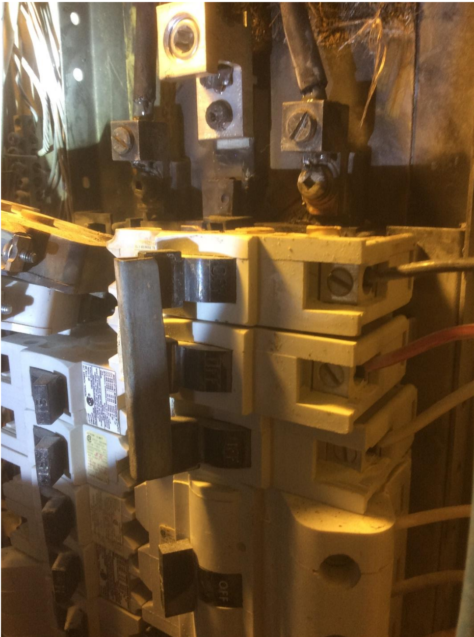
Photo #8 The previous existing terminal lug was removed and was replaced by electrician doing repairs as shown a shiny new terminal lug as compared to the other two burned and damaged terminal lugs.
