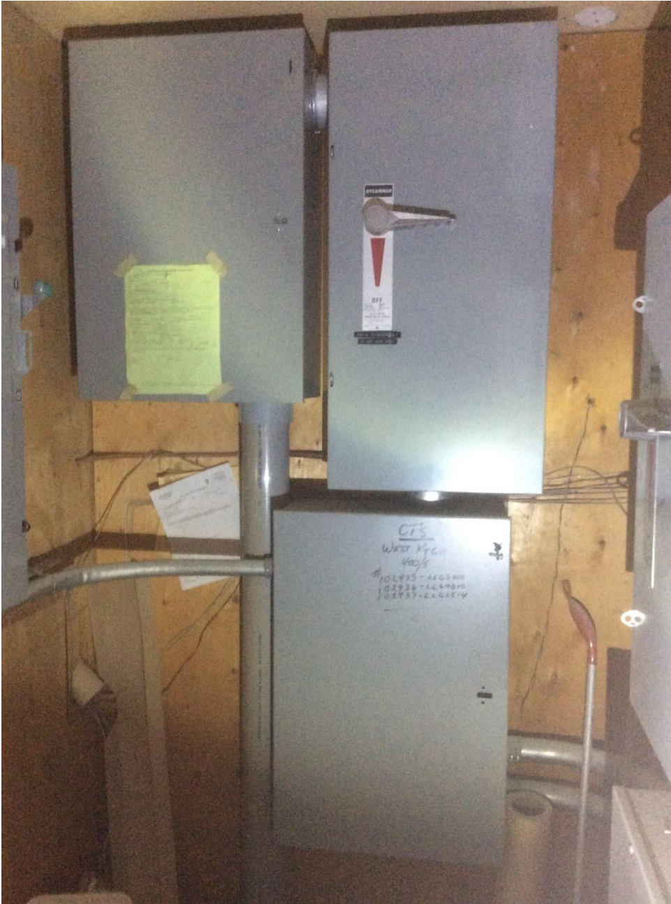
Photo #1 Main electrical room with 400amp 120/208 volt main service from utility hydro.
