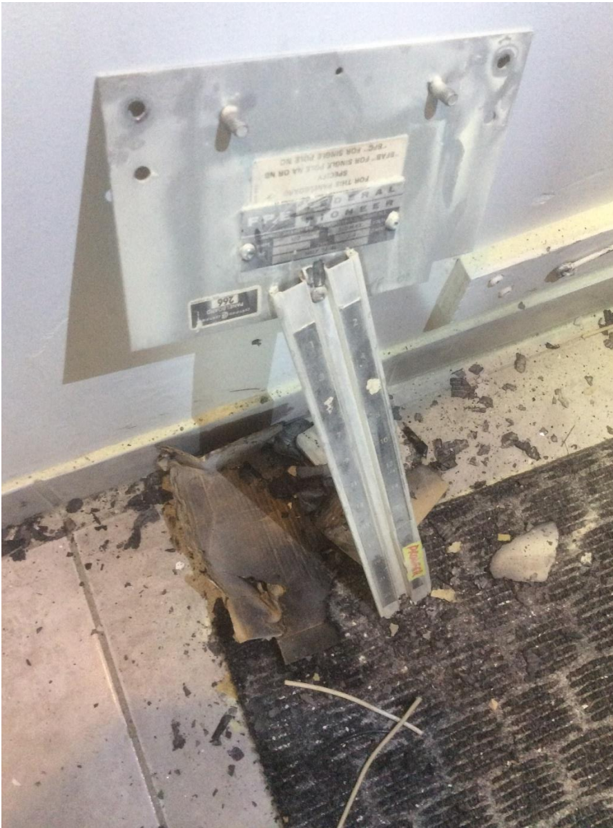
Photo #6 Remnants of the cardboard paper laying on the floor below panel board that electrician said was inserted beside terminal feeder lugs and paper caught fire near 3 phase terminal lugs
