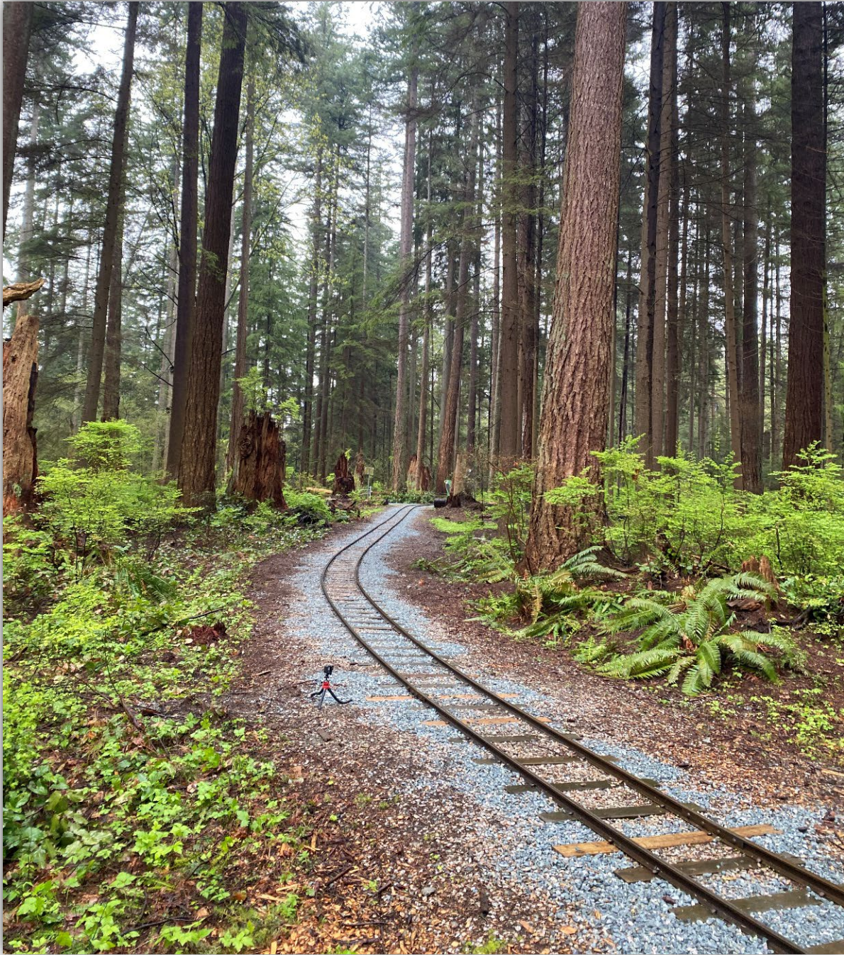
Image 4 – Area of track where the derailment occurred after repairs, realignment and releveling completed by rail contractor.
