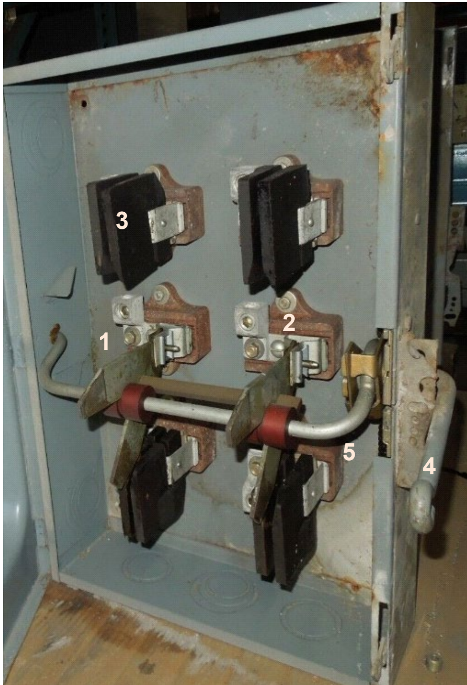
Image 3 – Similar style manual transfer switch.
