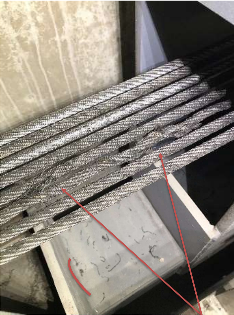
Premature worn rope with broken strands
