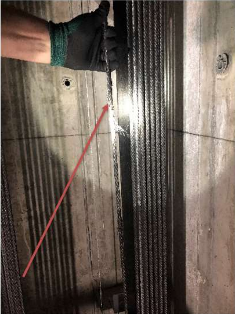
Premature worn rope
