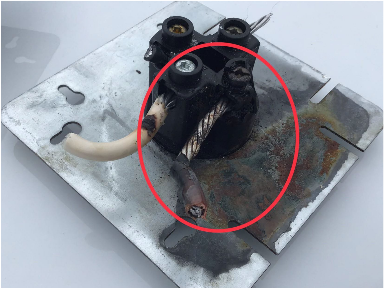
Image 1 - Line termination point where loose connection was found.
