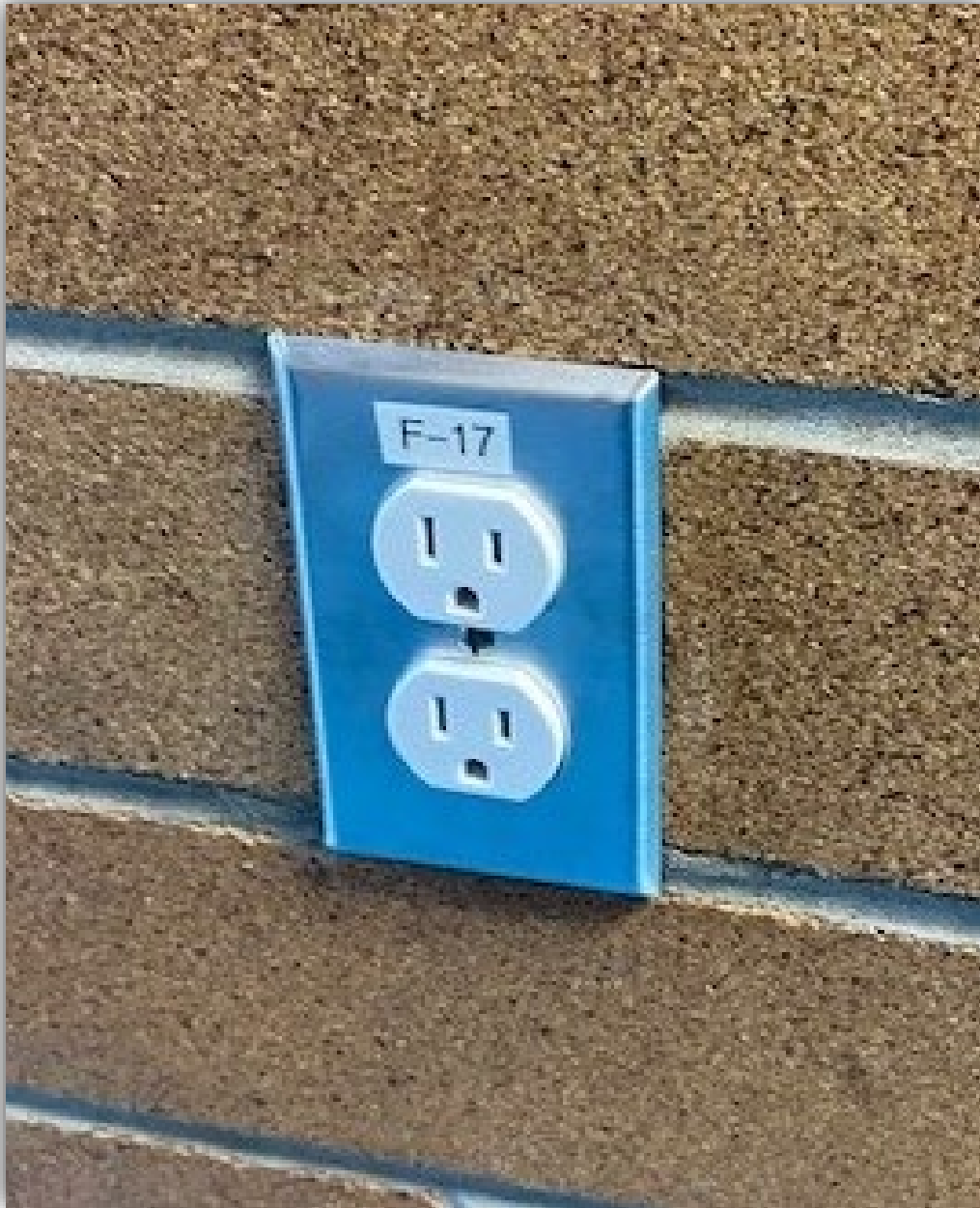
Image 2 - Location of install of original outlet. Replaced with Tamper Proof receptacle as observed in photo.
