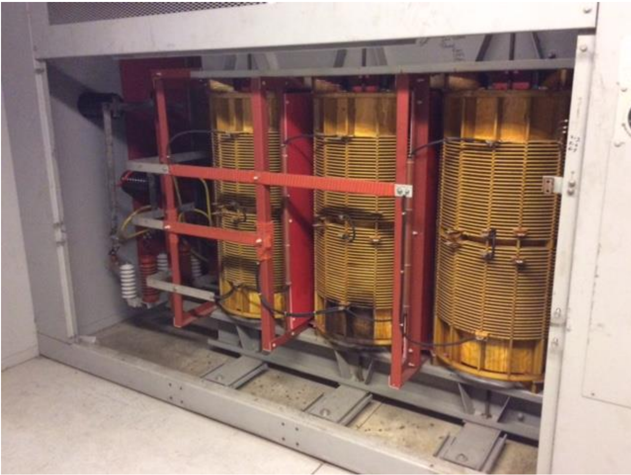
Failed transformer core.
