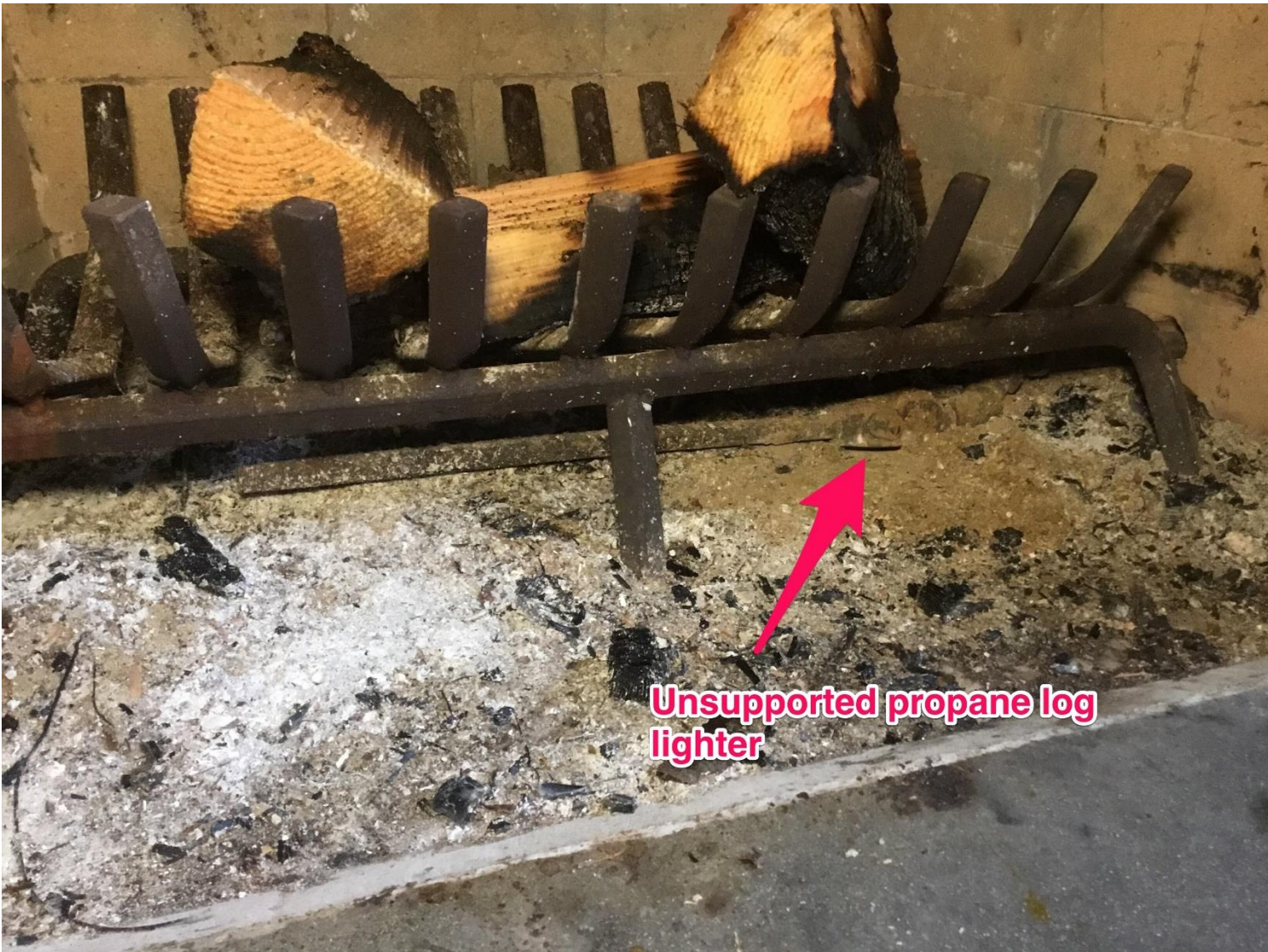
Picture #2 Unsupported propane log lighter
