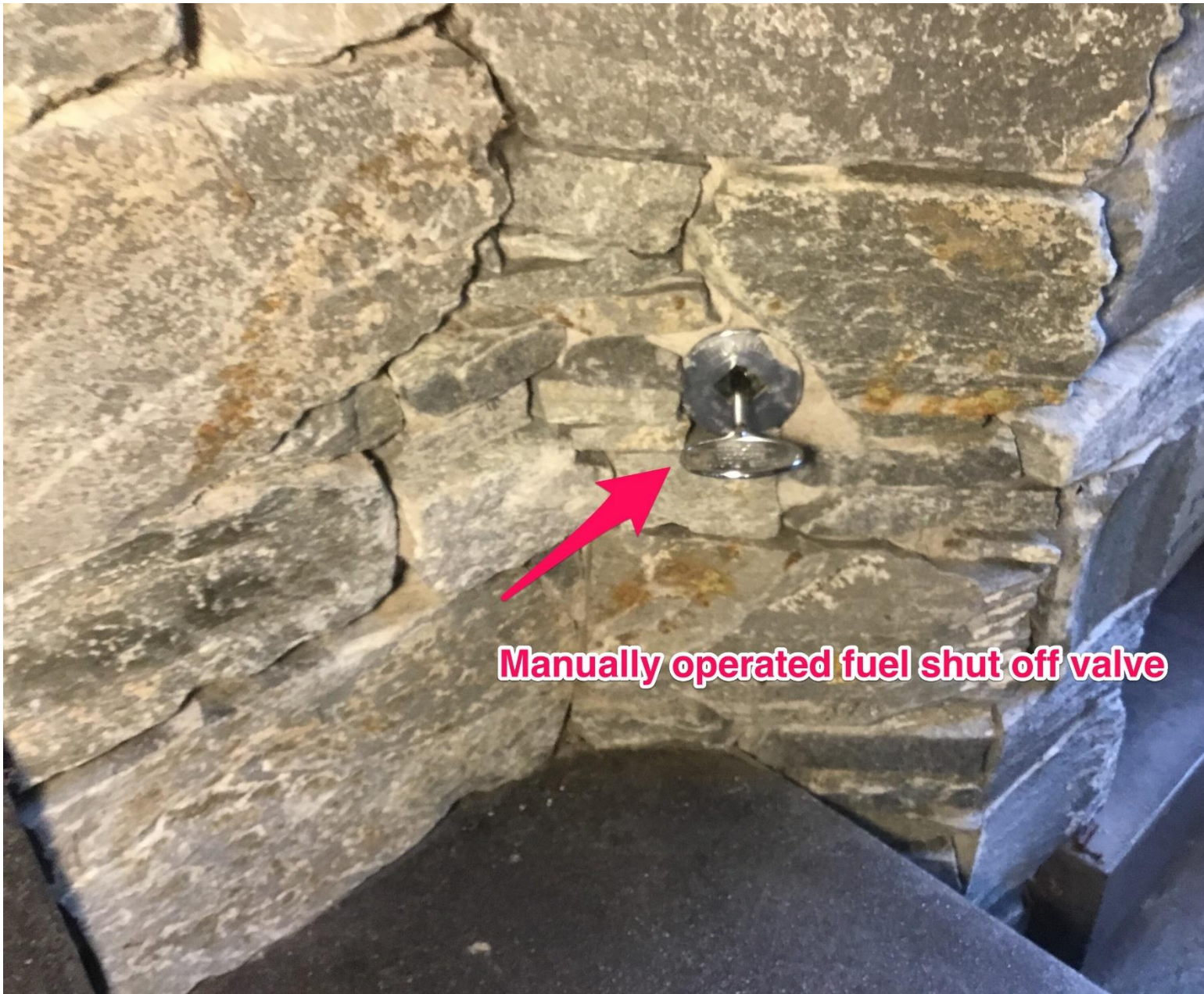
Picture #1 manually operated fuel shut off valve
