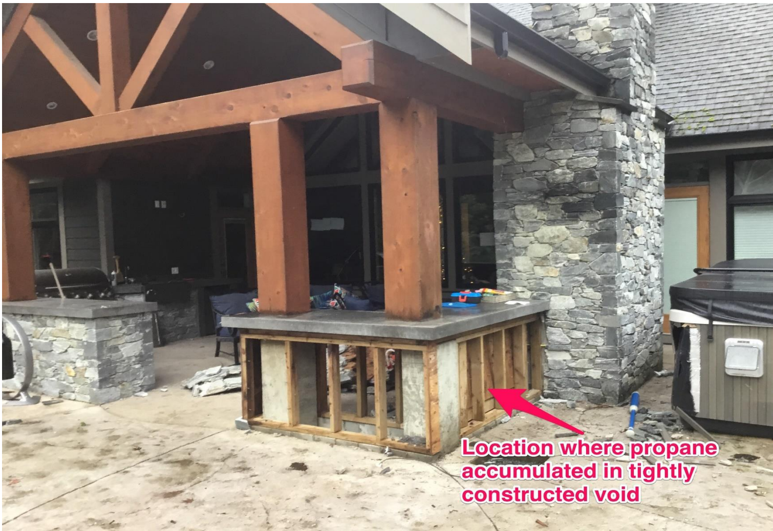
Picture #4 Where propane accumulated in tightly constructed void
