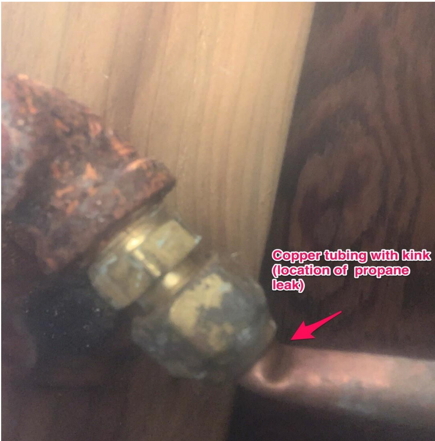
Picture #3- Copper tubing with kink (location of propane leak)
