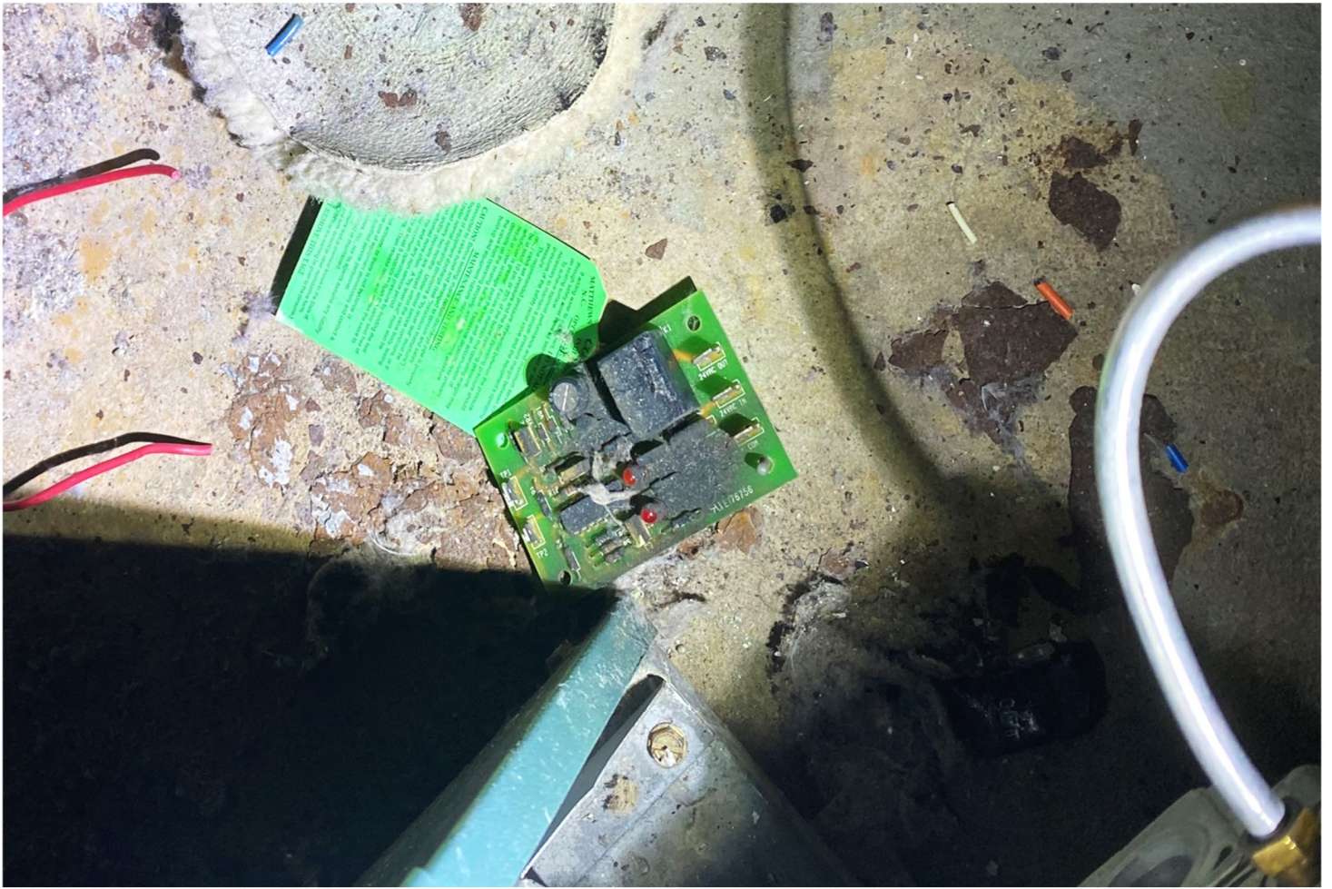
Photo 2 - The rapid thermal drop-out sensor was found laying on the floor beside the boiler.
