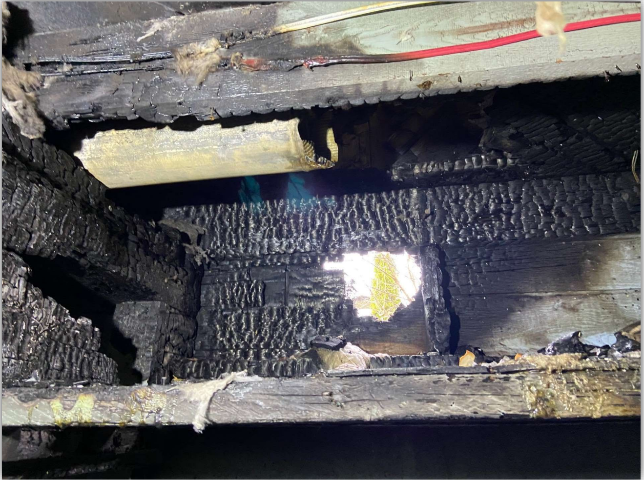
Image 3 - Shelving in the basement under the bedroom, the shelving contained plastic bottles.
