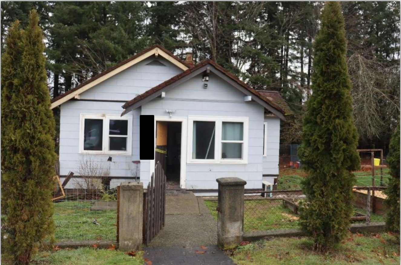
Image 1 - Front of house, fire started in the bedroom to the left of the main entrance.
