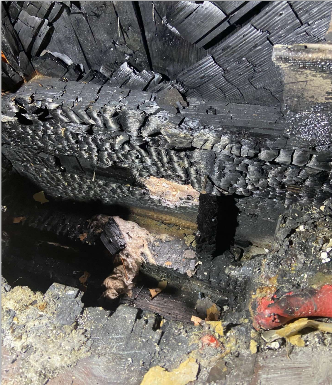
Image 4 - Looking from bedroom through hole in floor to the basement.
