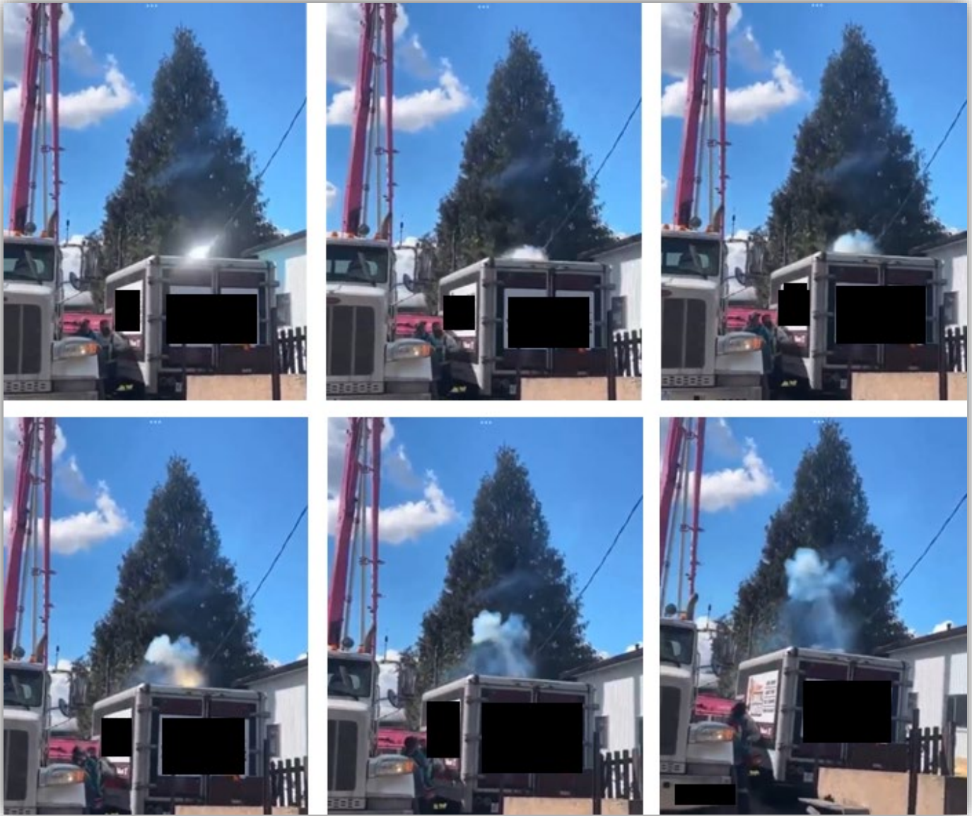
Image 5 – Screenshots of smoking and sparking utility lines from a phone video taken by a site worker.
