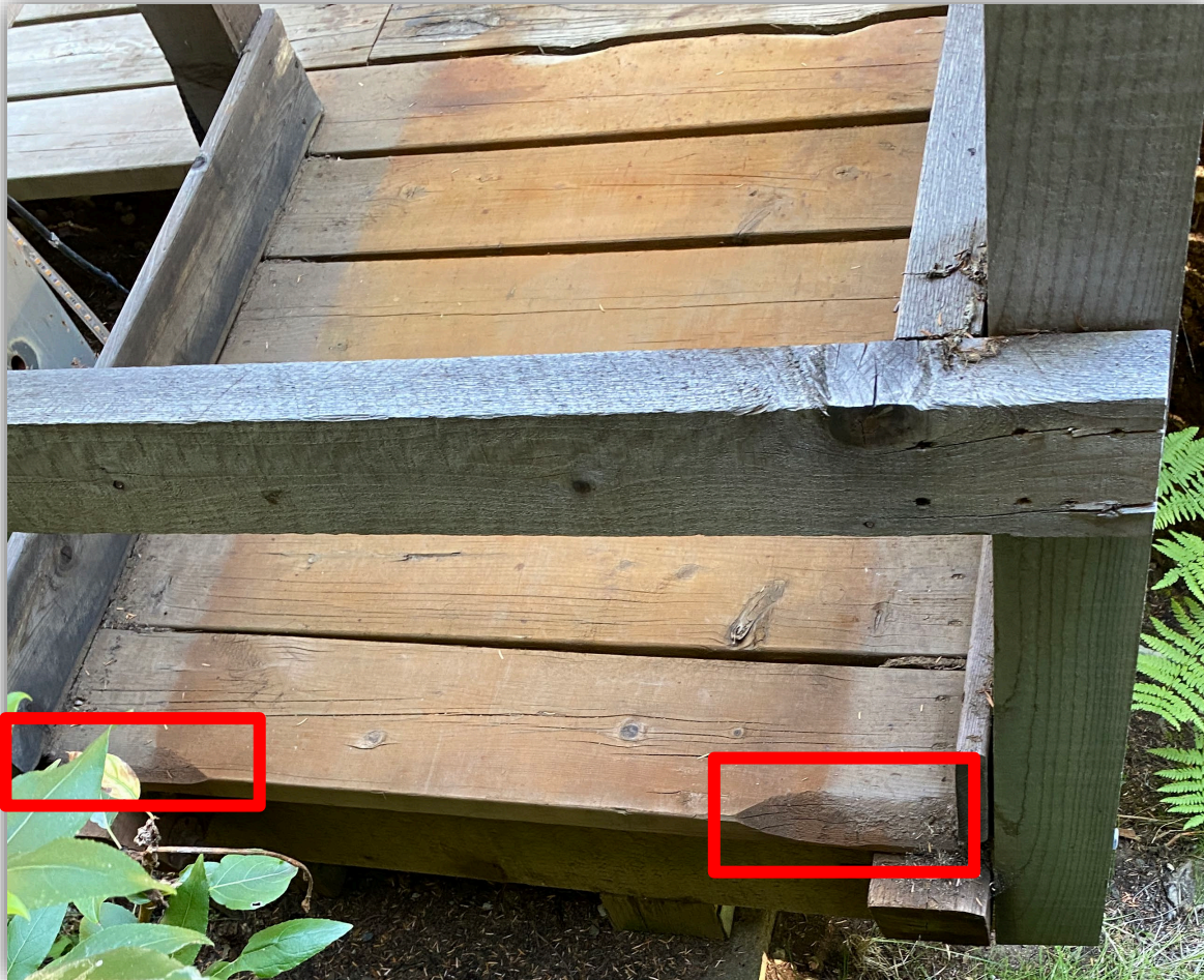
Image 7 – Staircase storage location with beveled edges [RED] for capturing staircase wheels.
