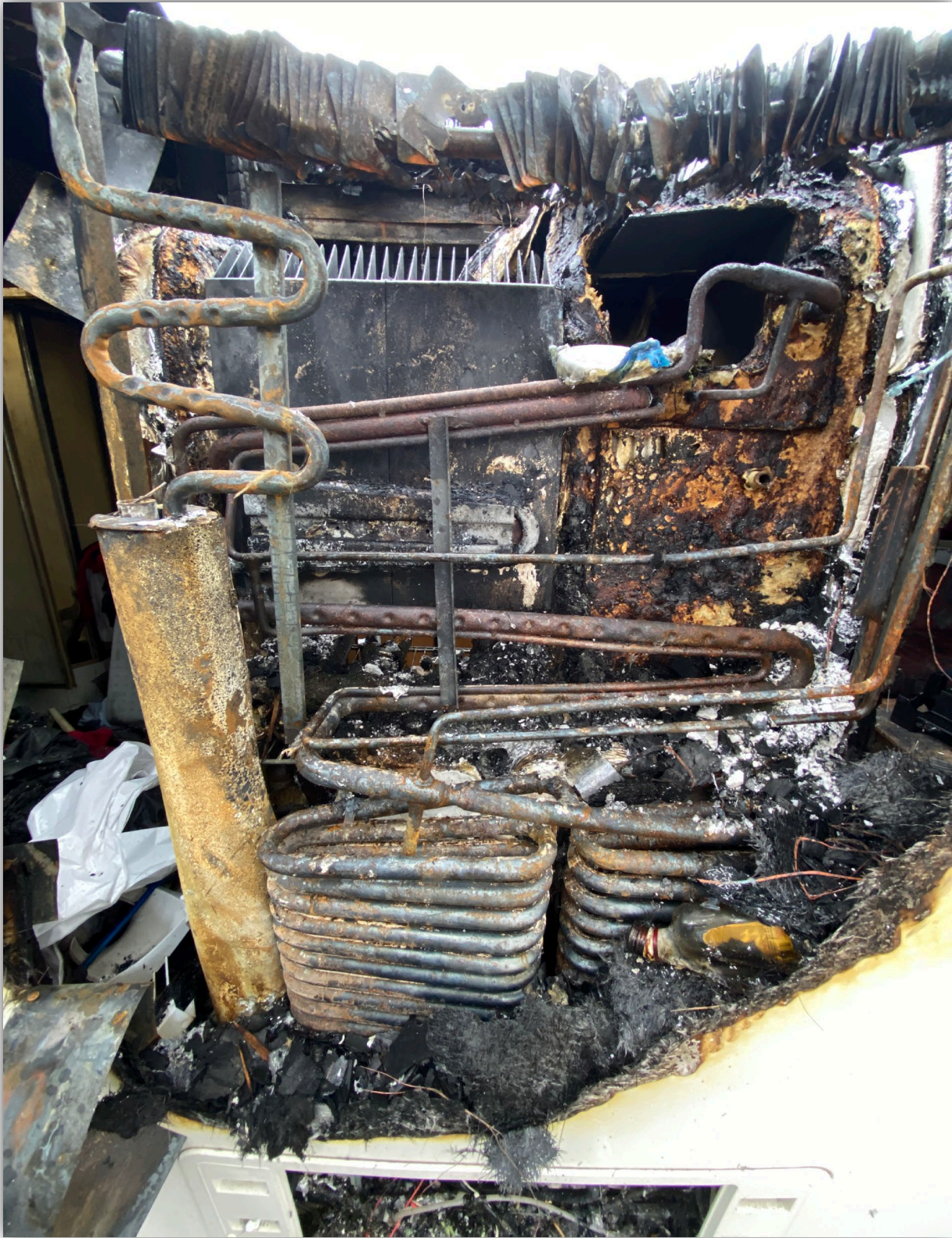
Image 3 - Rear of the fridge at time of investigation.
