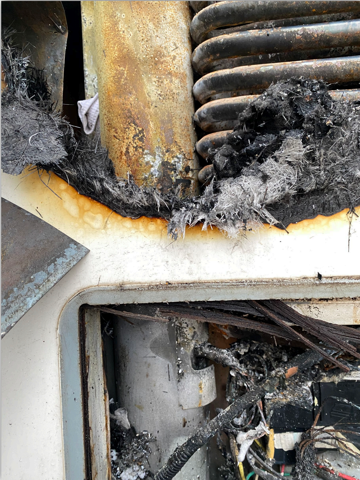
Image 4 - The combustion chamber of the fridge. Note the difference in the colors of the metal due to flame exposure. Flame patterns indicate a "V" style burn with the base of the "V" indicating the origin of the fire.
