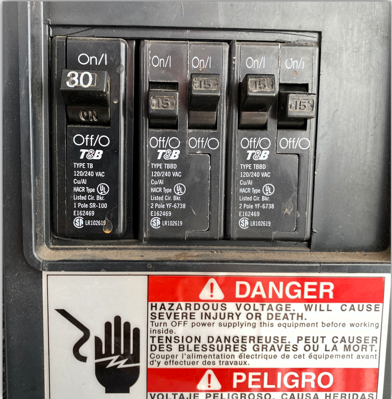
Image 8 - Breaker panel showing first, and fourth 15-amp breakers tripped.
