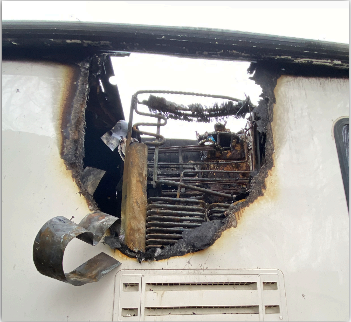
Image 2 - Exterior of the RV where the fire occurred.
