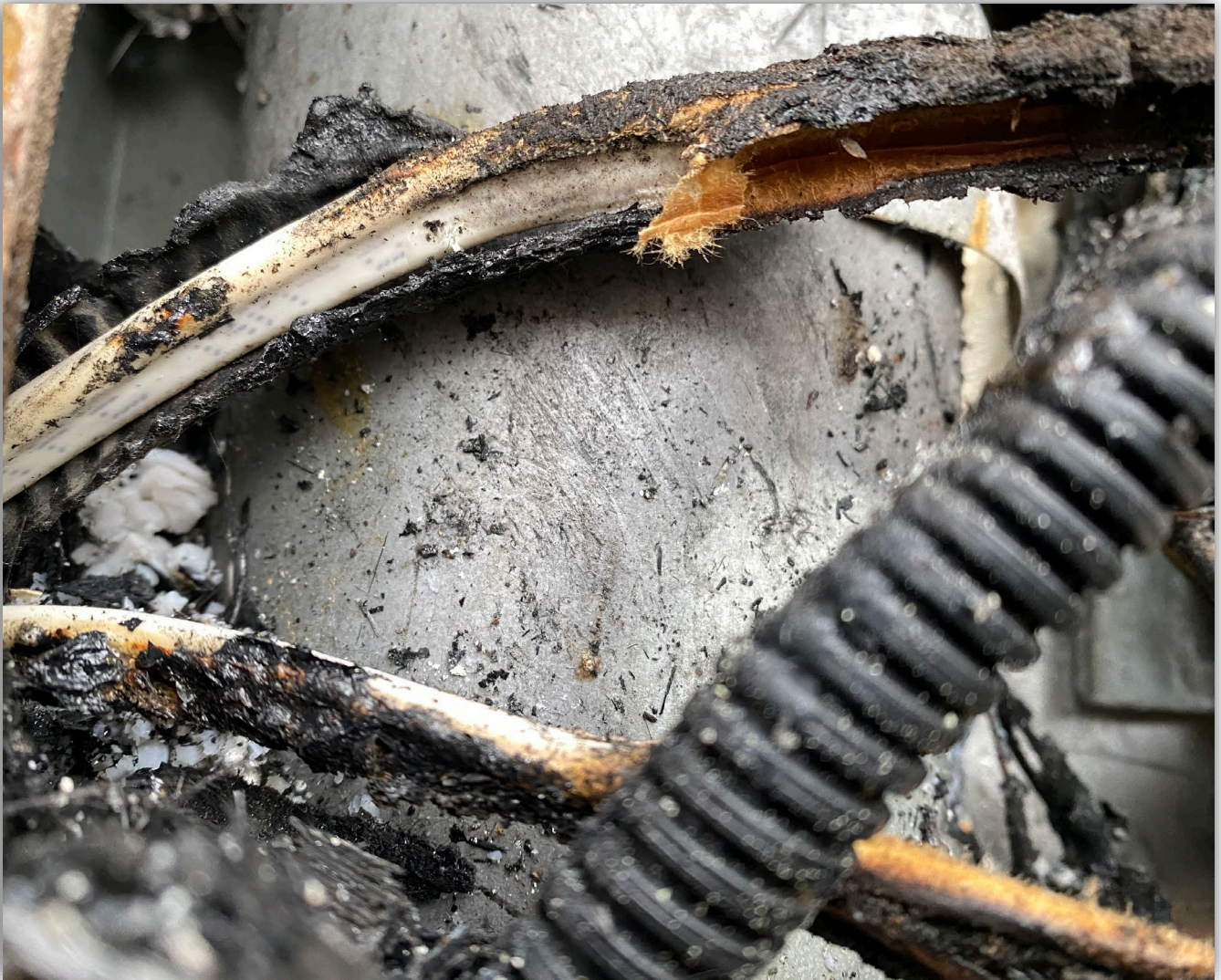
Image 7 - Exposed insulation of wire that was found to be in contact with the combustion chamber, showing that it was not low voltage wire in contact with the combustion chamber. This shows that the electrical potential would have been enough to cause the hole in the combustion chamber.
