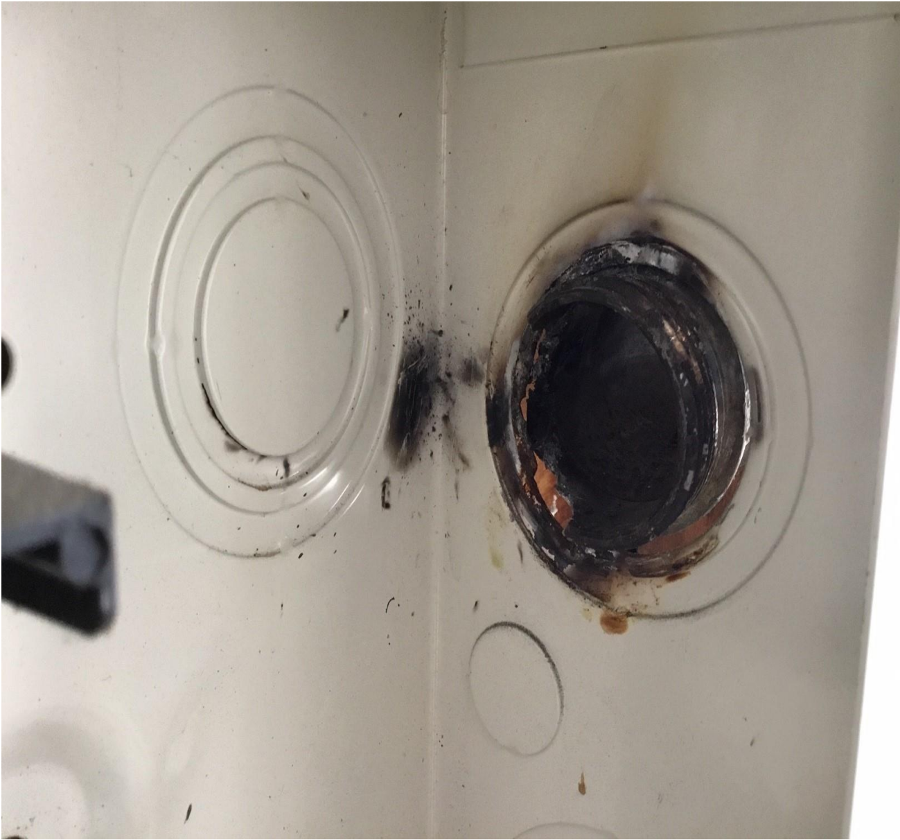
Picture #3 – Picture of the damage to the electrical metallic tubing connector after the conductors and lock nut were removed.
