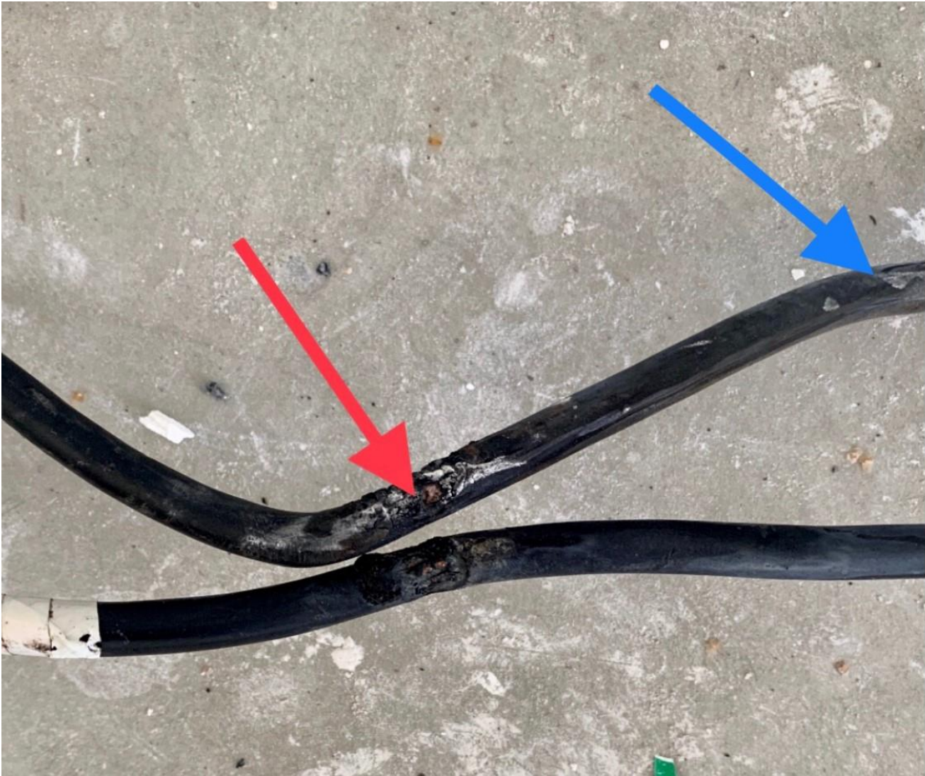
Picture #2 – Picture of the conductors after they were removed for the installation. Red arrow indicates the damage to the insulation of the ungrounded conductor where the fault occurred and the blue arrow is indicating other damage to the conductor's insulation.
