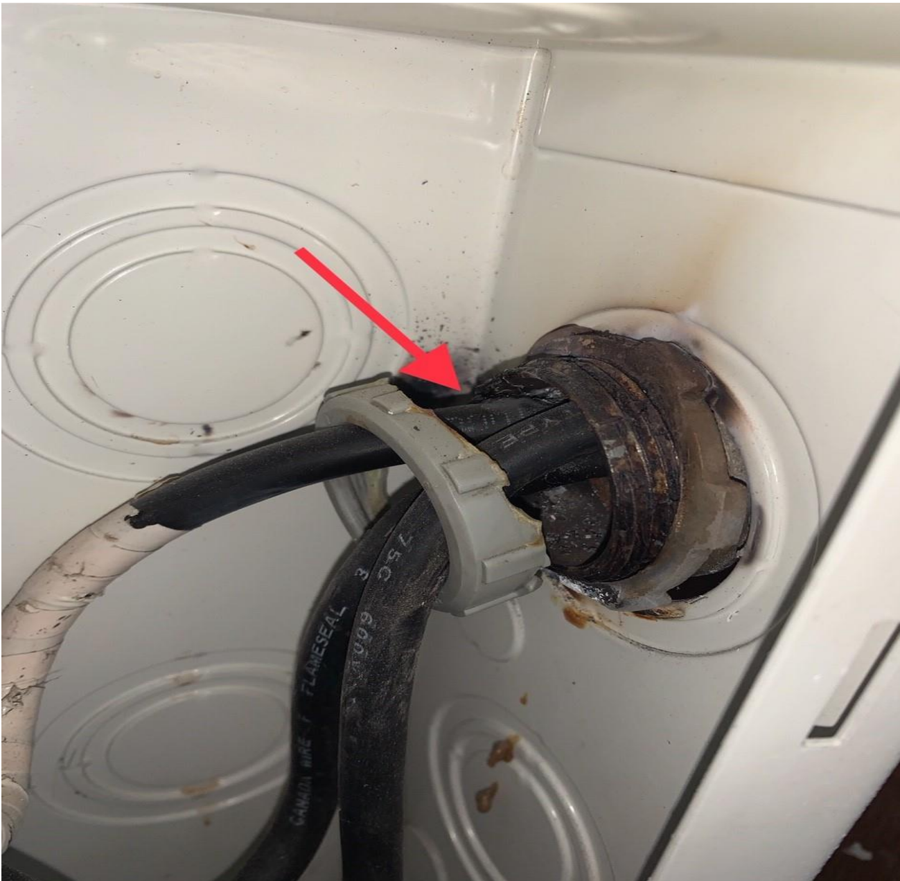
Picture #1 – Picture of when the service entrance section barrier was removed. Red arrow indicates where the damaged was to the ungrounded consumer service conductor shown in Picture #2 with a red arrow.
