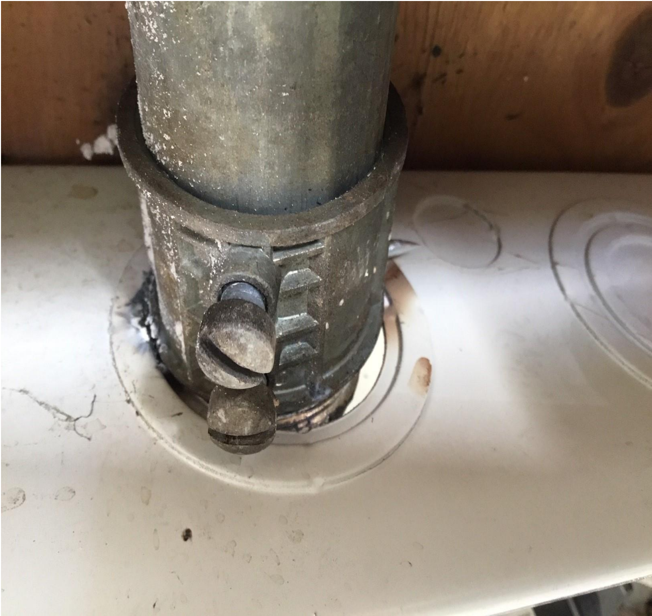
Picture #4 – Picture showing the knock out in the panelboard is oversized for the installed connector.
