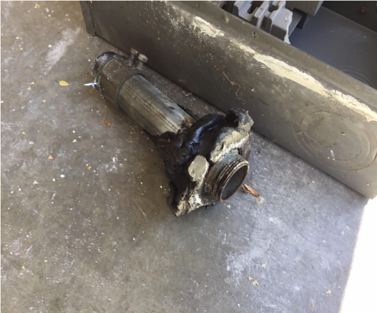
Picture #6 – Picture of the electrical metallic tubing raceway once it was removed showing the black sealant around the connector on the side that was entering into the meterbase.
