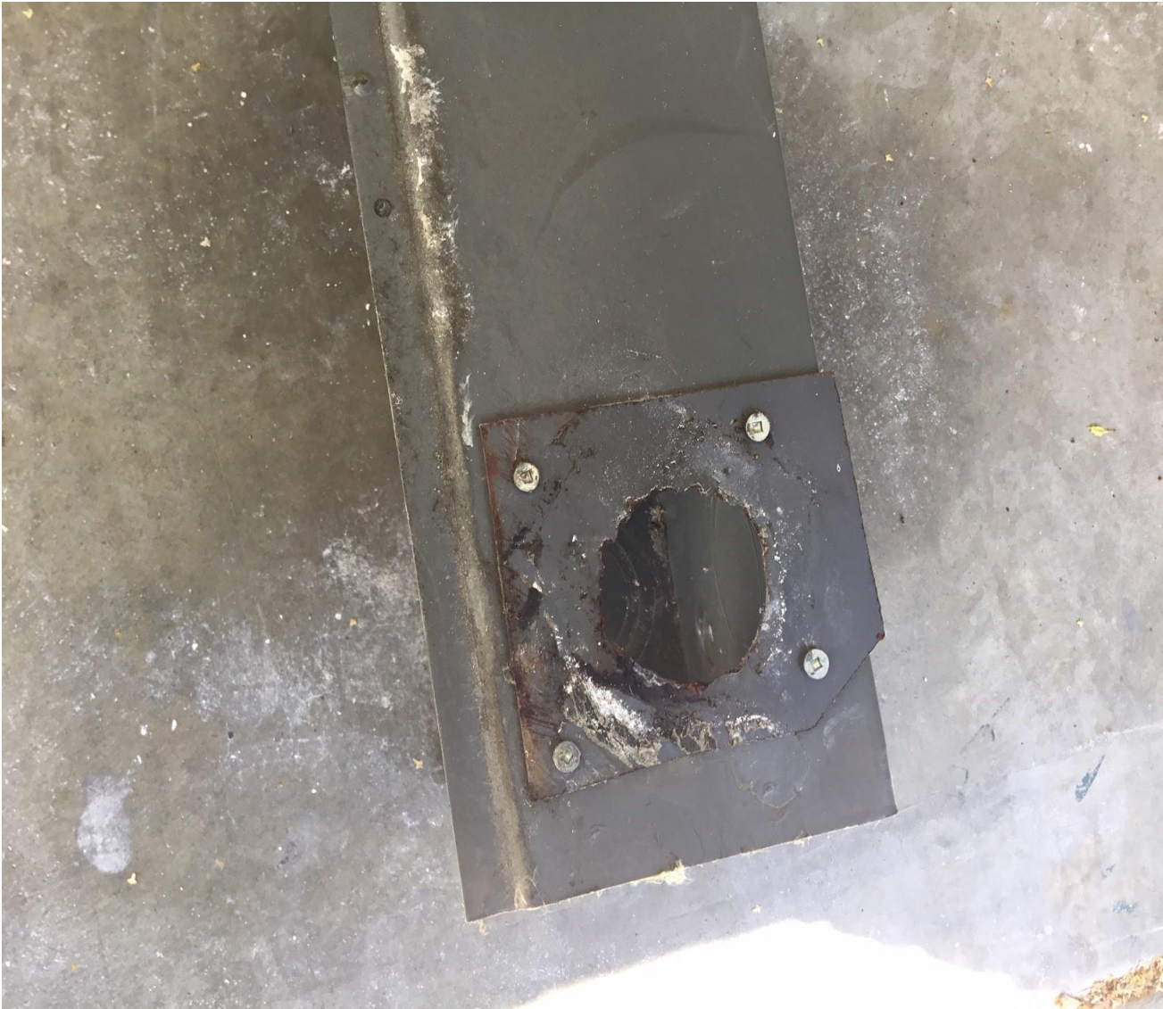
Picture #5 – Picture showing the alterations to the single meterbase.
