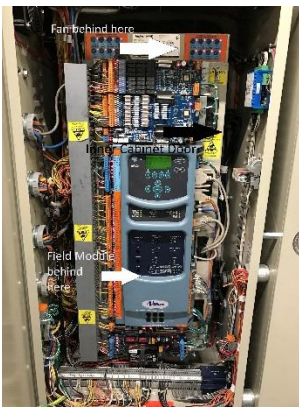
Photo 7: The elevator controller layout with the inner cabinet door closed
