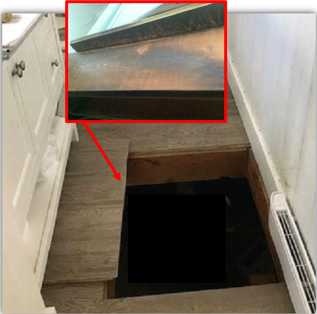
Photo 5 – Burn damage to crawl space entrance.
