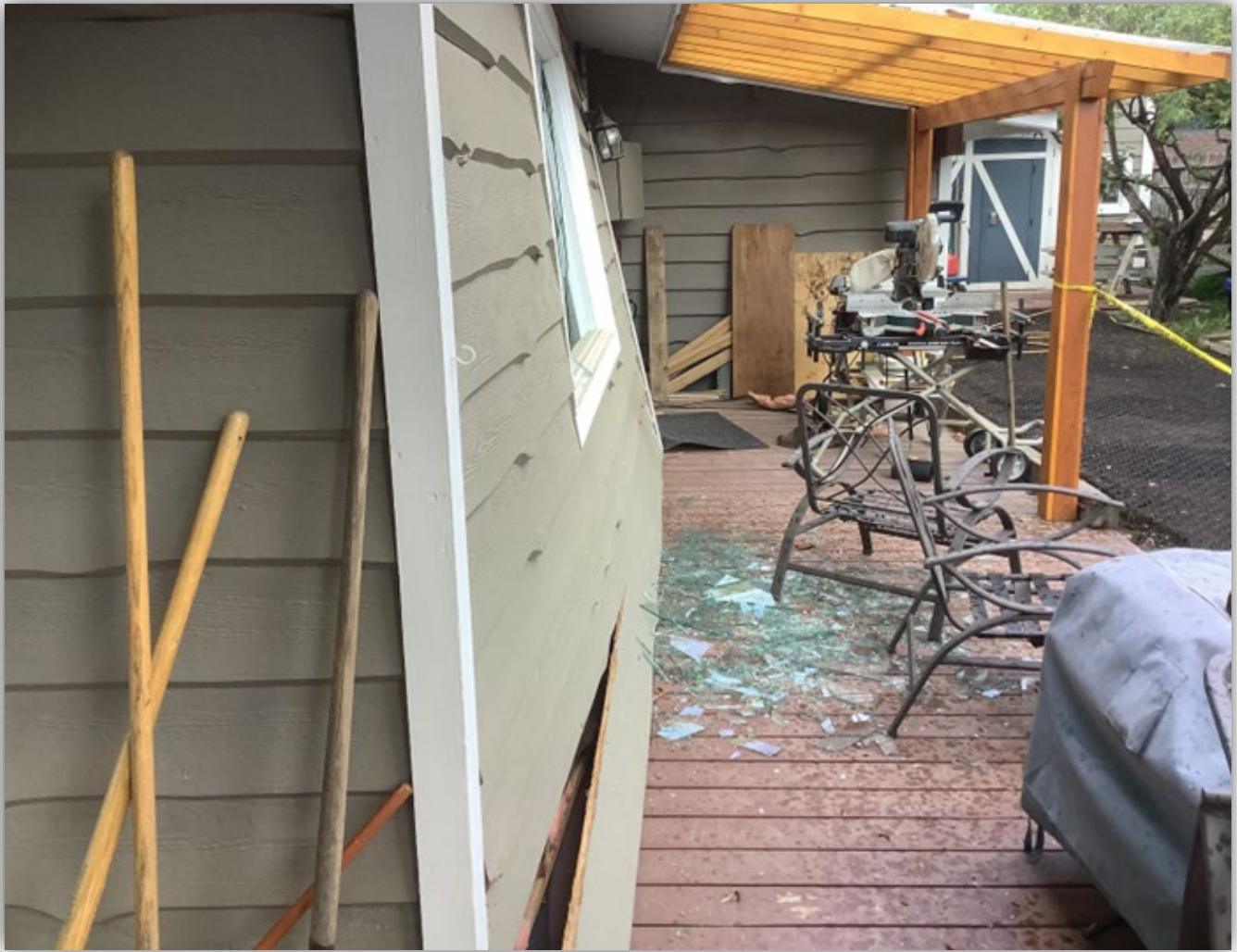
Photo 1 – Exterior wall of cabin blown out.
