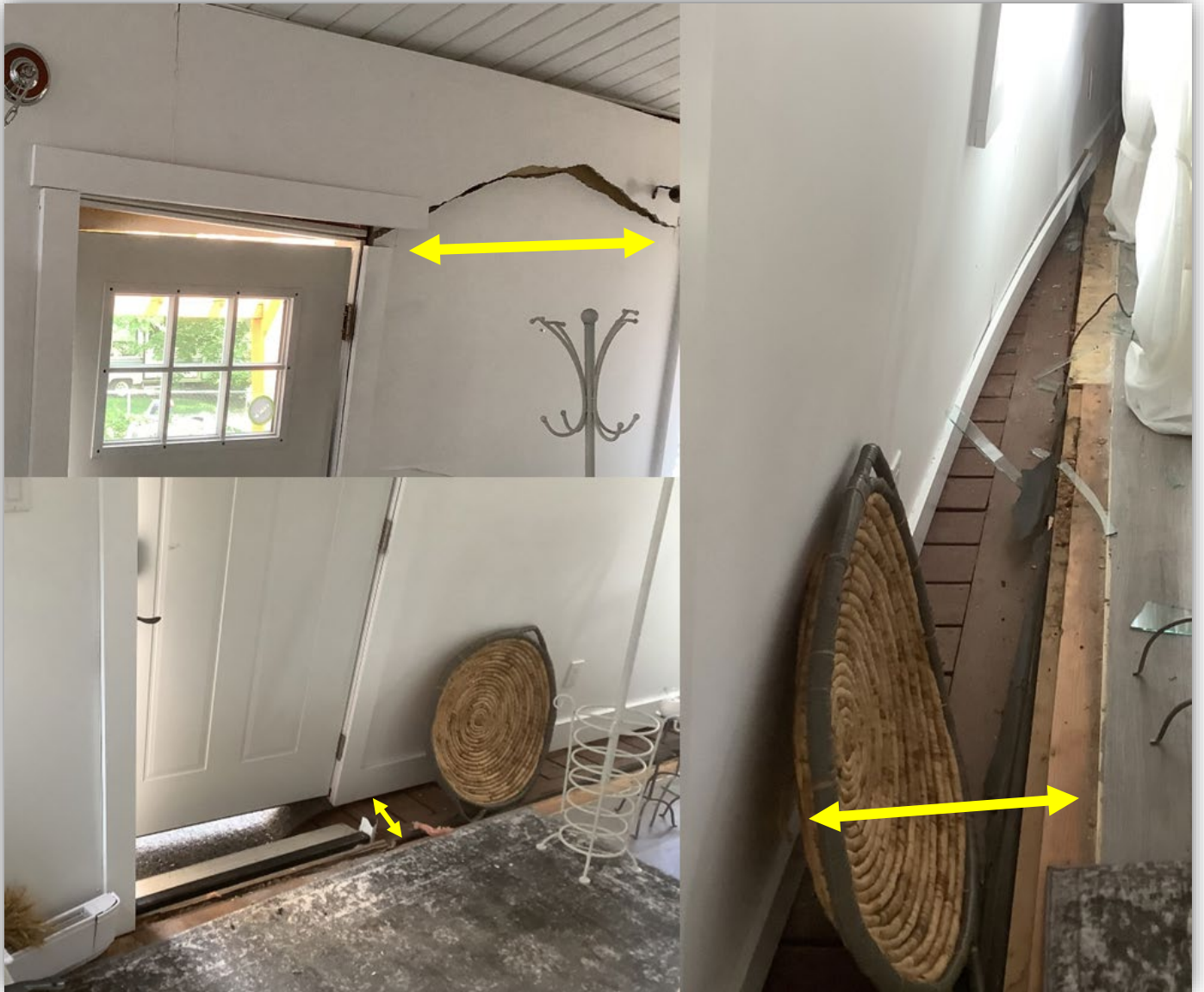
Photo 3 – Damage to wall.
