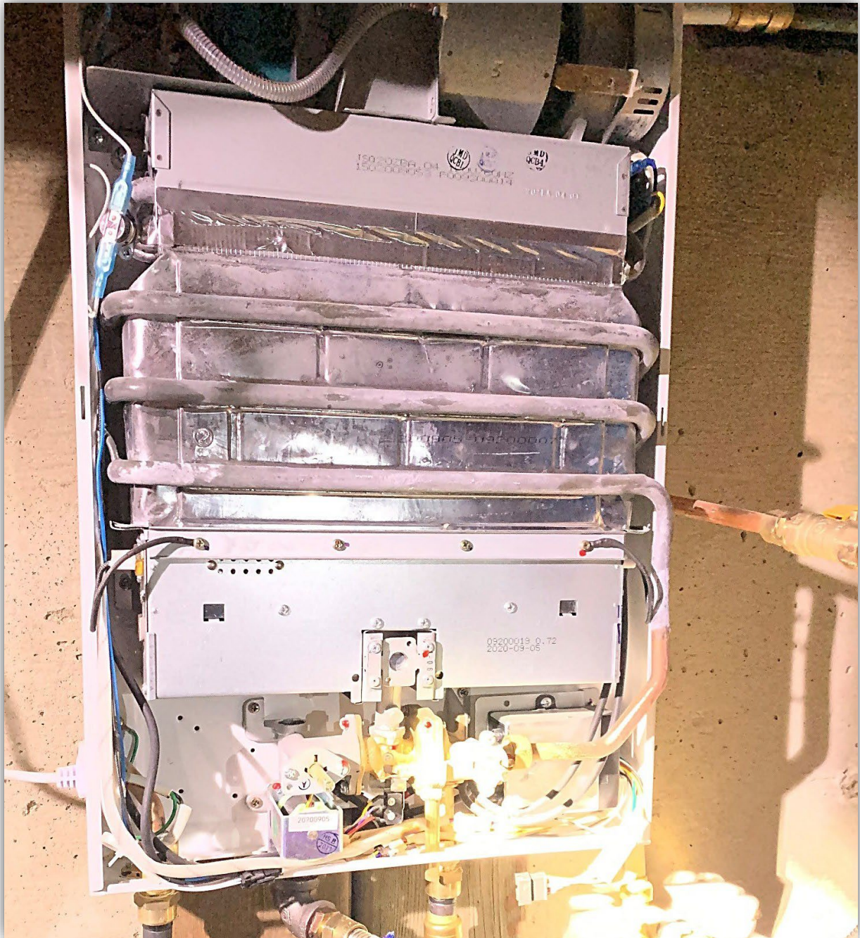
Photo 7 – On-demand water heater.
