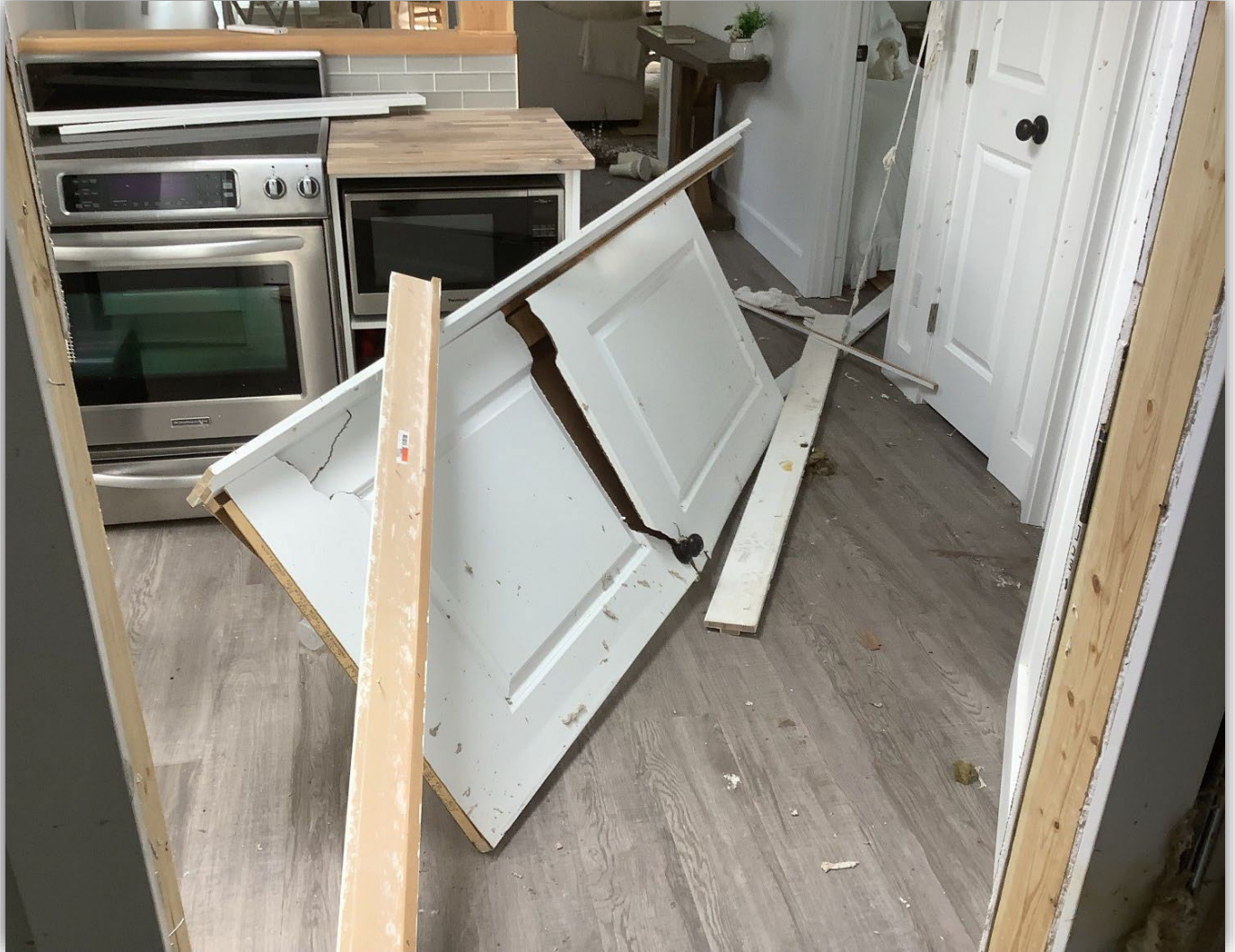
Photo 4 – Interior door blown out.
