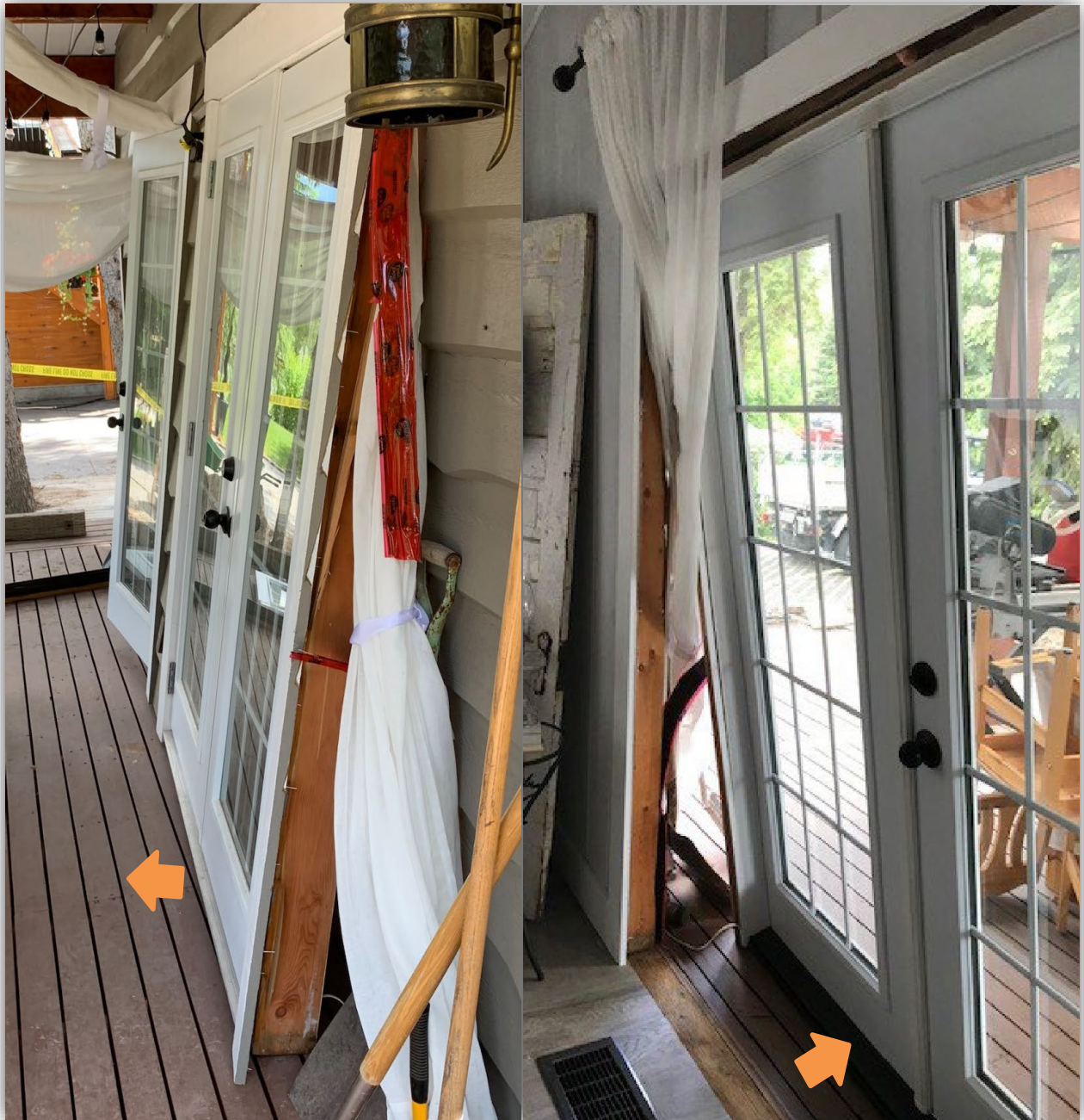
Photo 2 - Exterior doors blown out.
