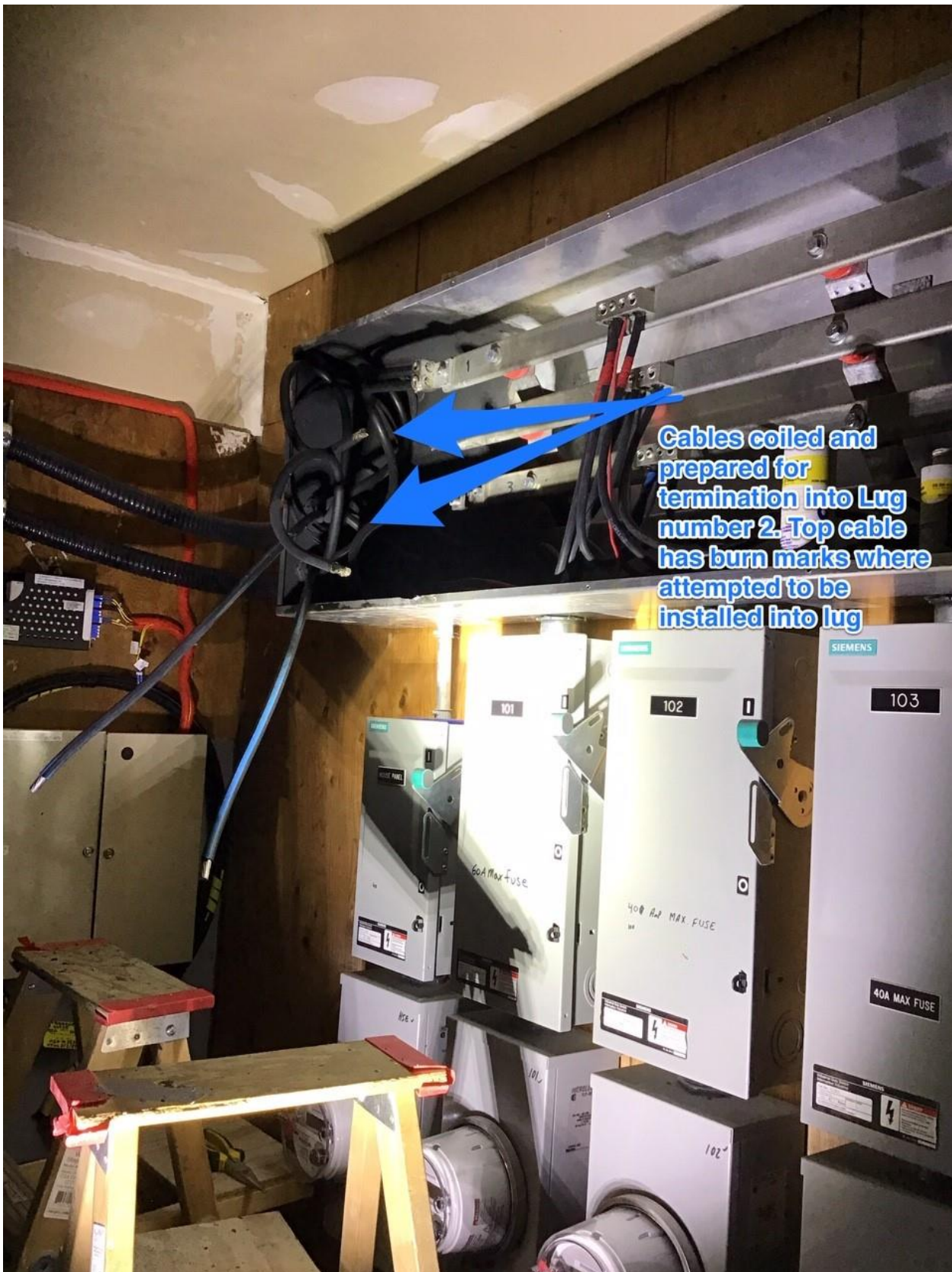
PHOTO 4: Line 2 Cables were cut, coiled and were attempted to be terminated into Lug #2.
