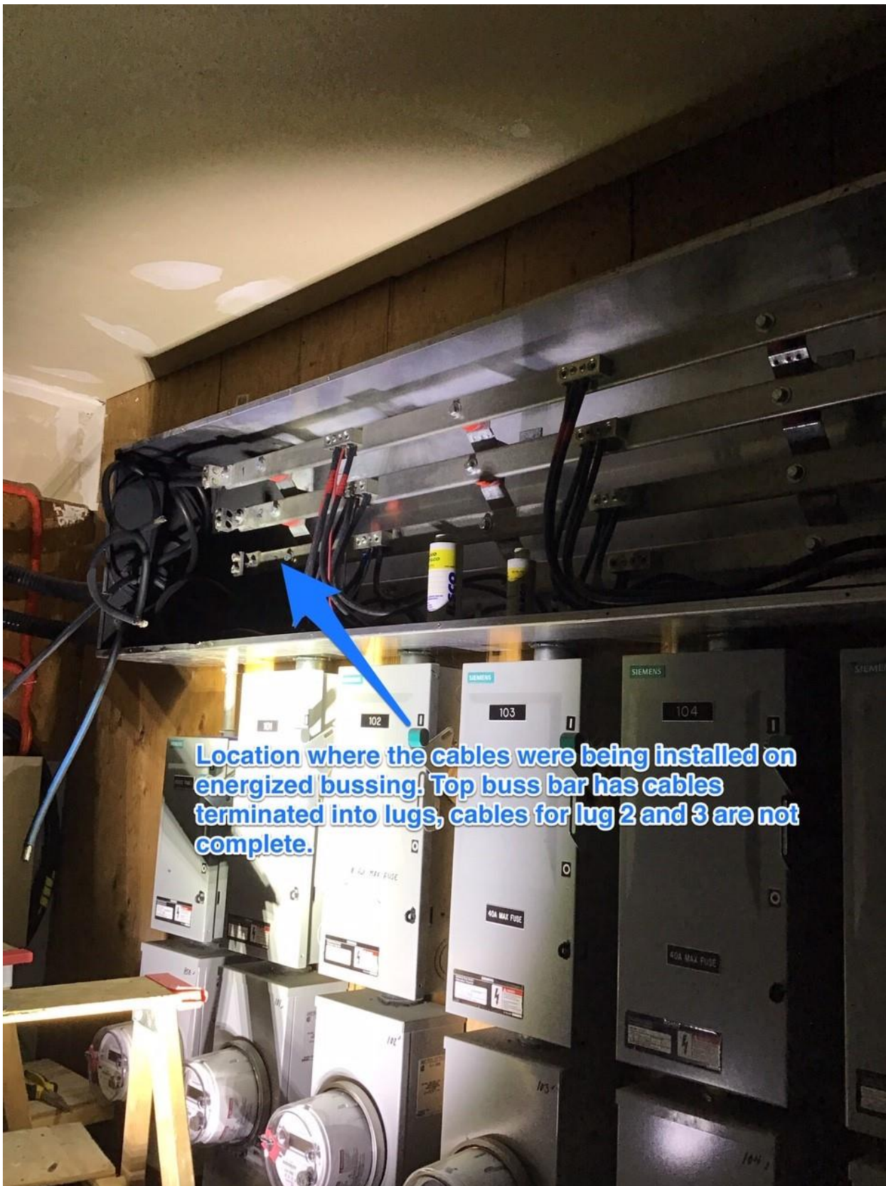
PHOTO 2: Junction box with energized bussing at time of incident, de-energized by the utility at time of photo.
