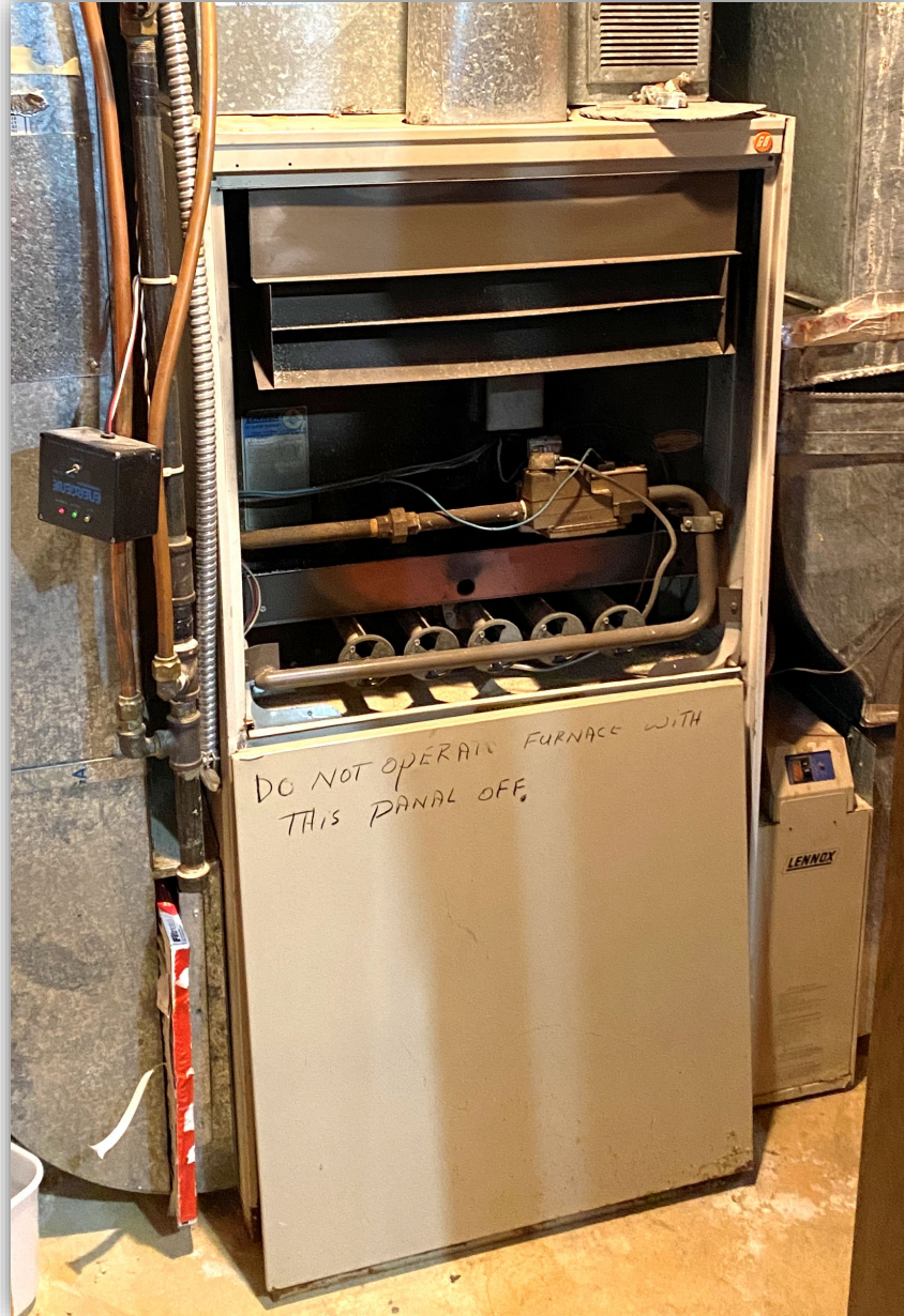
Photo 1 – The gas furnace in the mechanical room with the front cover removed.
