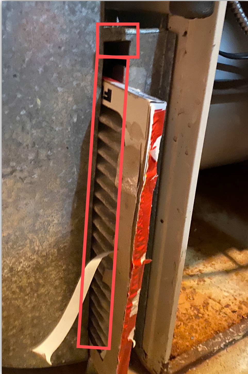
Photo 6 – Incorrect furnace filter installed. (RED) Opening gaps allowing air to be drawn into the blower from the mechanical room.
