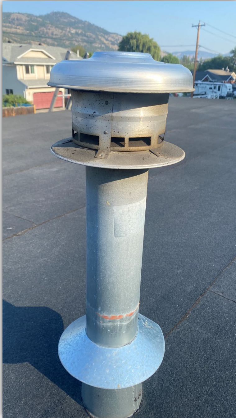
Image 7 – The b-vent termination for the dryer with the unsecured rain cap still attached after the explosion.
