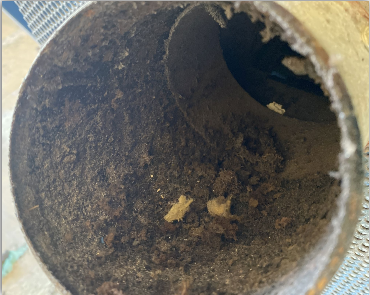
Image 4 – Inside of dryer exhaust vent showing dust, lint and debris from the operations process.
