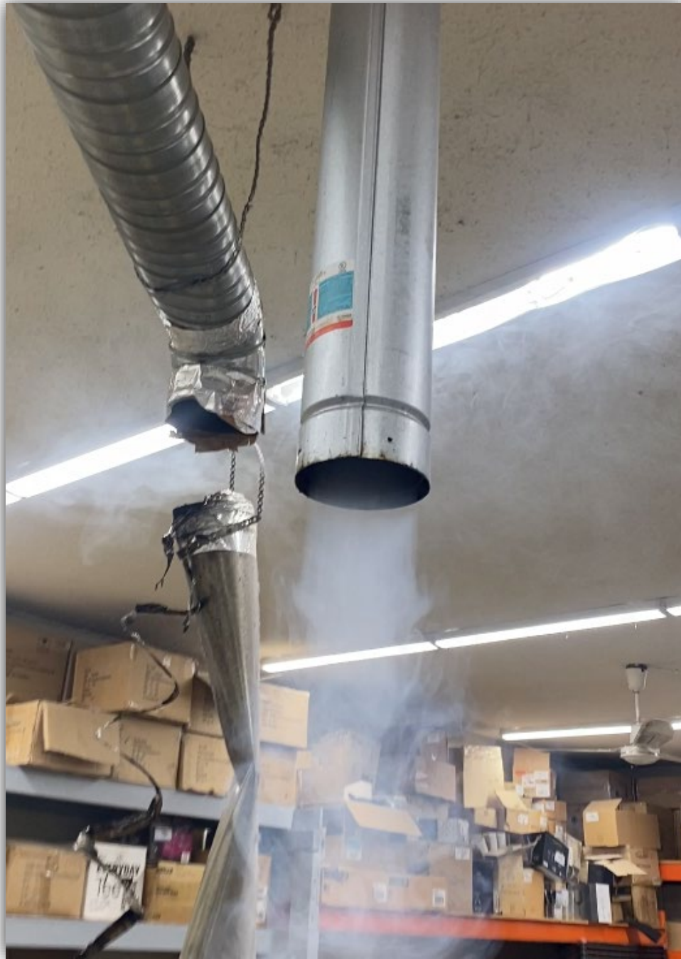
Image 8 – Smoke from a smoke stick test being drawn into the building from the roof through the disconnected dryer vent due to a negative pressure condition in the building created by one exhaust fan operating.
