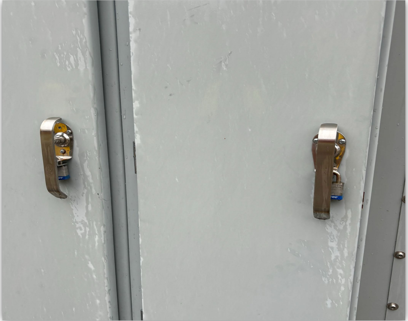
Image 5 – Substation – Public facing padlocks.
