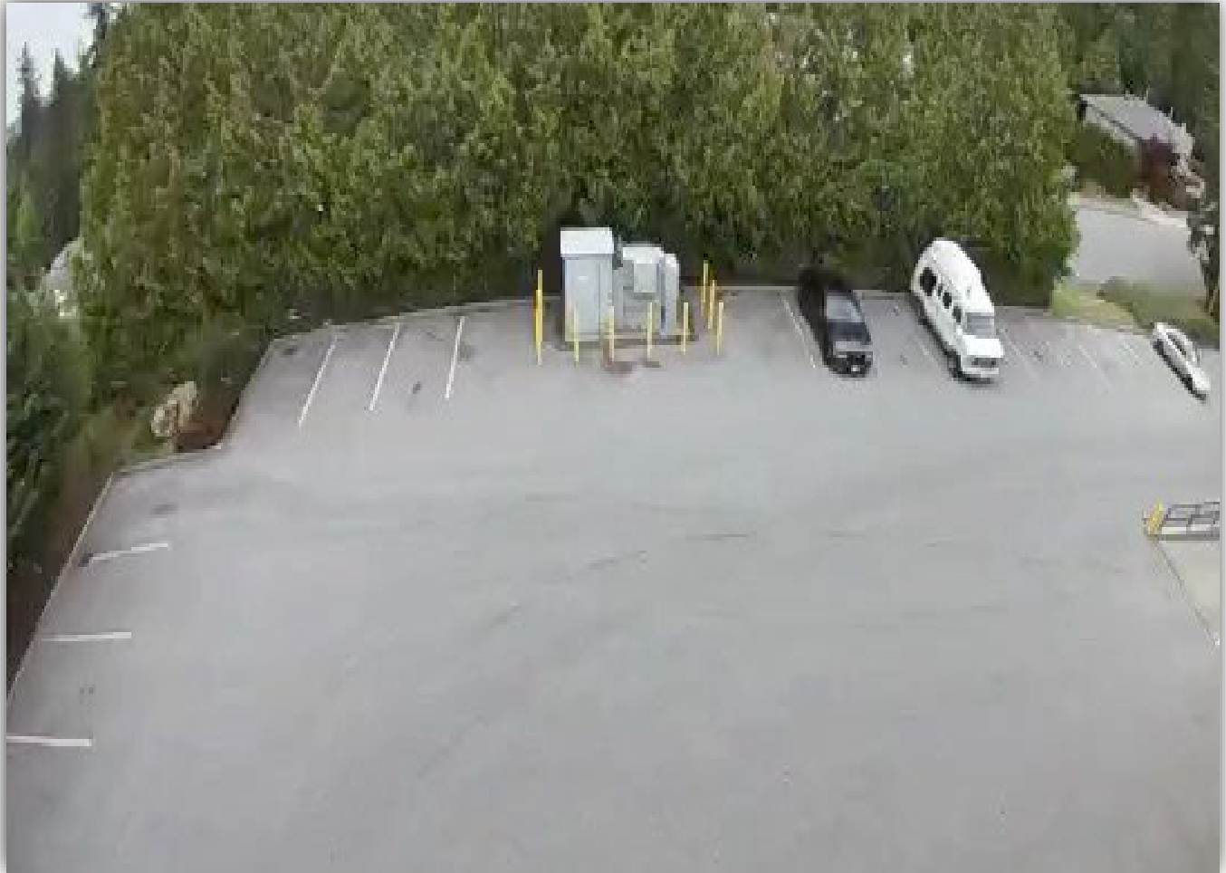
Image 1 – Substation within the parking lot. Tree area behind.
