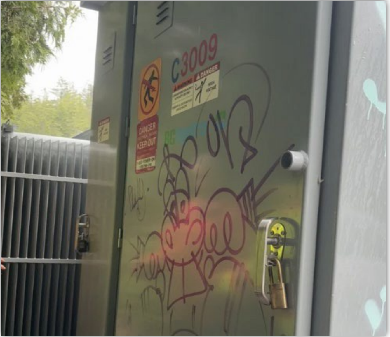
Image 4 – Substation - Rear doors facing into trees and shows vandalism. Also shows private and public locks that were replaced after incident where previous locks were removed and damaged.
