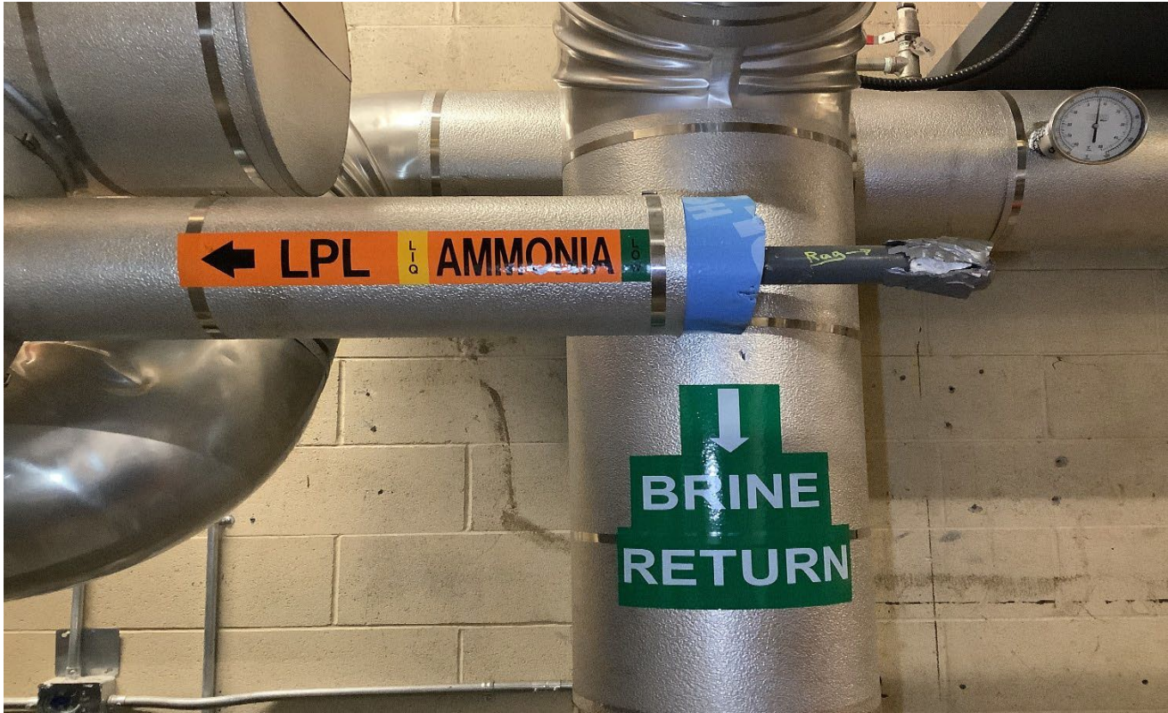
Image 1 - The pipe that was cut.
