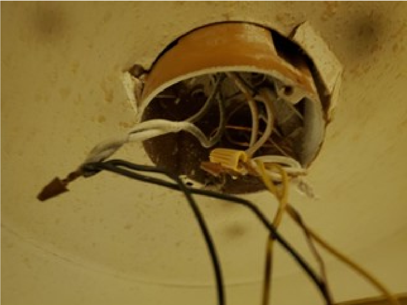
Image #1– Ceiling junction box that supported the light fixture. Shows wire nut melted off, distorted screw hole top left and darkened ceiling.
