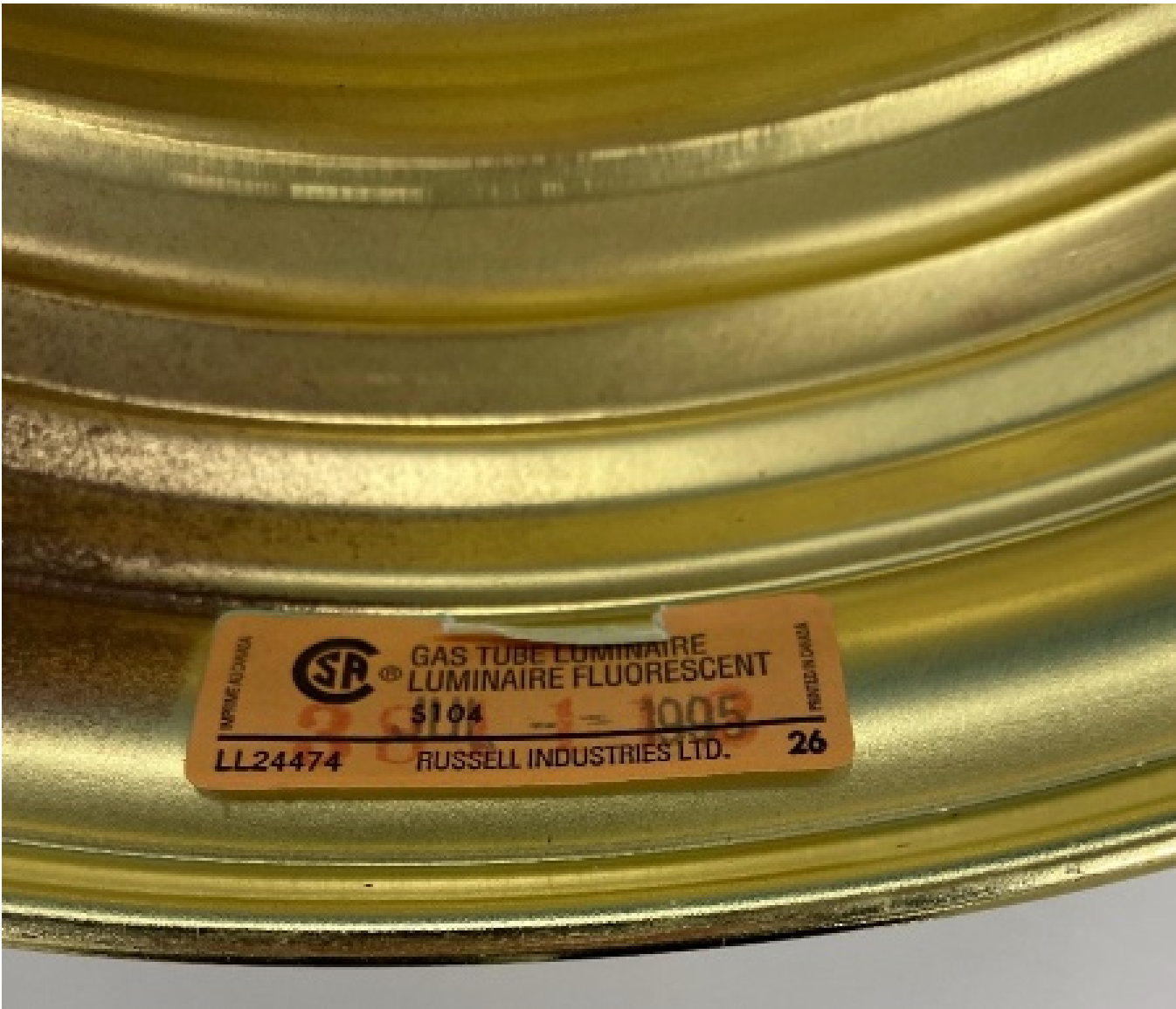
Image 6 - shows fixtures approval label.
