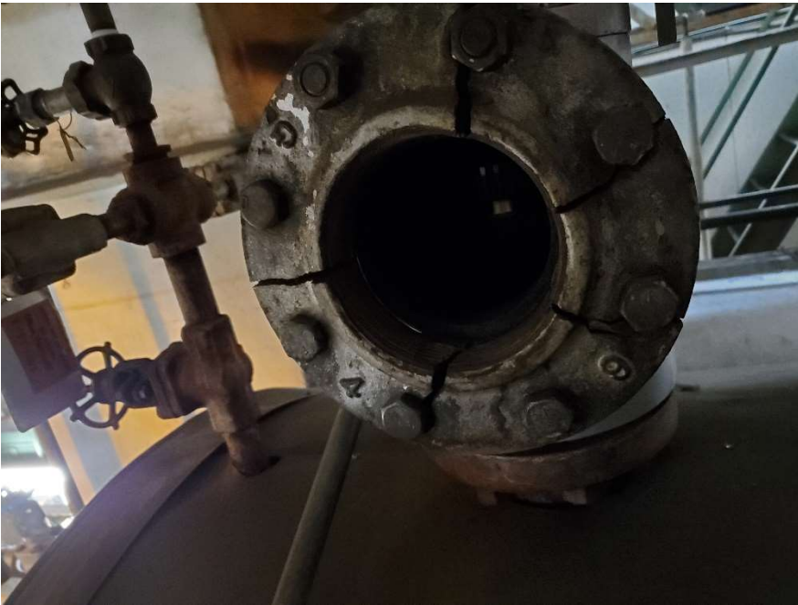
Safety Valve outlet flange showing radial cracking
