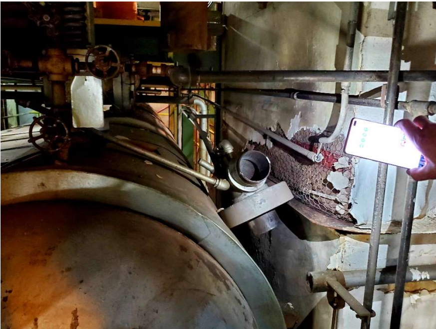
Drip Pan between steam drum and flue-gas uptake ducting
