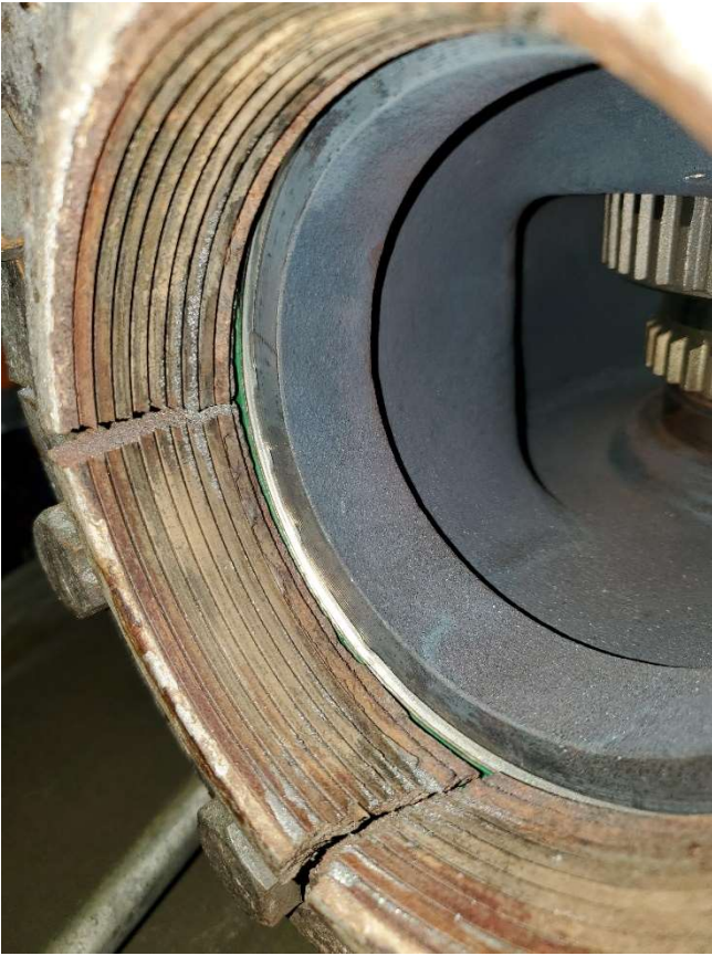
Safety Valve outlet flange showing internal through cracking
