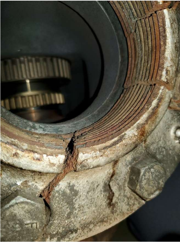
Safety Valve outlet flange cracking
