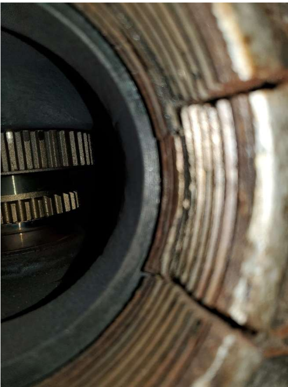
Safety Valve outlet internal cracks
