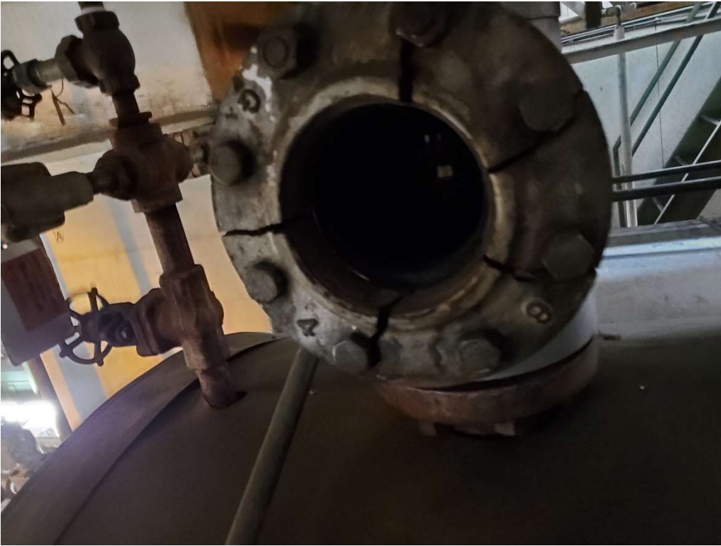
Outlet safety valve flange, still in place, note radial cracking.
