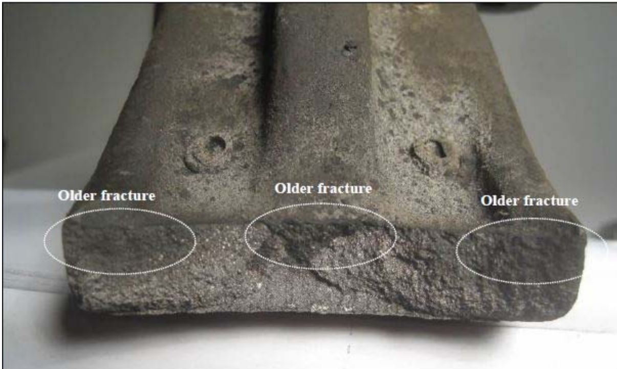
Figure 2 Cross section- darker areas show previous cracking. Photo courtesy of Acuren Group Inc.
